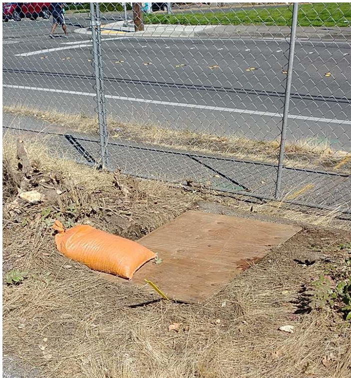
Covered pothole location. Facing East.
