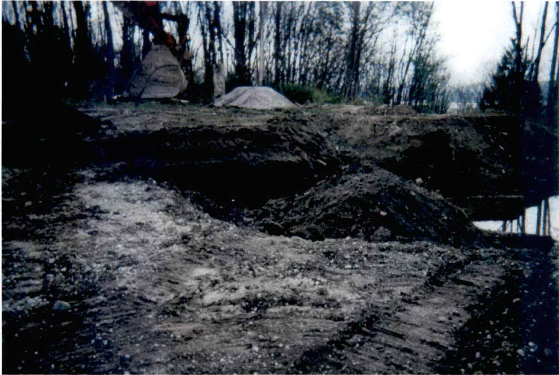
Photograph #7 – View during excavation of battery casing material. Clean soil being stockpiled to use as fill.
