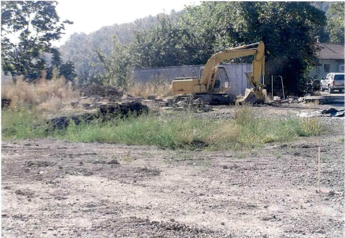
Area south of the excavation (near test pits TP-18, TP-19, and TP-20)
