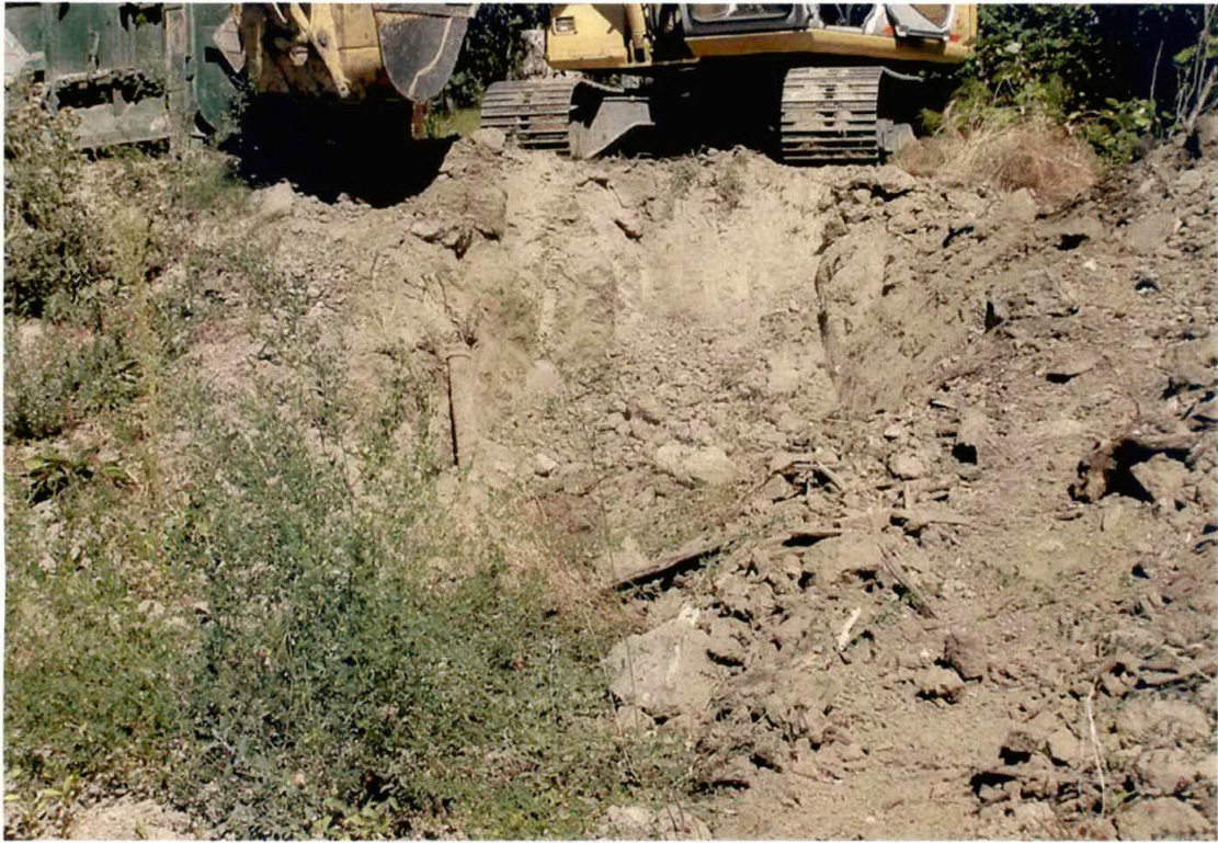
Removal of residual arsenic and lead impacted soil in NE corner of excavation (near TP-22)
