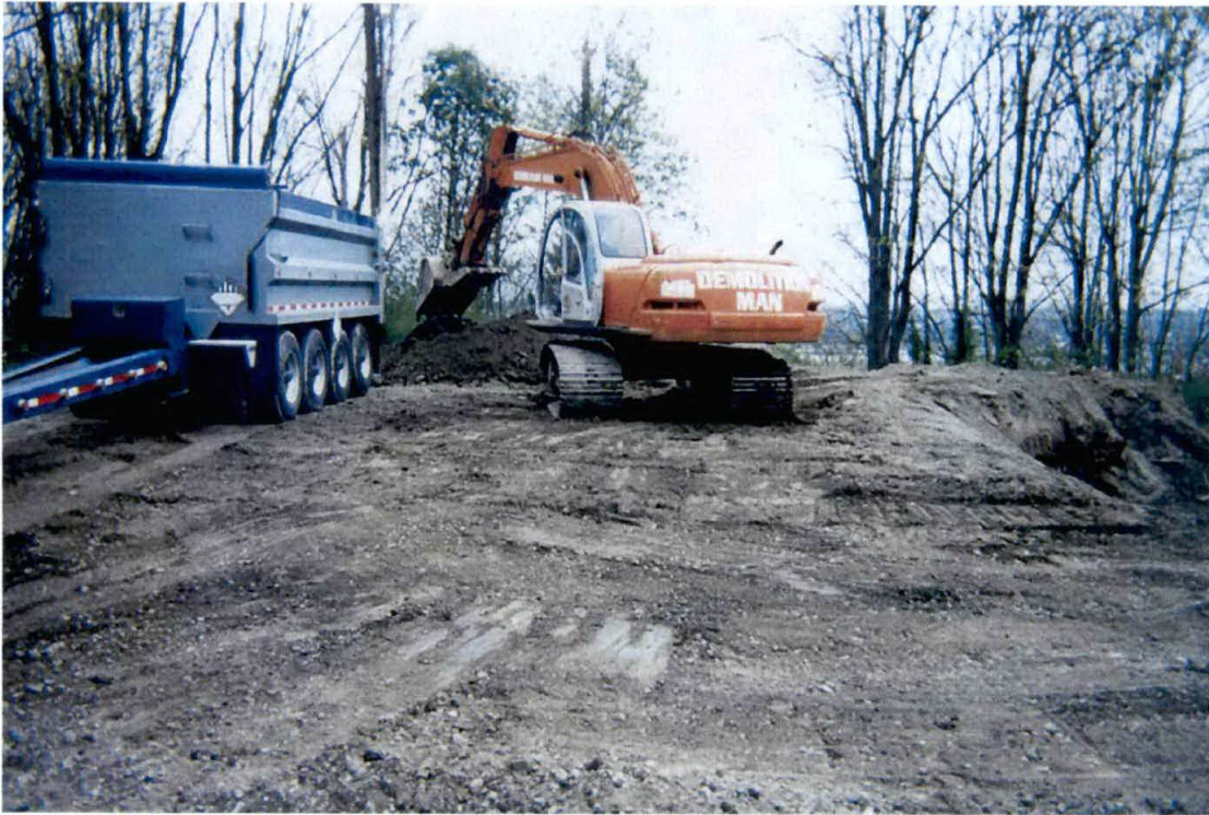
Photograph #15 – Showing removal of battery casing material is close to completed. Excavator is on the final pile of excavated battery casing material that was stockpiled during initial finding of battery casing material.
