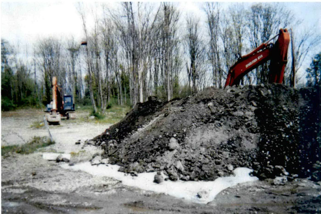
Photograph #12 – View of CKD material pile to be removed from site.
