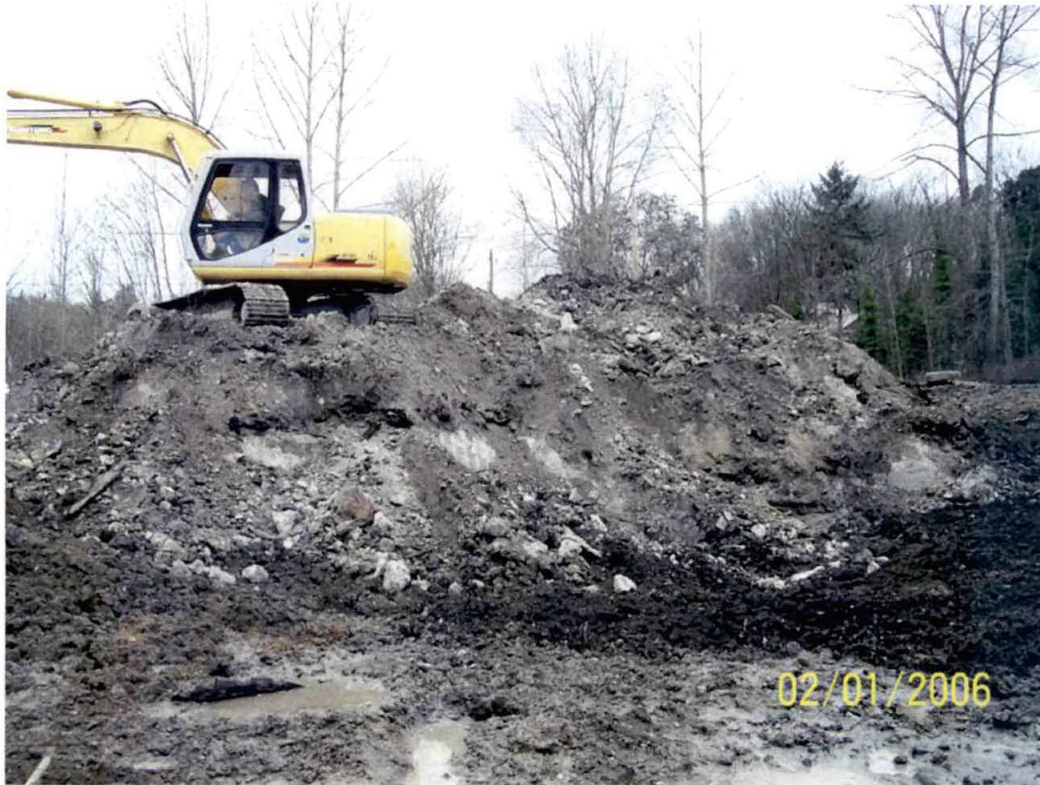
Photograph #15 – View from the east side looking west towards the remaining pile.
