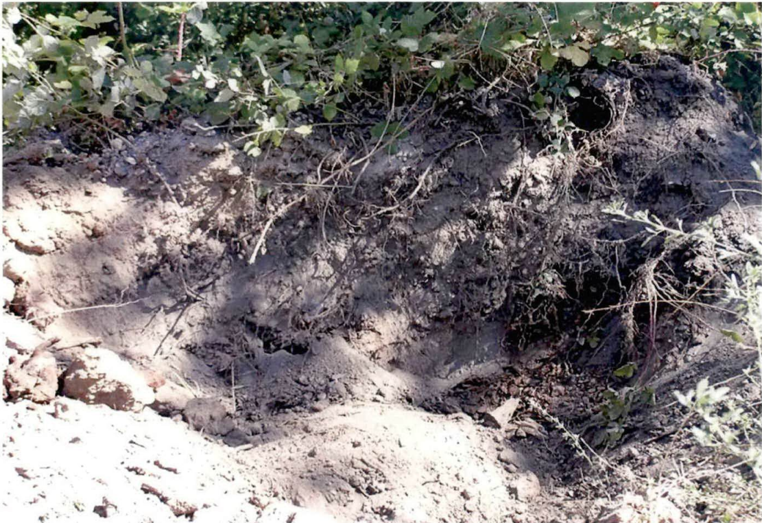
Removal of residual arsenic and lead impacted soil in NE corner of excavation (near TP-21)
