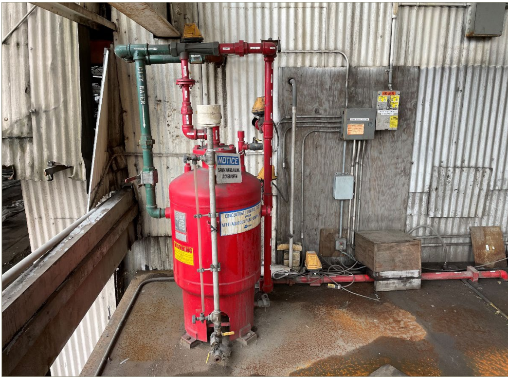
Exhibit 2-5: AFFF Tank and Piping on Roof of the 2,500-Ton Press Pump Room (January 2022)
