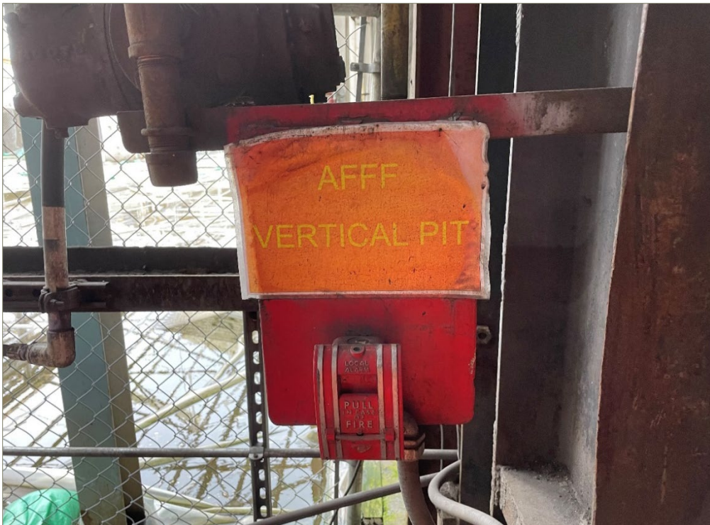
Exhibit 2-6: AFFF Placard on Wall Adjacent to Q1/Q2/Q3 Vault (January 2022)
