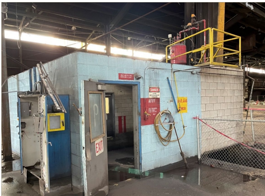
Exhibit 2-1: AFFF System at the 660-Ton Press Pump Room (November 2021)
