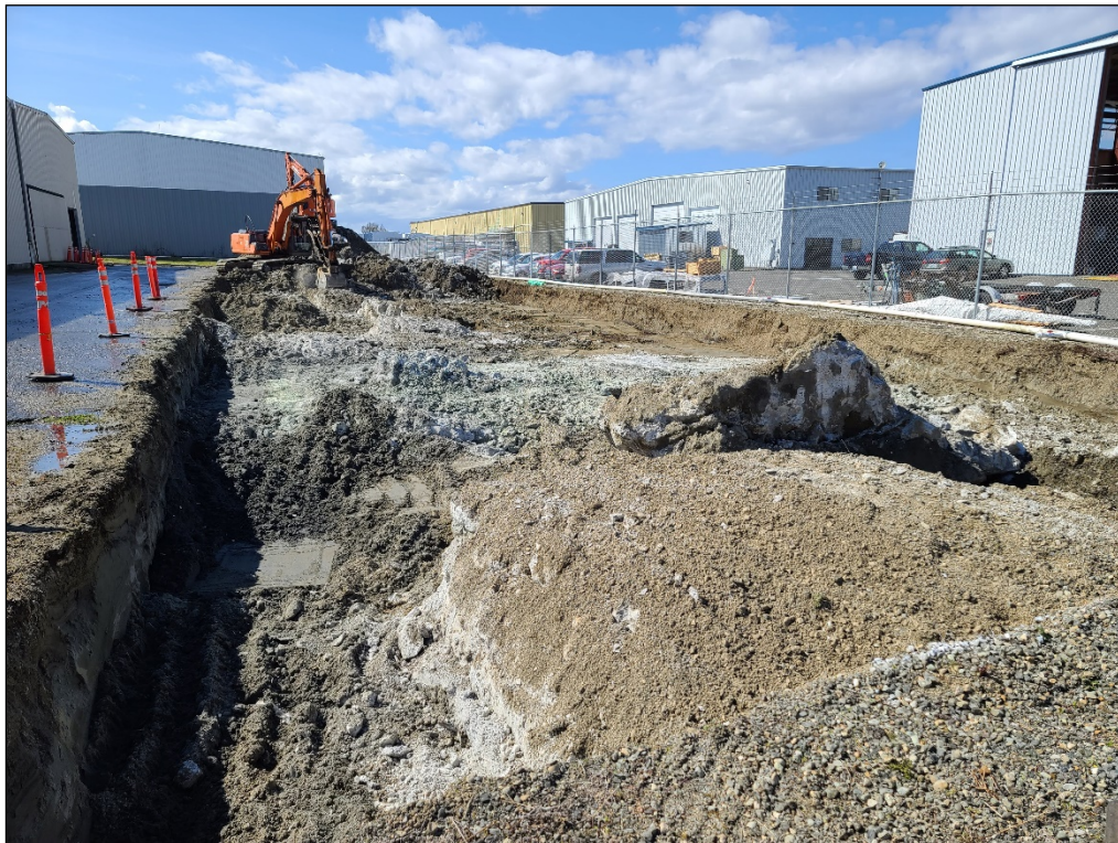
2. Looking west from area H with concrete material in areas F, G, and H.
