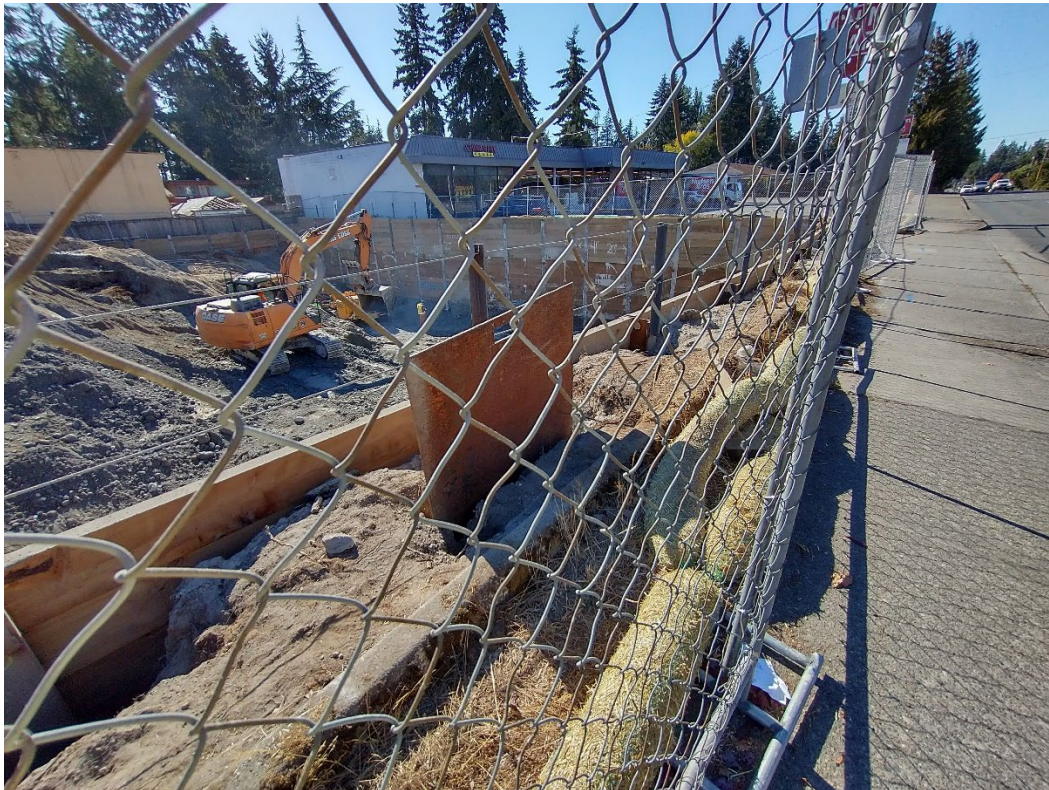
View of north perimeter fence and shoring wall from 196 th St, facing southeast. Shoring wall location set by existing Telecom line behind metal plate.
