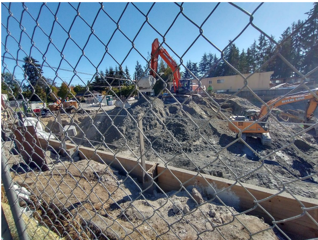
View of excavator for truck loading operations from 196 th St, facing southwest.
