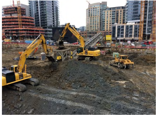
Photo 1: Remedial excavation area, January 25, 2017. Standing near the southeast Property boundary looking northwest across the Property. Excavated fill soil pending transport off-site is shown in center right; excavated native glacial soil is shown in the center.
