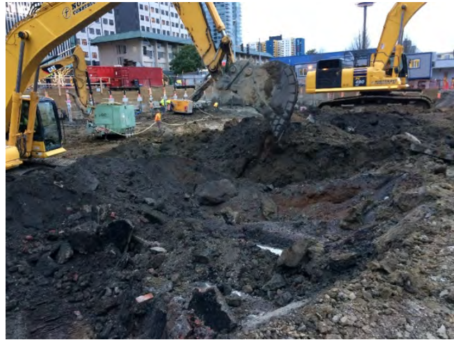
Photo 2: Remedial excavation area, December 15, 2016. Excavated fill soil, typical at the Property, and pending transport off-site. Fill soil contains significant quantities of debris, including charred wood, brick, and concrete.
