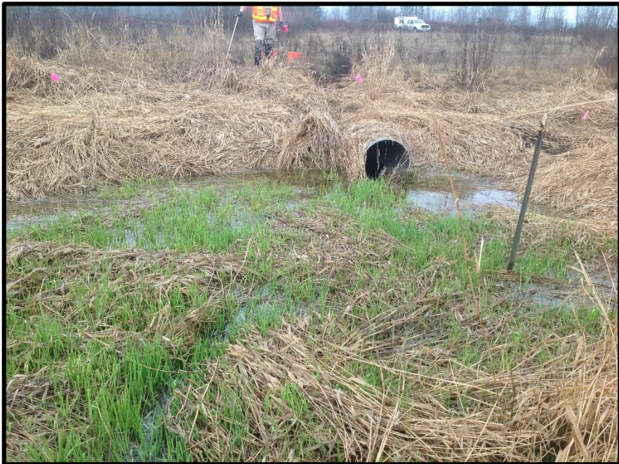
Culvert connecting Wetland A near the rail line to the larger portion of Wetland A.
