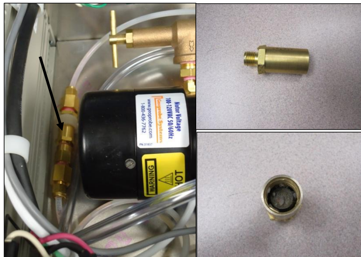
Figure 7.2: Location of Inline Filter in K6300 and buildup of particulates in filter.
