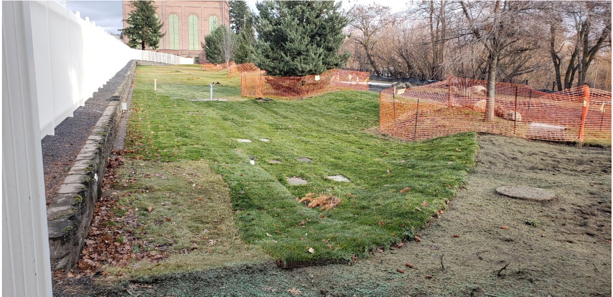
Photograph 3. Photo of the infiltration basin where drained water from the cap discharges (Inspection Area 3), looking north.
