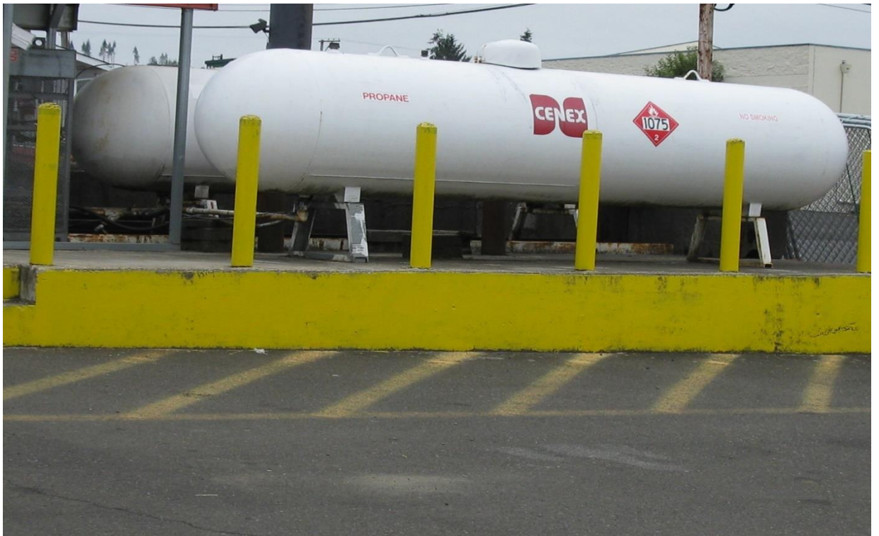
Photo 4: Propane above ground storage tanks – from the Southeast.
