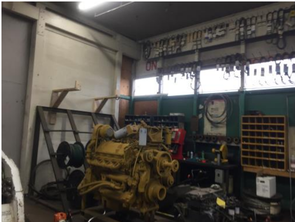
Photo 12 Inside of the vehicle maintenance building
