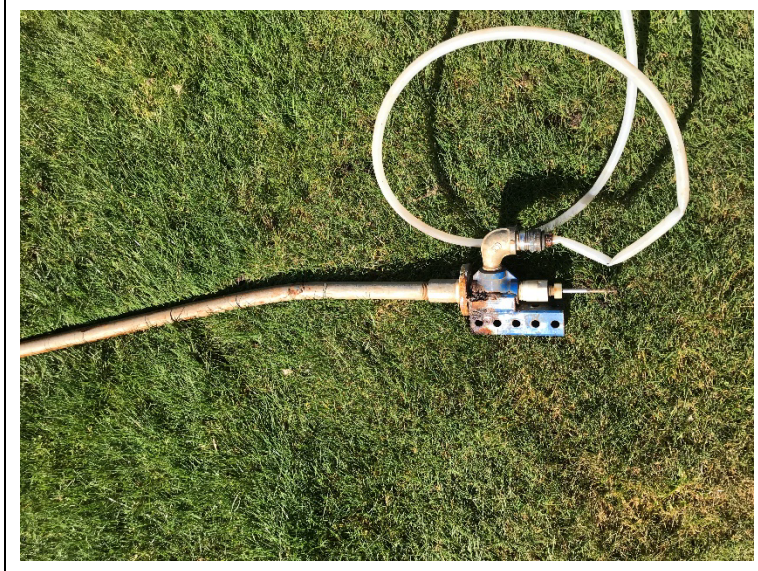
The landing plate and upper portion of the well MW-2 Hydrostar pump discharge pipe showing the degree of bend.
