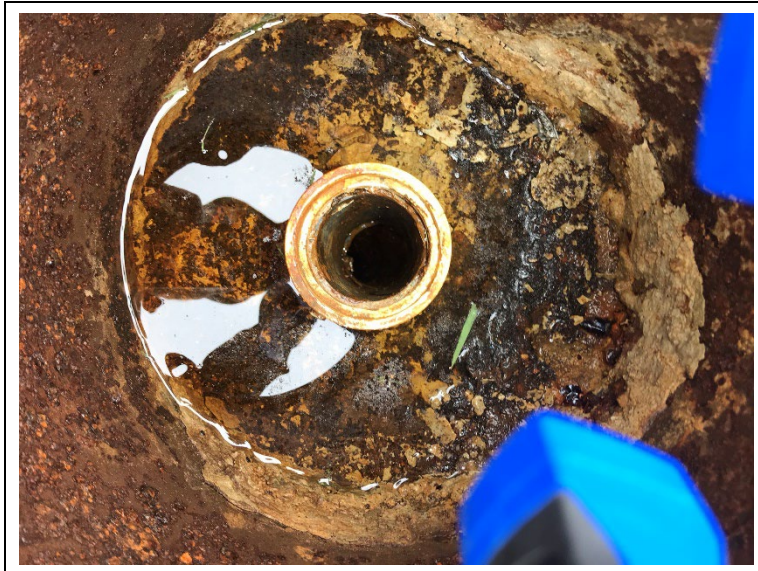
Photograph showing the break in the MW-2 PVC well casing (left center) at the area of the bend in the Hydrostar pump discharge pipe.
