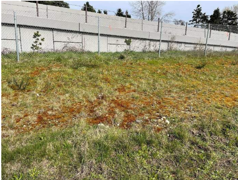
Photograph L2. Stations LLA 05 at the northeast corner of the property with slight loss of vegetation used for erosion control.
