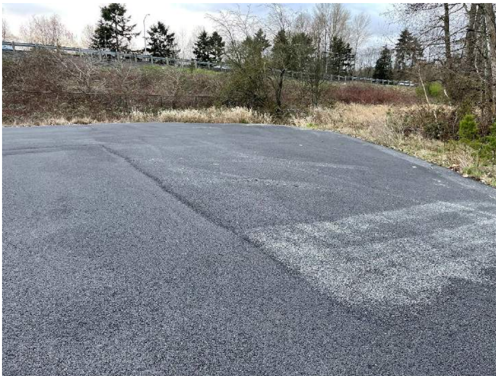
Photograph D2. Good conditions at Station DMCA 04 at the northeast portion of the cap.
