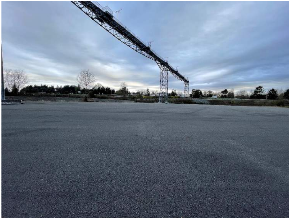
Photograph D6. Generally good cap conditions observed from Station DMCA 08, looking north.
