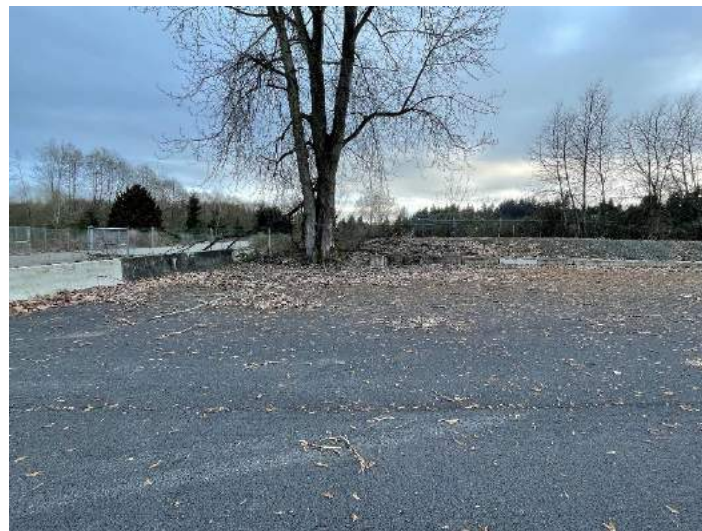
Photograph D4. Substantial organic debris and dust at the southwest corner of the cap near Station DMCA 09.
