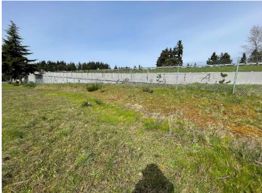
Photograph L1. Station LLA 04 at the northeast corner of the property with slight loss of vegetation used for erosion control.
