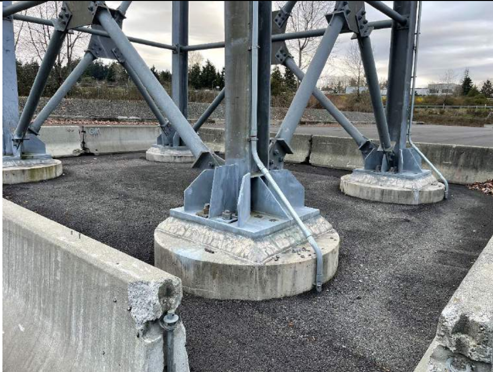
Photograph D5. Good cap conditions around the ecology blocks and structure at DMCA 10.
