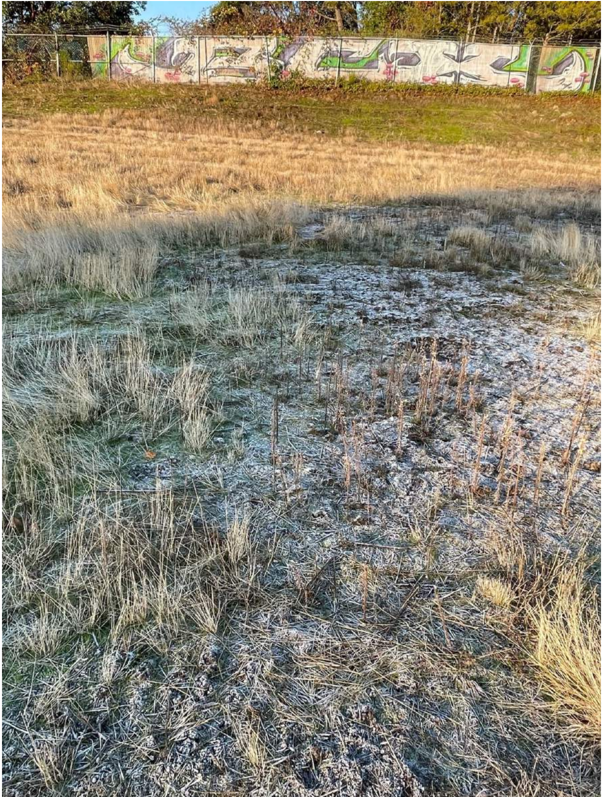
Photograph 5. Natural reseeding at Station LLA 12 and LLA 18 in the area near the swale that was previously noted as requiring maintenance for vegetation loss.
