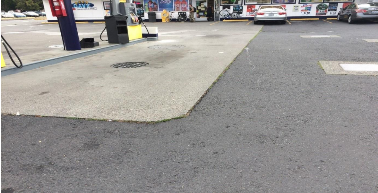
Photo 7: Approximate Area of Soil Contamination Left in Place at 15 feet Below Ground Surface and the Concrete/Asphalt Cap From the North.
