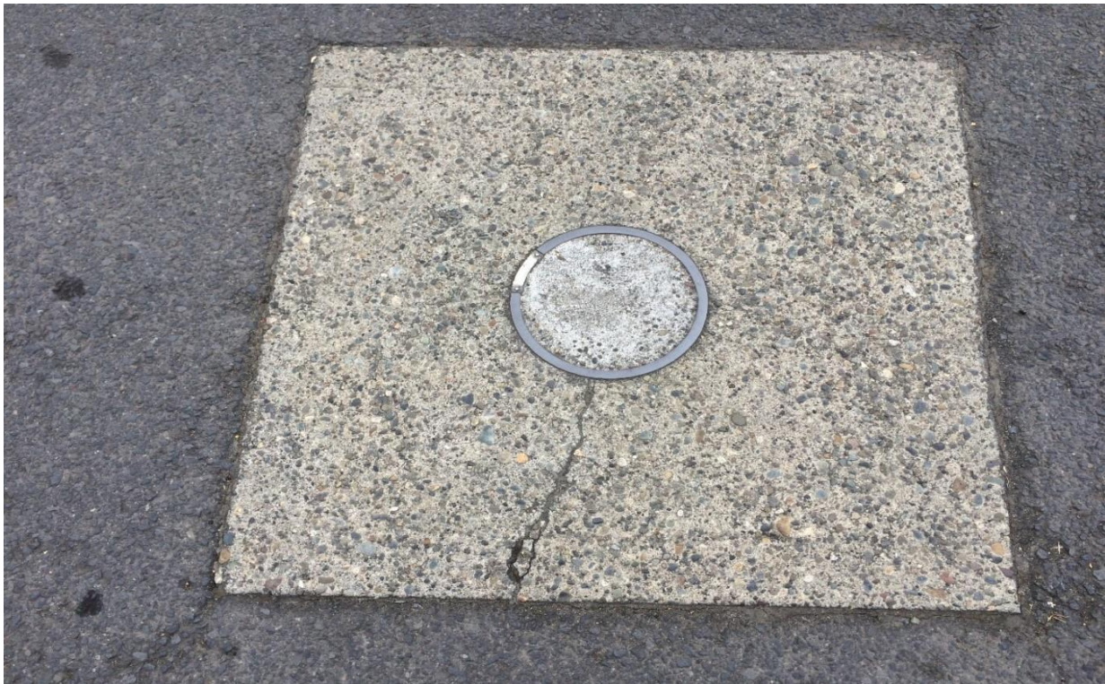
Photo 8: Abandoned Groundwater Monitoring Well.
