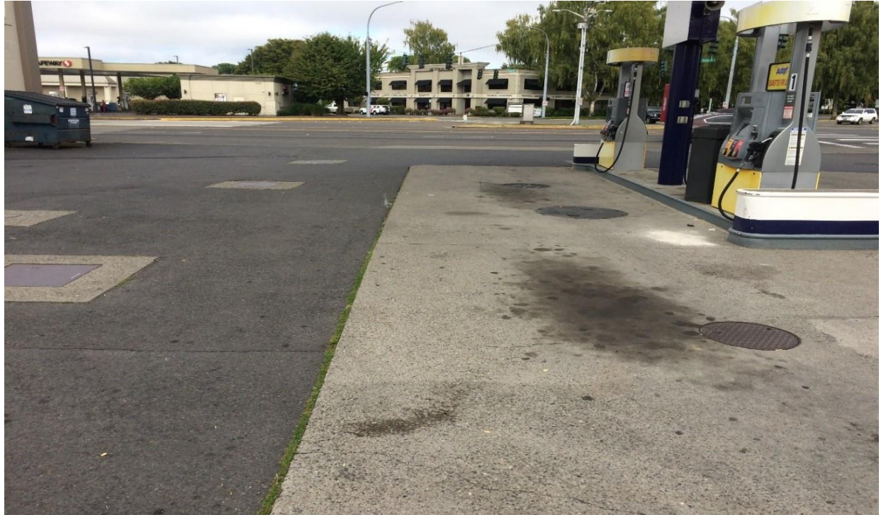
Photo 6: Approximate Area of Soil Contamination Left in Place at 15 Feet Below Ground Surface and the Concrete/Asphalt Cap From the South.
