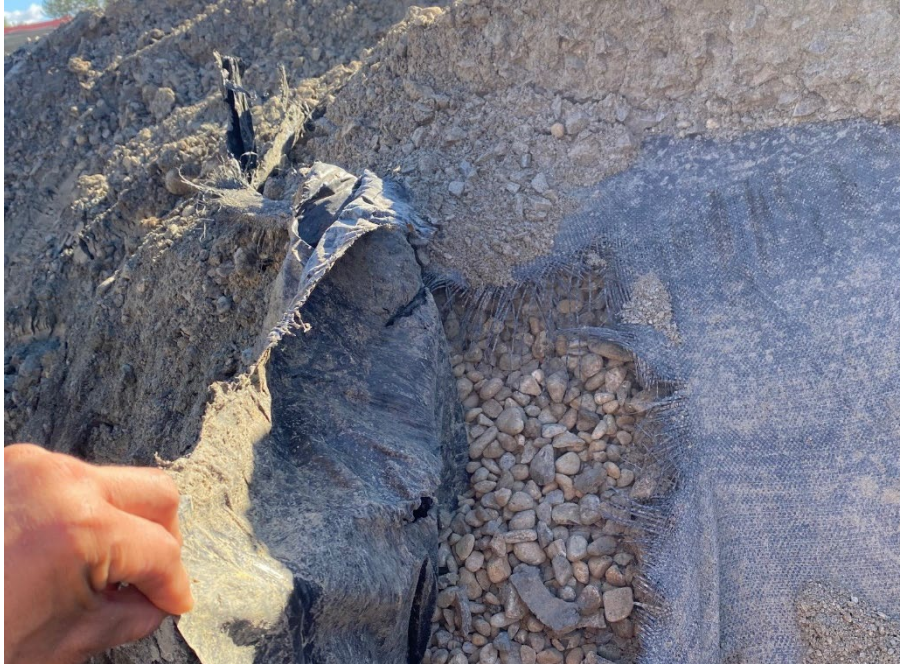
Photograph 37. Toad's Visqueen barrier exposed in upper 1 foot bgs near SIDE-19R to guide overexcavation. View S.
