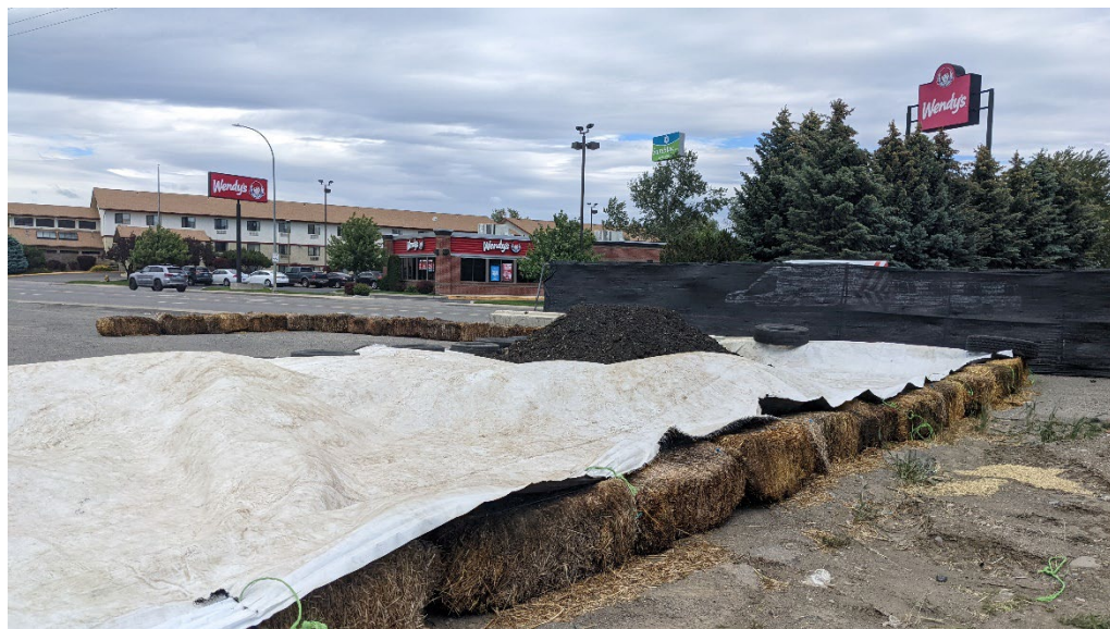
Photograph 26. Impacted soil staging area prior to removal and disposal off-site. View NE.
