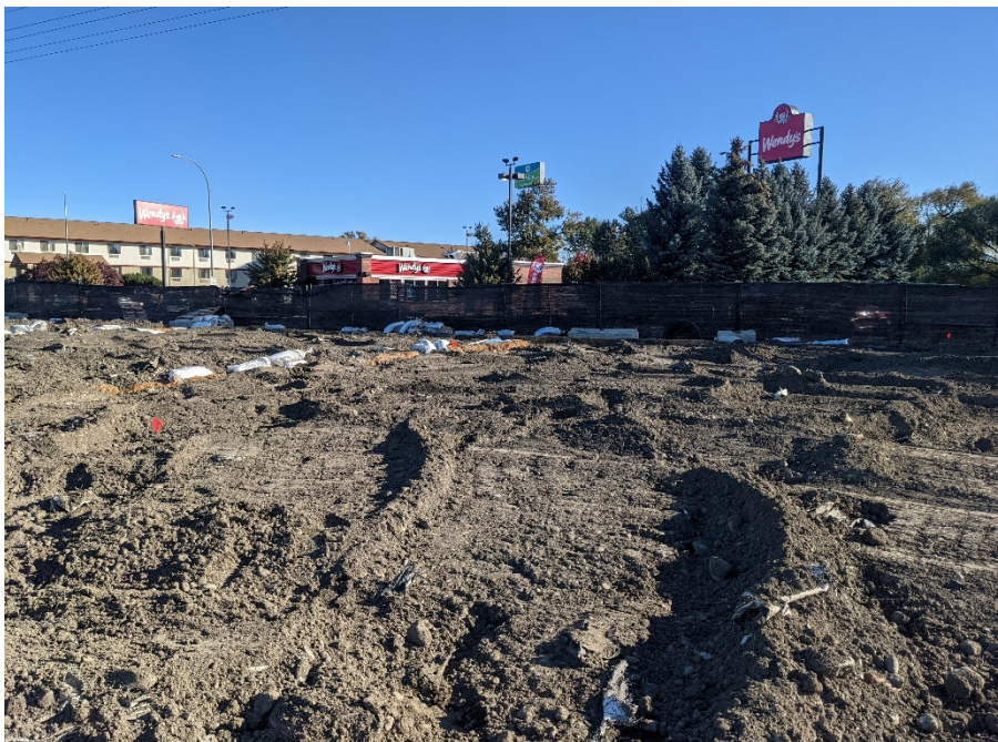
Photograph 18. Overview of DU-03 prior to landfarming confirmation soil sample collection. View NE.
