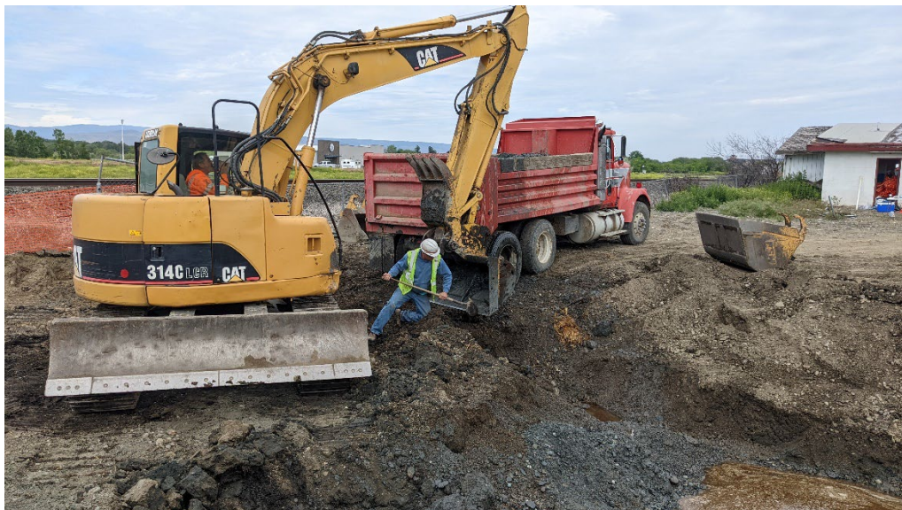
Photograph 24. Cleaning of excavator bucket after removal of LNAPL collection trench, before beginning excavation in SW corner on Toad's property. View NW.
