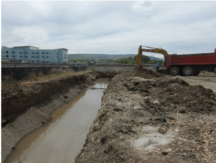
Photograph 3. Exposed pea gravel within light non-aqueous phase liquid (LNAPL) collection trench. View SW.
