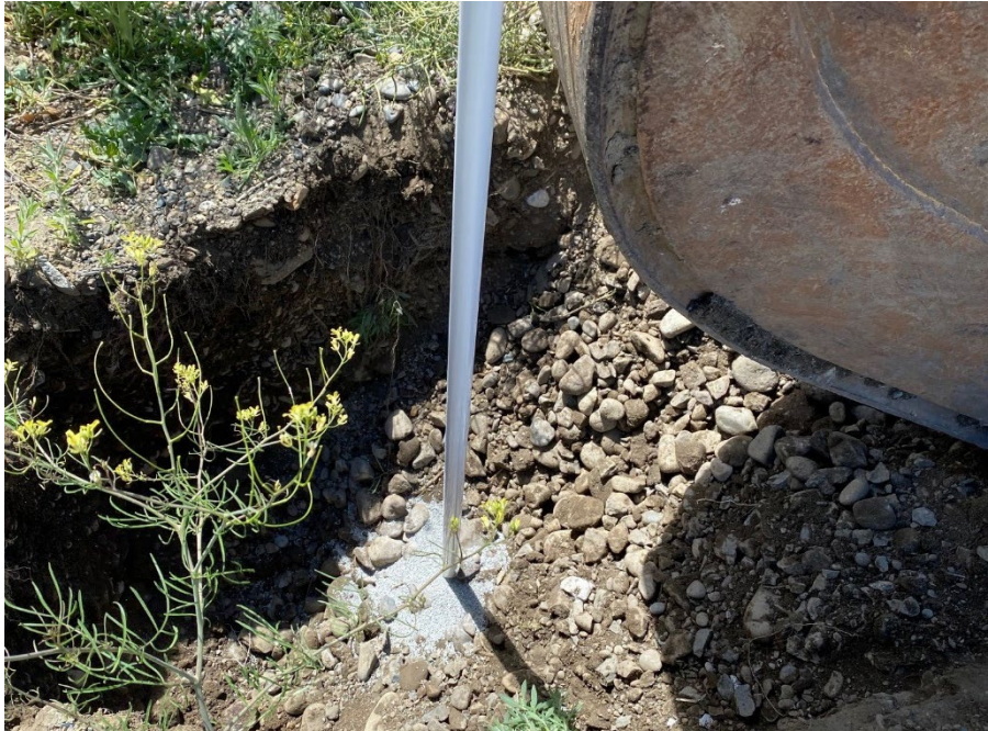
Photograph 55. Installation of bioventing soil vapor monitoring points to 3 feet bgs. Alternating layers of sand and bentonite flakes were poured into the 0.75-inch PVC annular space to prevent short-circuiting.
