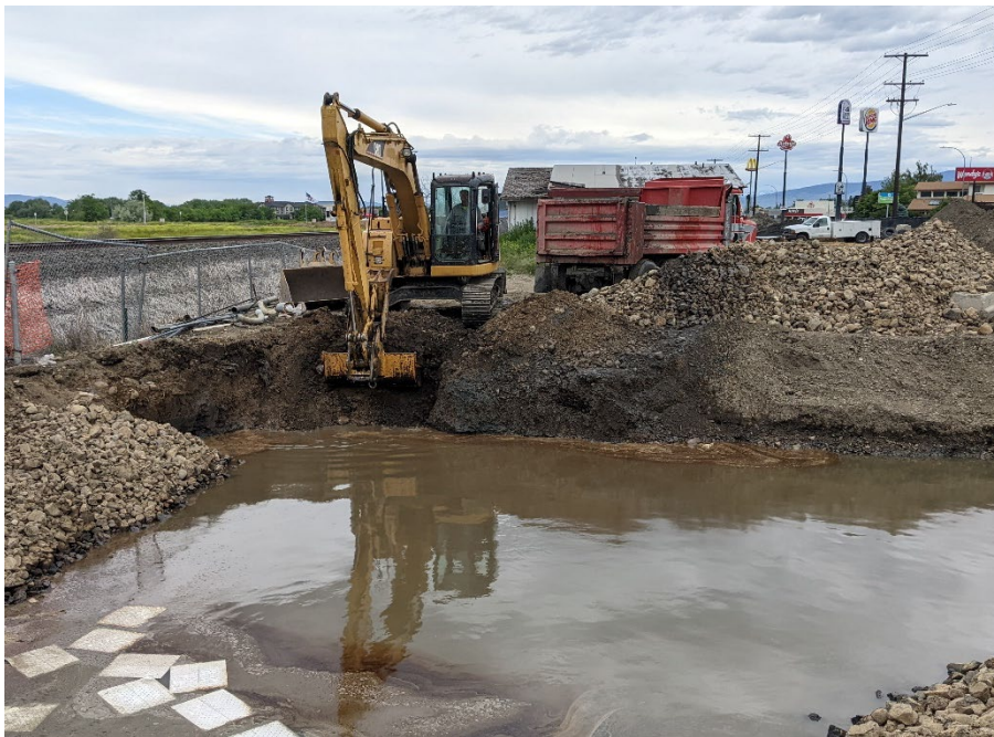
Photograph 34. Excavation of LNAPL collection trench in BNSF ROW. LNAPL visible leaching from pea gravel. View N.
