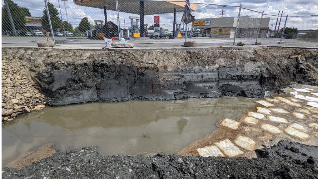
Photograph 29. Excavation extent on Toad's property, view of black silty sand. View S.
