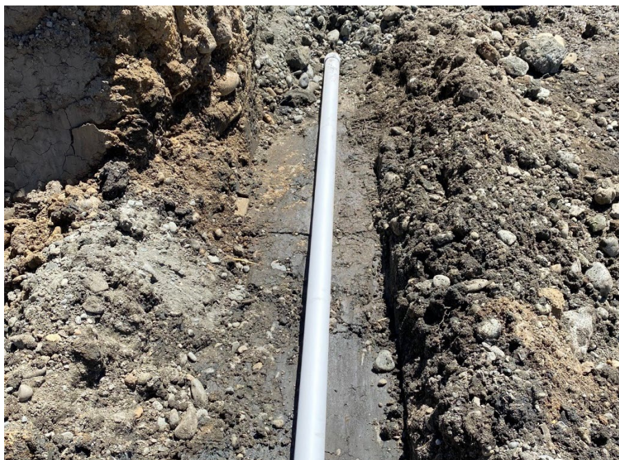
Photograph 42. Installation of easternmost Toad's property bioventing line placed at 3 feet bgs on remaining impacted soil.
