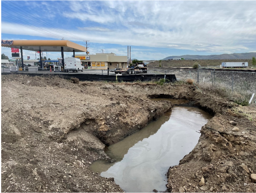
Photograph 5. Southern DRO excavation within BNSF Railway Company (BNSF) right of way (ROW). View SW.
