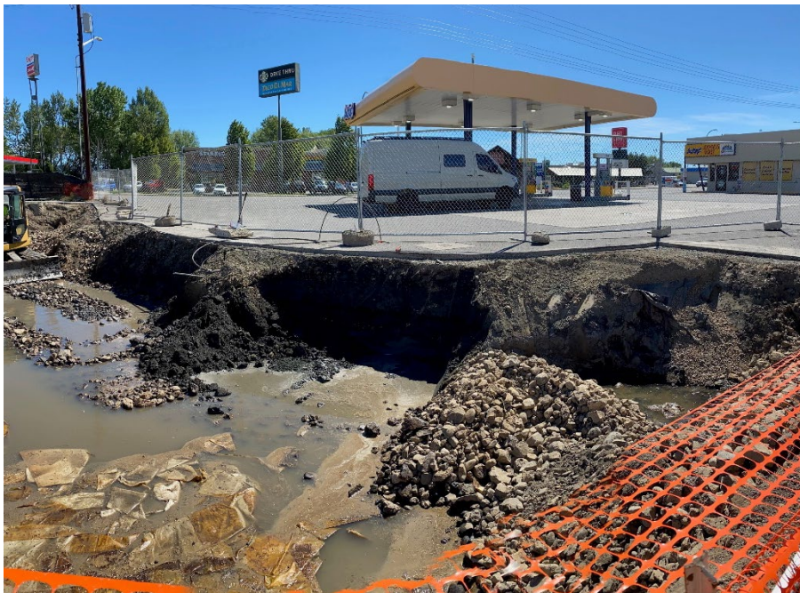
Photograph 38. Toad's Visqueen barrier exposed in upper 1 foot bgs to guide excavation past SIDE-18 and SIDE-19. View SE.
