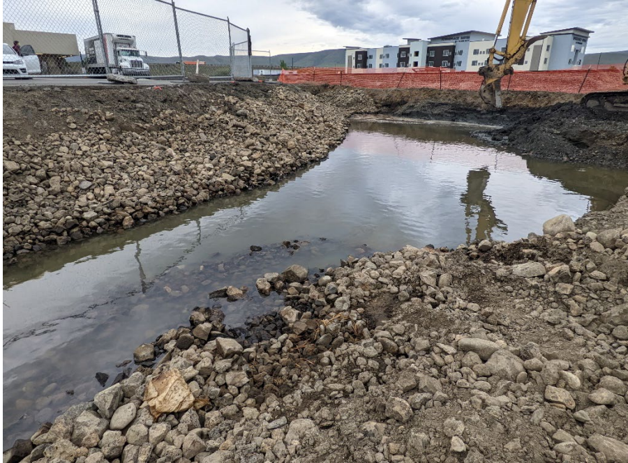
Photograph 33. Excavation and slope shoring. No visible leaching of LNAPL from Toad's or Big B properties. View SW.
