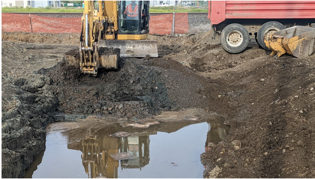
Photograph 23. Excavation on Toad's property and removal of LNAPL collection trench. View W.
