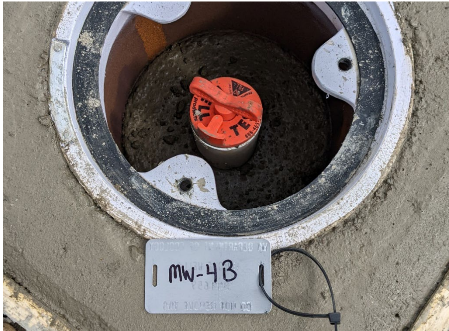
Photograph 51. Monument completion of MW-4B.
