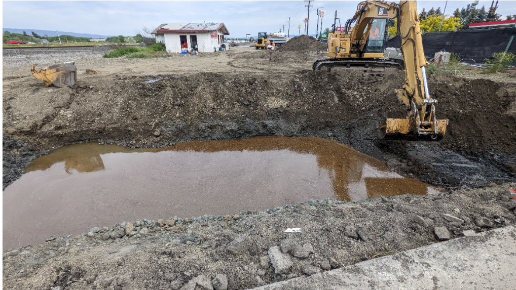
Photograph 27. Excavation to 6.5 feet below ground surface (bgs) above storm sewer, after removal of LNAPL collection trench. View N.
