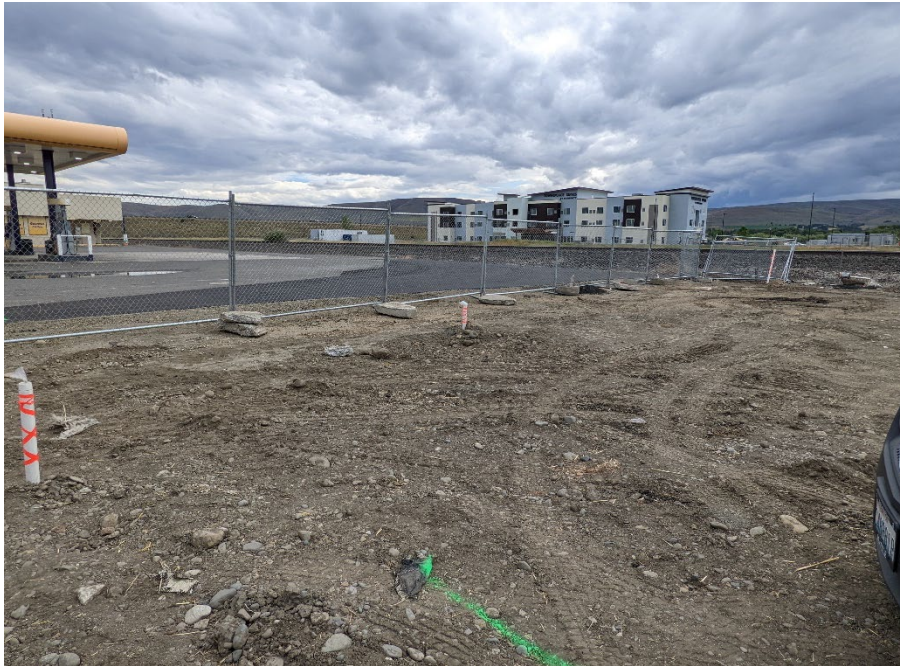
Photograph 47. Aboveground stick-up locations of three Toad’s property bioventing lines, after backfilling. View SW.
