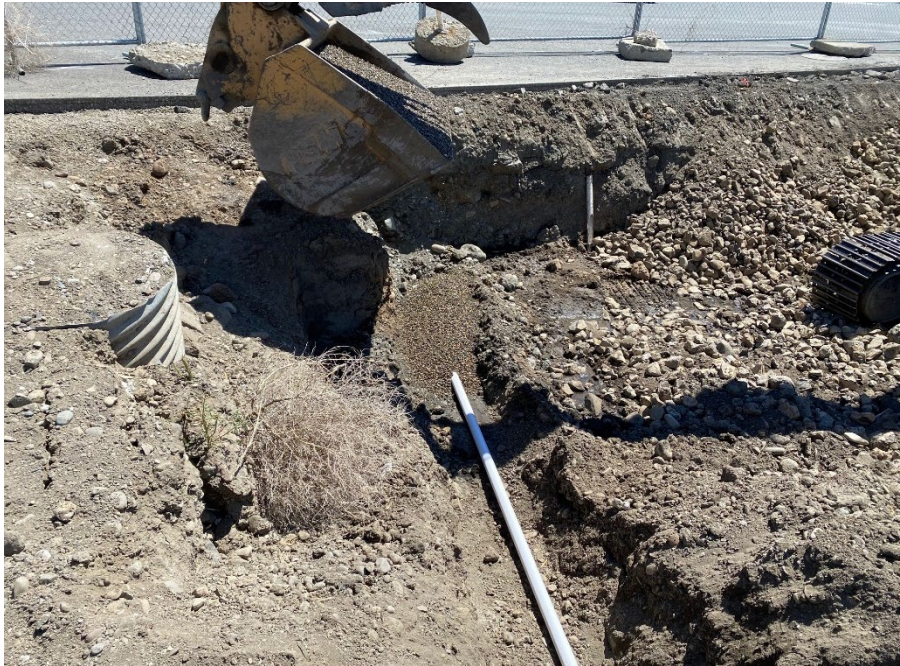
Photograph 43. Installation of easternmost Toad's property bioventing line on impacted soil and placement of pea gravel. View S.
