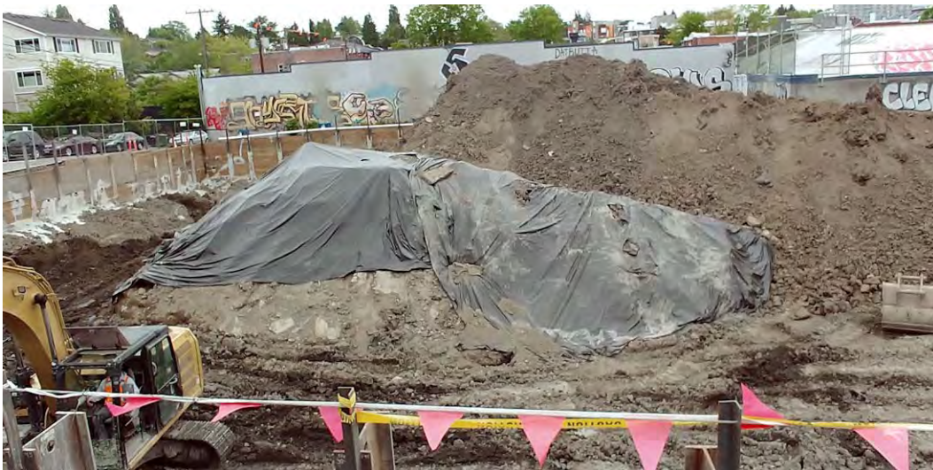
32. View of additional segregated PCS waiting to be loaded and transported off-site for treatment.
