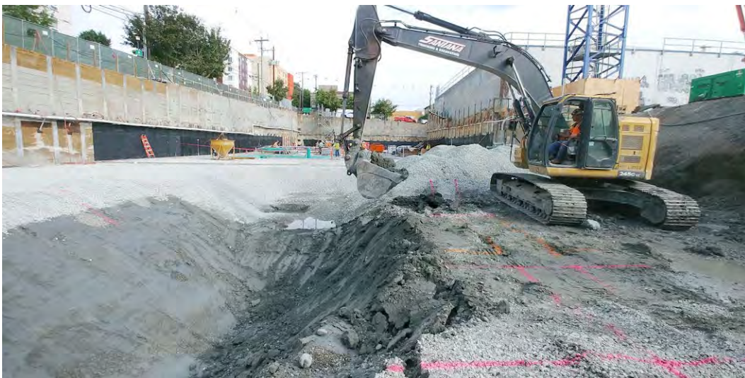
46. View of the elevator pit being dug at the south end of the excavation.
