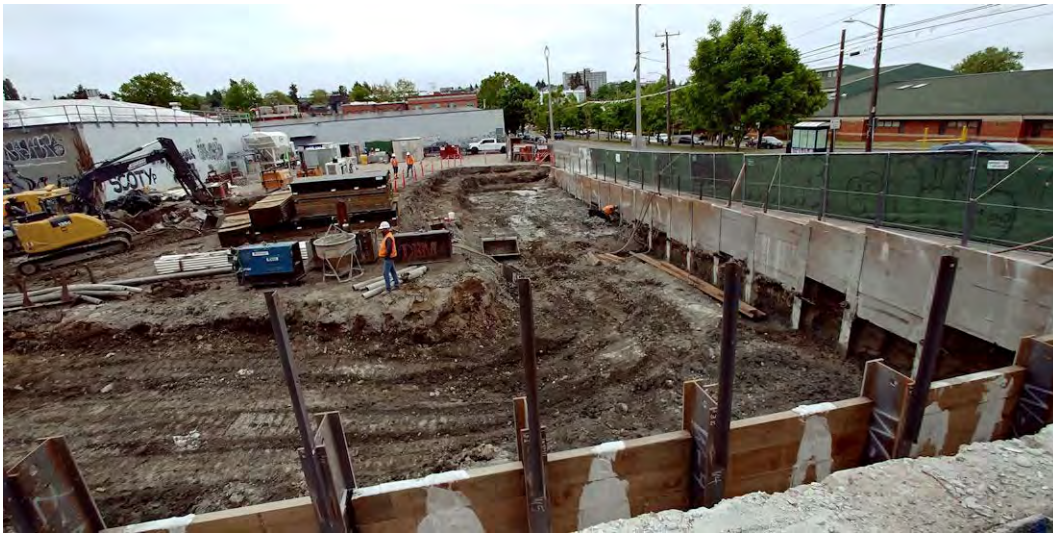
31. View of the south end of the excavation from near the southwestern corner, facing east.
