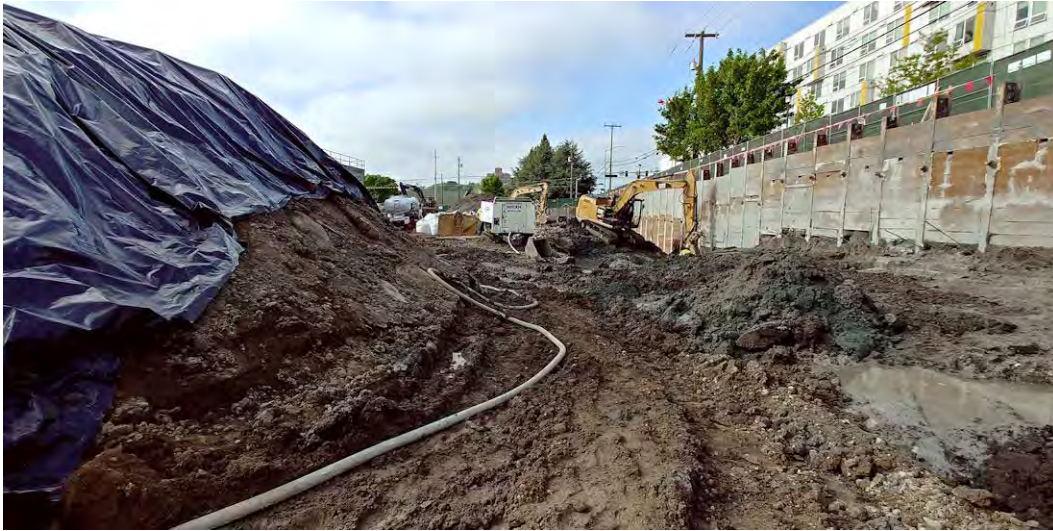
29. View of segregated stockpiles of PCS and the extent of excavation in the northwestern part of the property.
