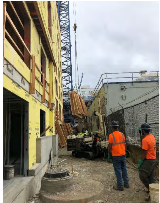
Photo 4: Construction materials being rearranged to allow access for drilling rig. (Northwest View)
