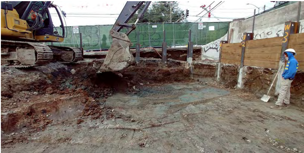
25. View of additional excavation near the former sump in the southwestern part of the site.
