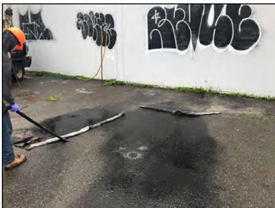
Photo 5: Surfacing from asphalt cracks.
