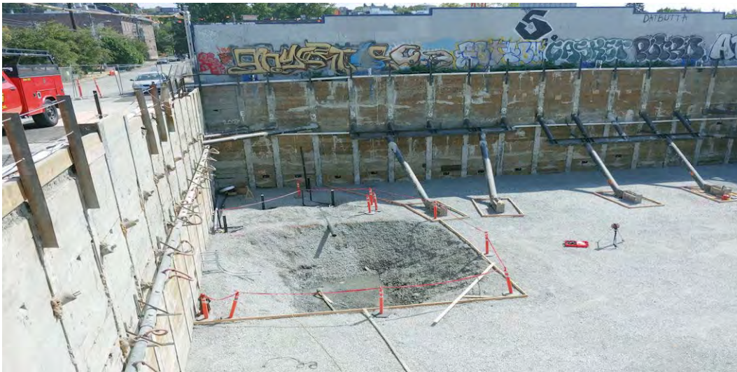
45. View of the north end of the excavation, with elevator pit dug below the main base elevation.
