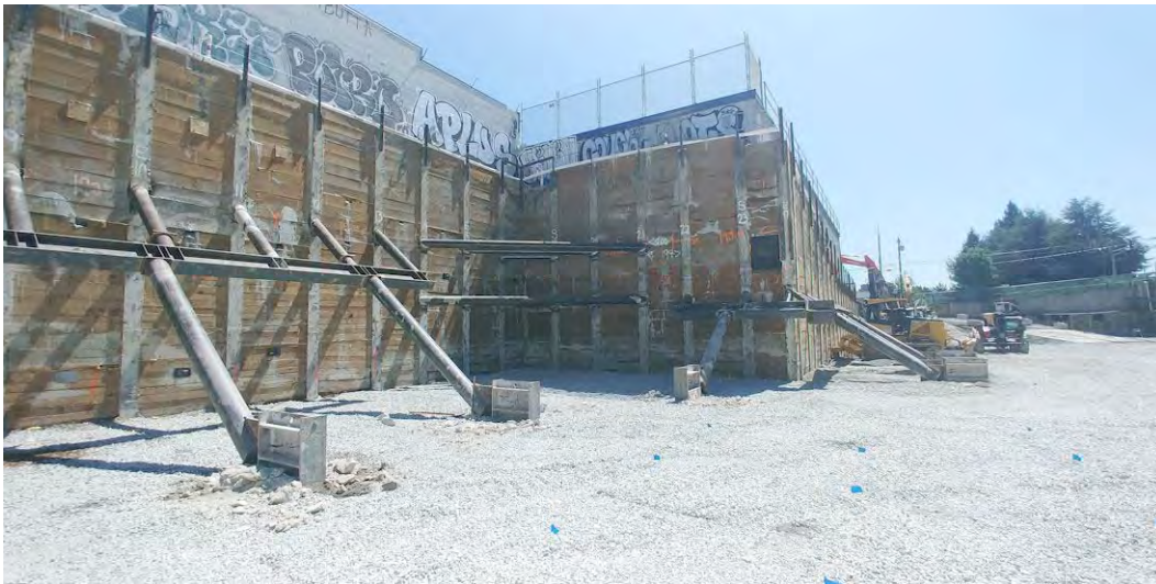
43. View of the main excavation at final depth, with a base layer of gravel installed.
