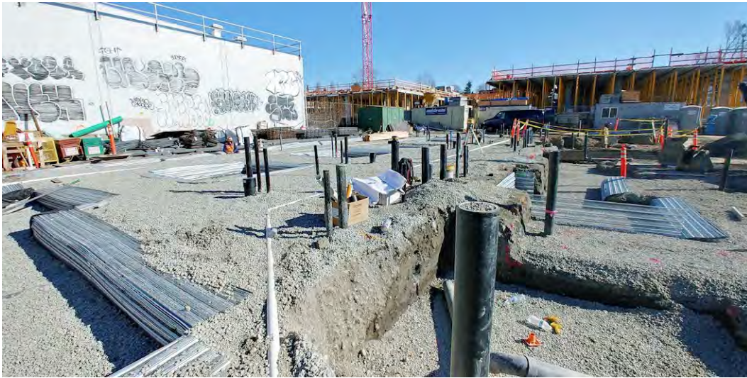
51. View of slab-on-grade foundation excavations and utility piping in the area south of the warehouse.
