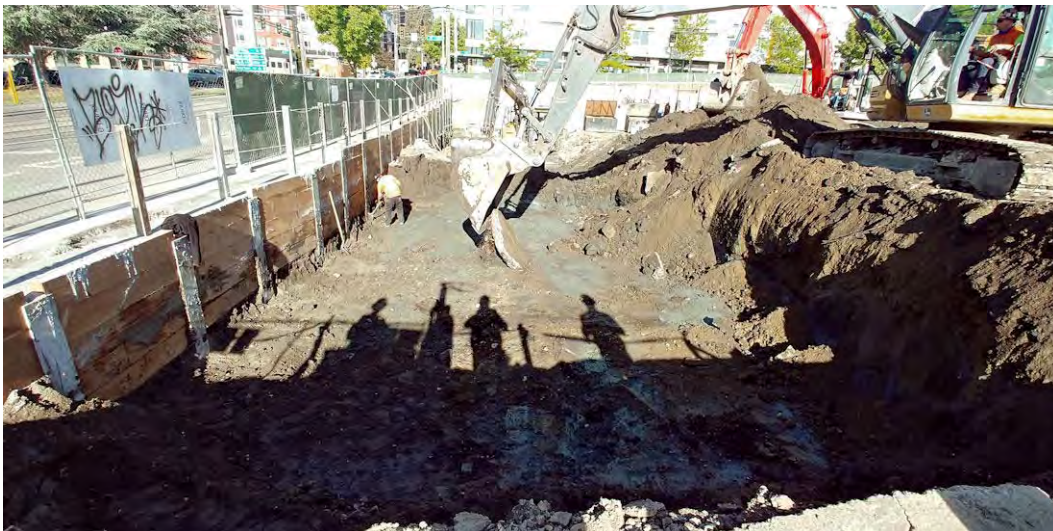
30. View of digging along the south wall of the site, where PCS was encountered, near the former southeastern corner of the 104 12 th Avenue building.
