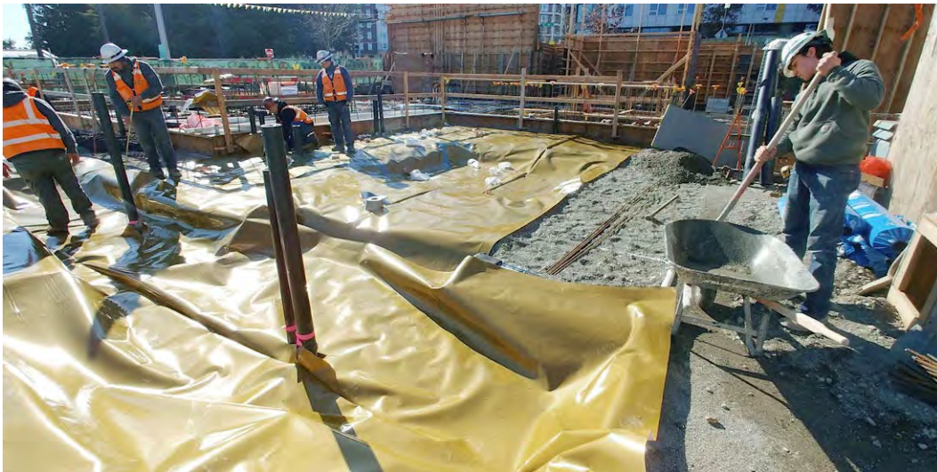
52. View of the installation of a chemical resistant vapor barrier beneath the entire slab-on-grade portion of the building.
