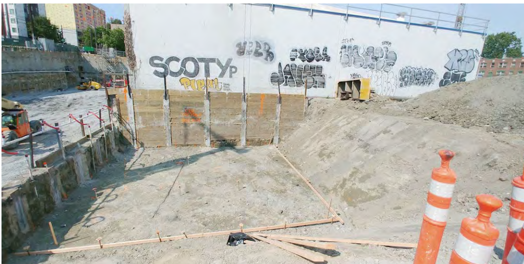
40. View of excavation near the southwestern corner of the King County warehouse for a tower crane foundation.
