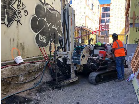
Photo 1: Holocene Drilling using a Geoprobe track mounted rig to advance injection rods. (East View)
