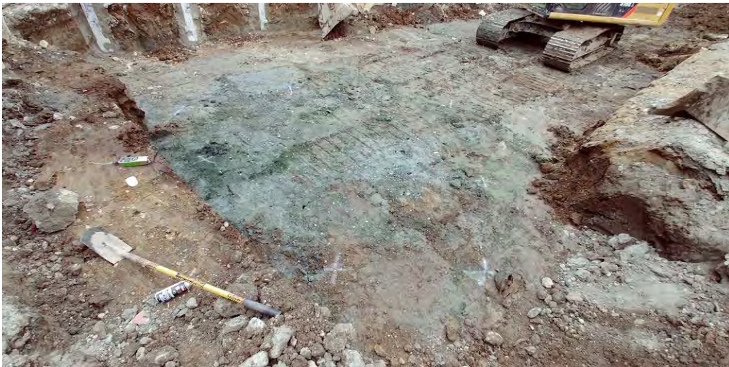
26. View of the discolored soil during field screening of the excavation of the former sump area.
