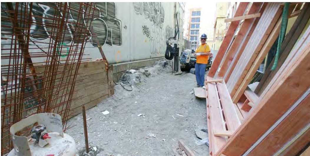
60. View of the driller installing injection points along the north edge of the property adjacent to the warehouse.
