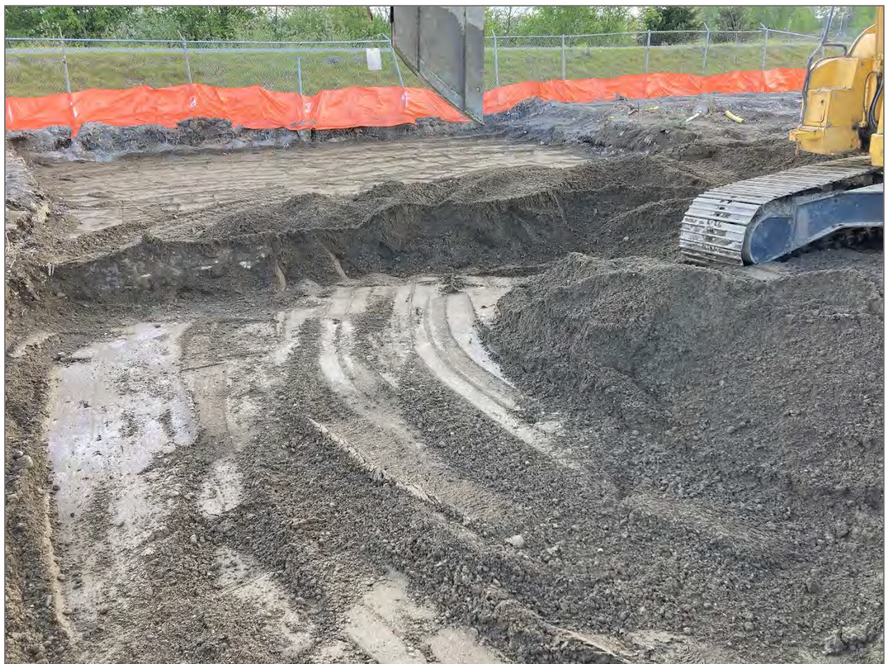
Photo 1: Backfill as observed today in UP-11. Area in the foreground was not compacted. Photo faces east.
