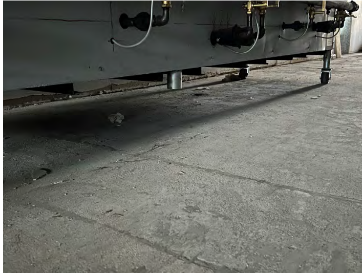
Photograph 17. Floor Slab in Suite B5, Along Shared Wall with Former Harbour Pointe Cleaners (December 19, 2022)
