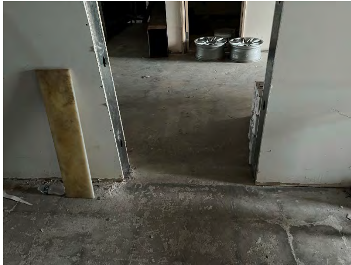
Photograph 16. Floor Slab in Suite B5, Looking into Former Harbour Pointe Cleaners (December 19, 2022)
