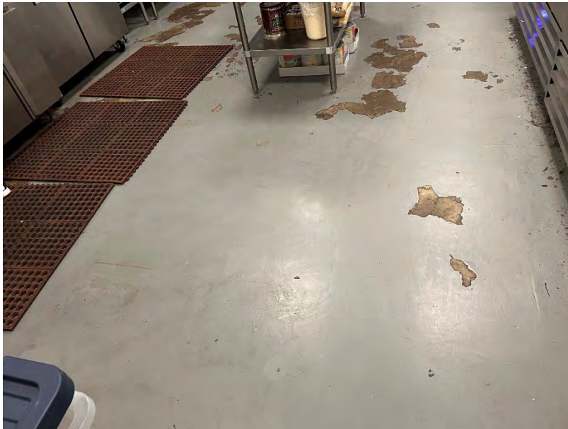
Photograph 12. Floor Slab in Kitchen of Adjacent-West Tenant Space (Suite B7) (December 19, 2022)
