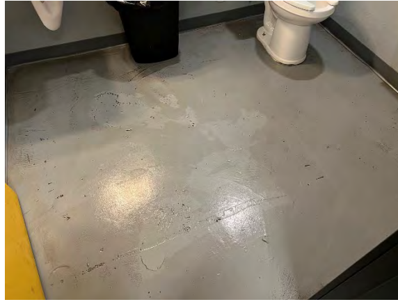
Photograph 15. Floor Slab in Bathroom of Adjacent-West Tenant Space (Suite B7) (December 19, 2022)
