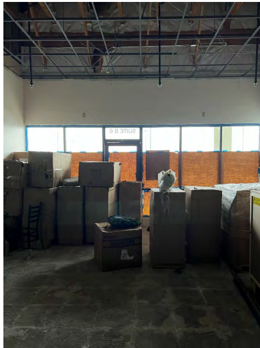
Photograph 4. Floor Slab in Front of Former Harbour Pointe Cleaners (Suite B6) (December 19, 2022)
