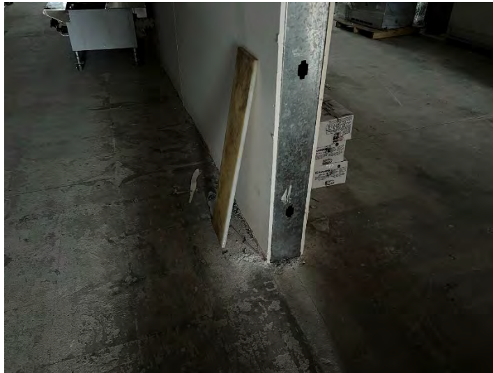
Photograph 18. Floor Slab in Suite B5, Along Shared Wall with Former Harbour Pointe Cleaners (December 19, 2022)
