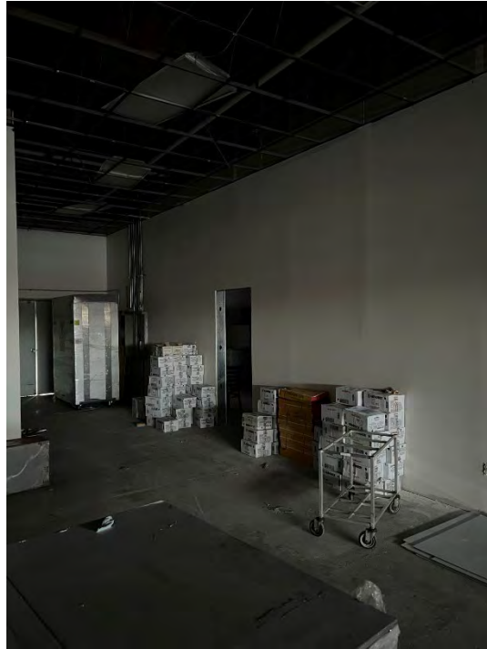
Photograph3. Floor Slab in Rear of Former Harbour Pointe Cleaners, Looking Toward Suite B7 (Suite B6) (December 19, 2022)
