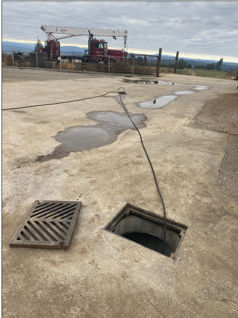
21. 2022: Upland solids staging area, FMF north catch basin sampling location after cleaning, looking south.
