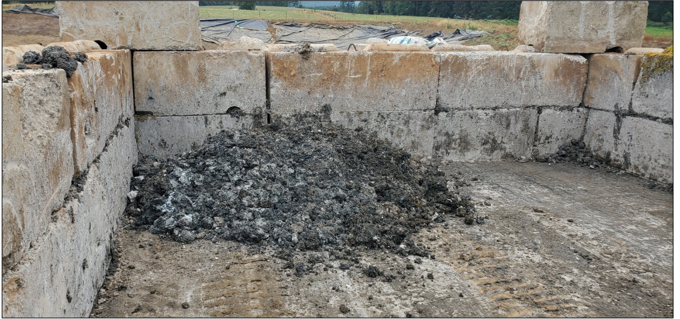
9. 2022: Mixed material temporarily staged on dump slab prior to being loaded onto conveyor.
