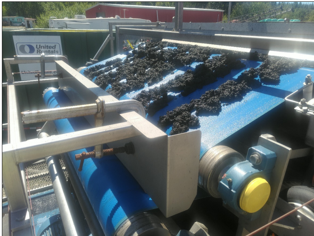
4. 2021: Belt filter press in operation.
