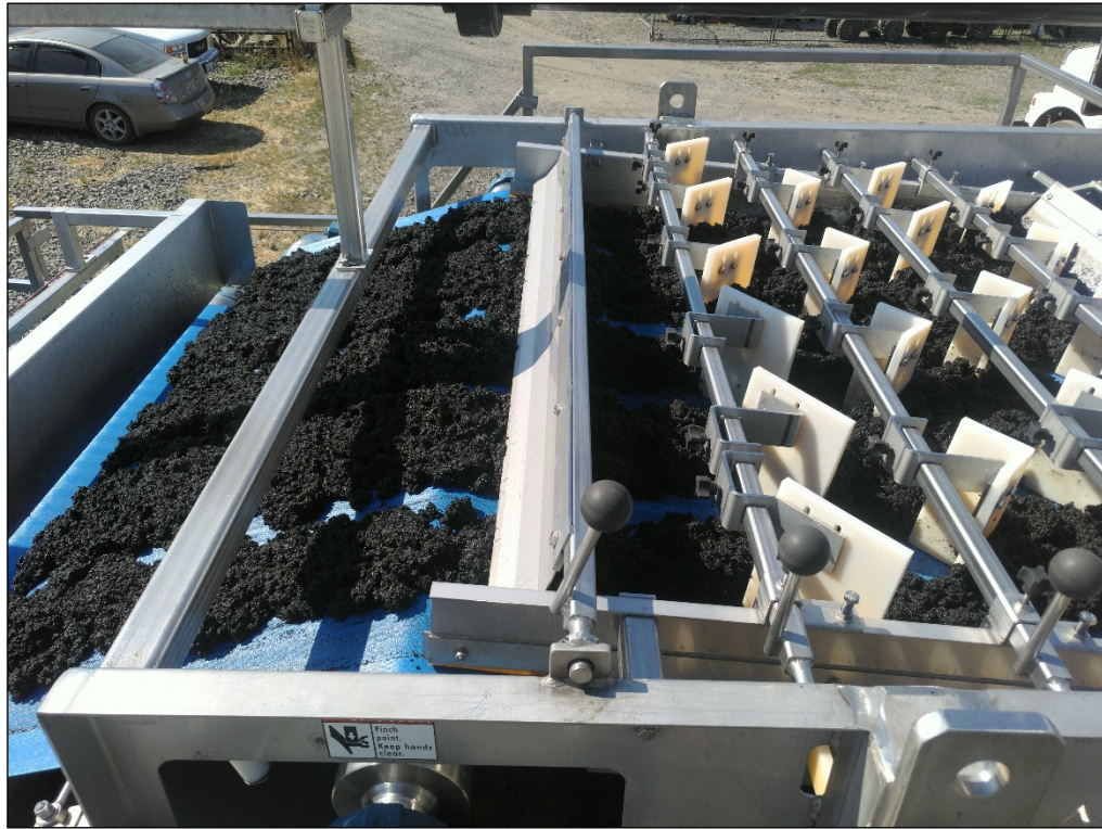
3. 2021: Belt filter press in operation.
