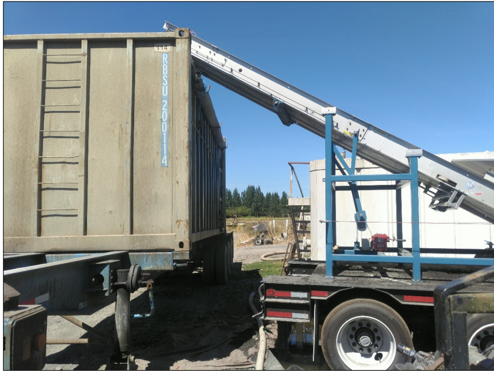
5. 2021: Belt filter press – loading LeMay container.
