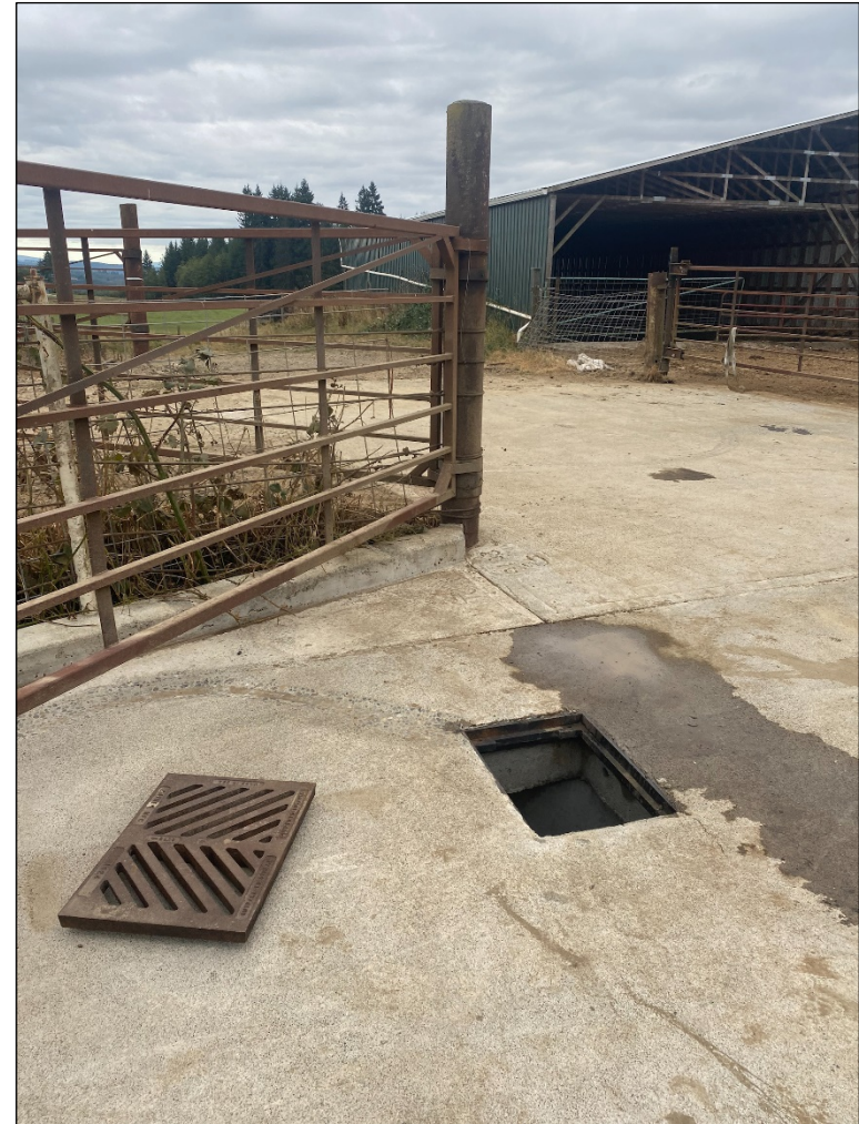
22. 2022: Upland solids staging area, FMF south catch basin sampling location after cleaning, looking west.
