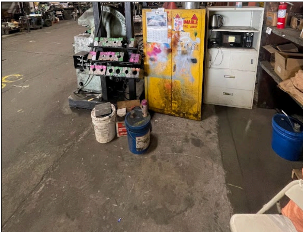
Area 5 containing hazardous materials locker and sealant peeling from seams
