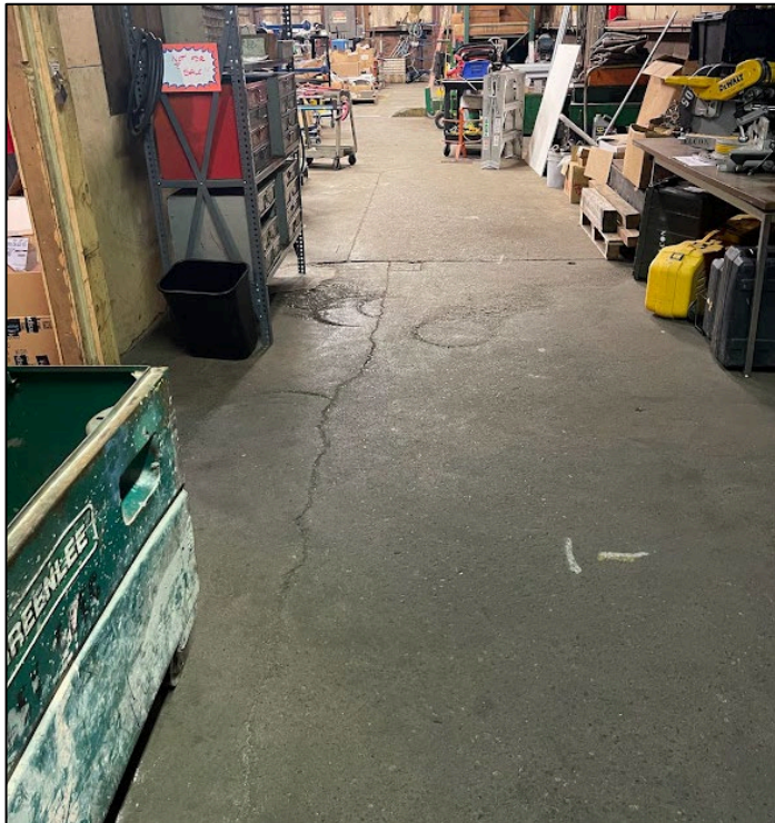
Area 1 (looking north) in the Equipment Repair Shop with unsealed cracks and seams
