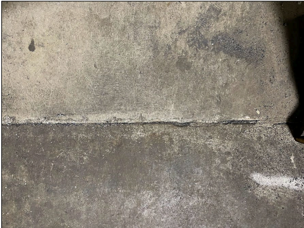
Exposed edge to evaporator pit showing seals covered in metal shavings and no cracks
