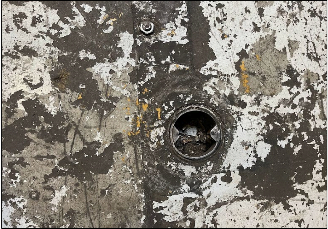
Area 2 unsealed drain and drill holes
