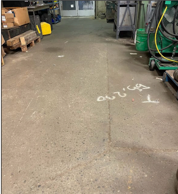
Area 1 (looking south) in the Equipment Repair Shop with unsealed cracks and seams
