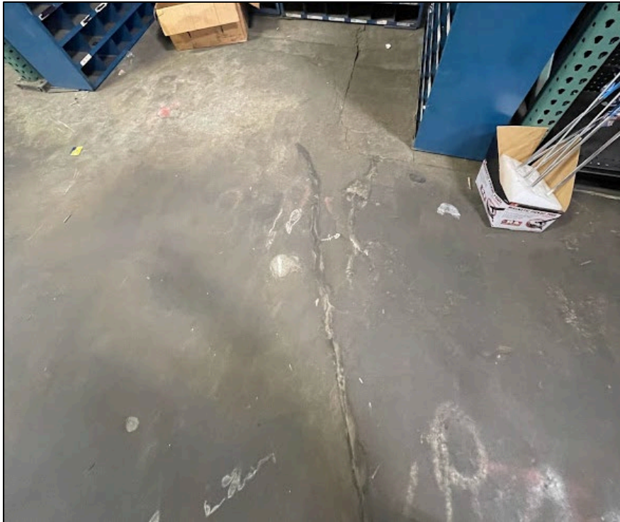
Area 3 unsealed cracks
