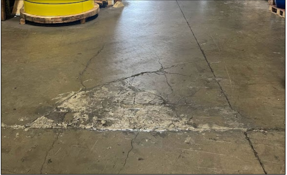
Area 7 showing unsealed cracks and seams
