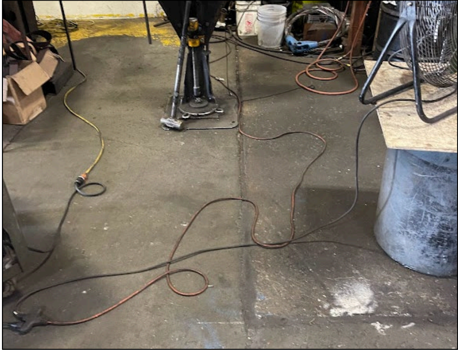
Central warehouse area showing minor sealant wear
