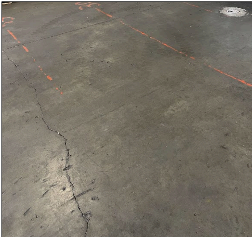
Area 9 showing unsealed cracks
