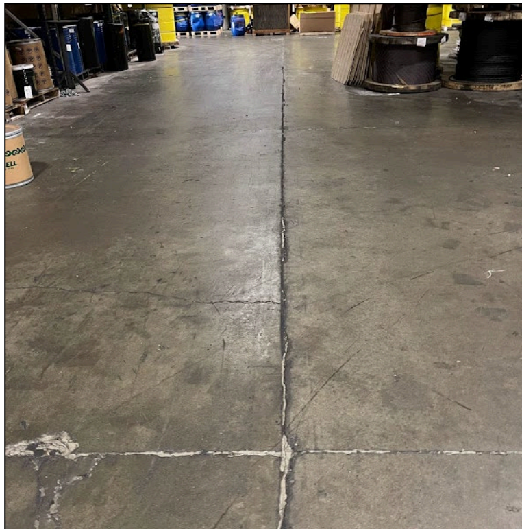
Area 6 showing unsealed cracks and minor sealant wear
