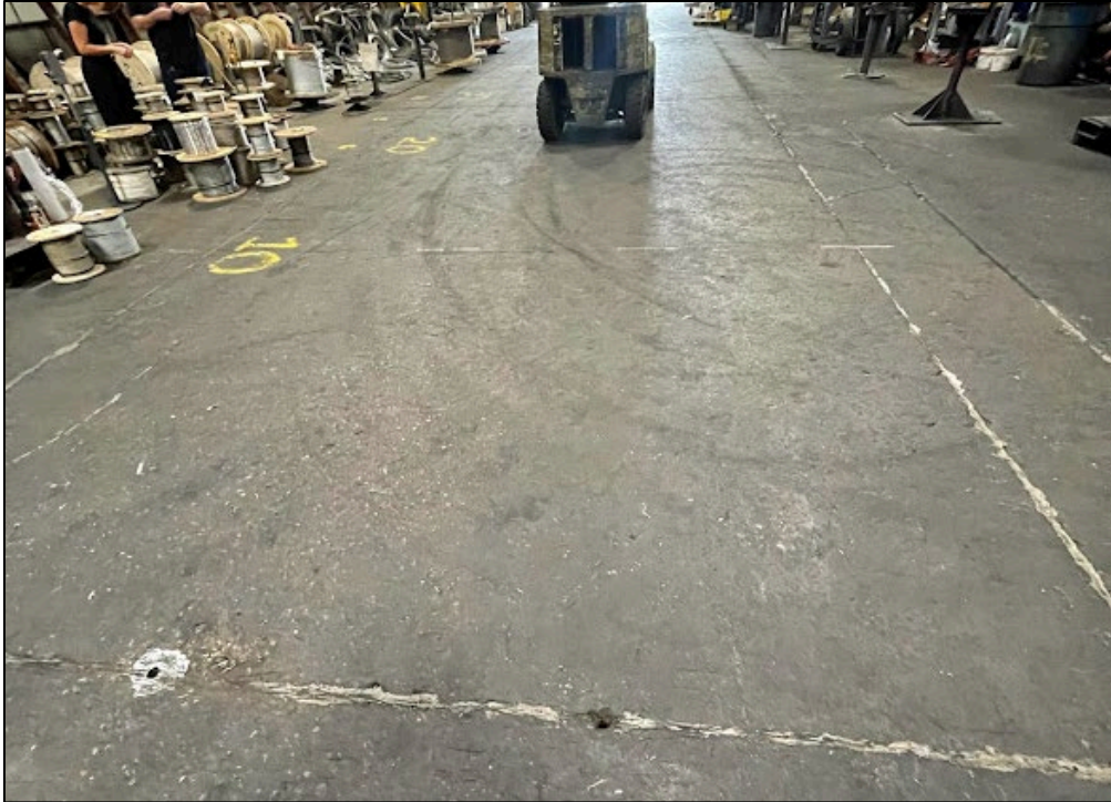
Area 9 showing sealant peeling from seams and unsealed drill holes
