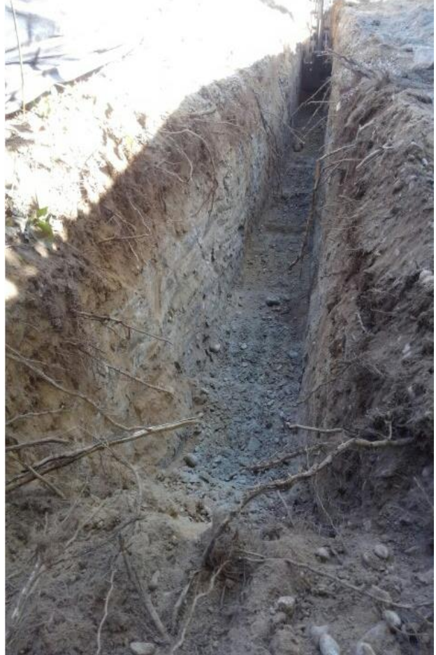
Part of Cleanup of SS-4 area and confirmation sample taken from this area
