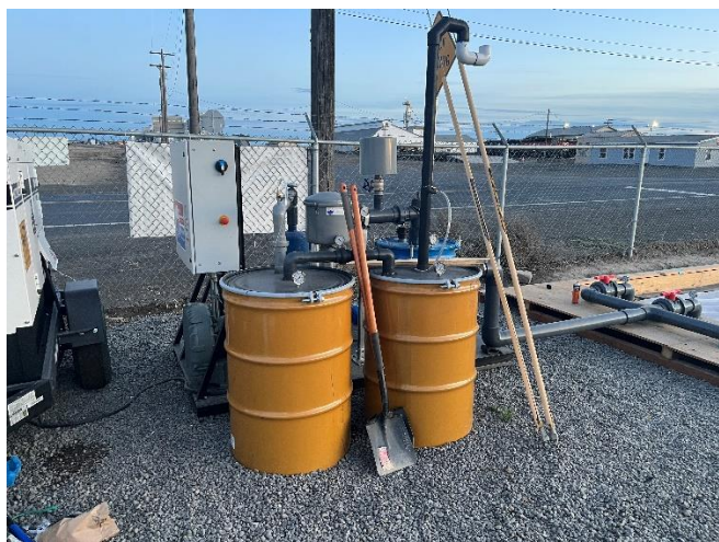
Photo 5. View of SVE equipment.
