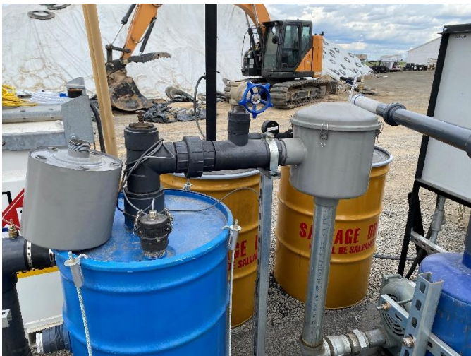
Photo 3. Partial view of SVE system.
