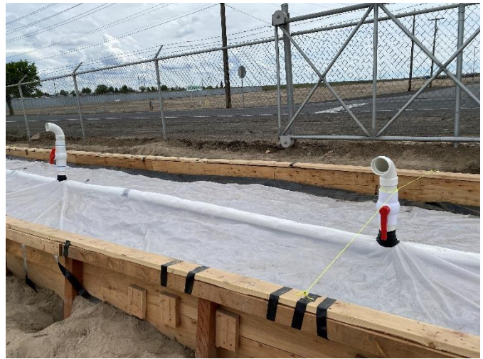
Photo 2. View of tubing on top of treatment cell, facing south. Note vacuum effect on top liner across treatment cell. Suction pulling liner taut against air inlet piping array.
