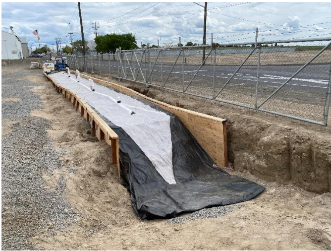
Photo 1. View of loaded treatment cell, facing southeast.
