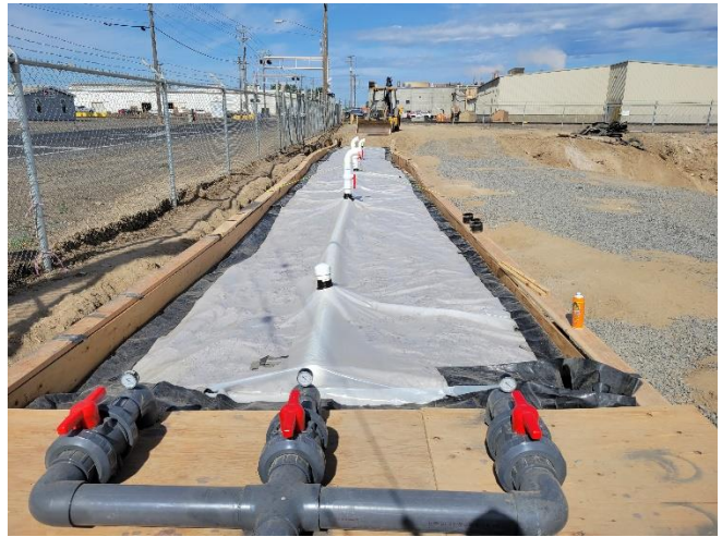
Photo 8. View of SVE treatment cell.
