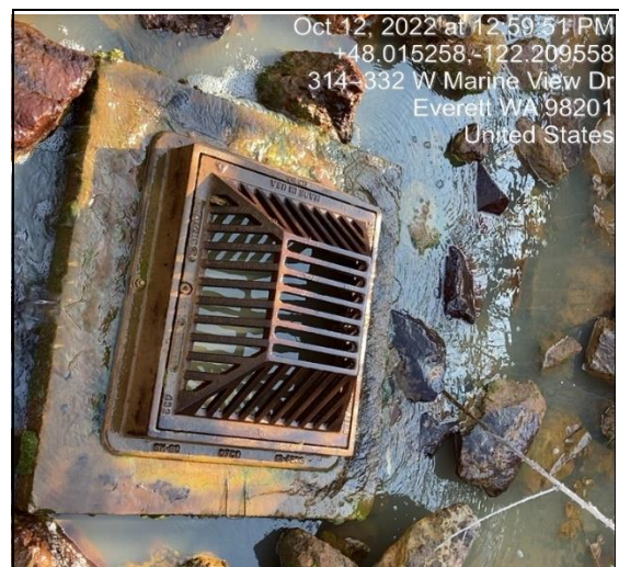
4. SWM staff measured the conductivity of this CB after the purging process at >1900 us/cm. SWM staff pulled a water quality sample from this catch basin for Oil and Grease, Metals, and Ammonia-N. Currently waiting on the lab results.
