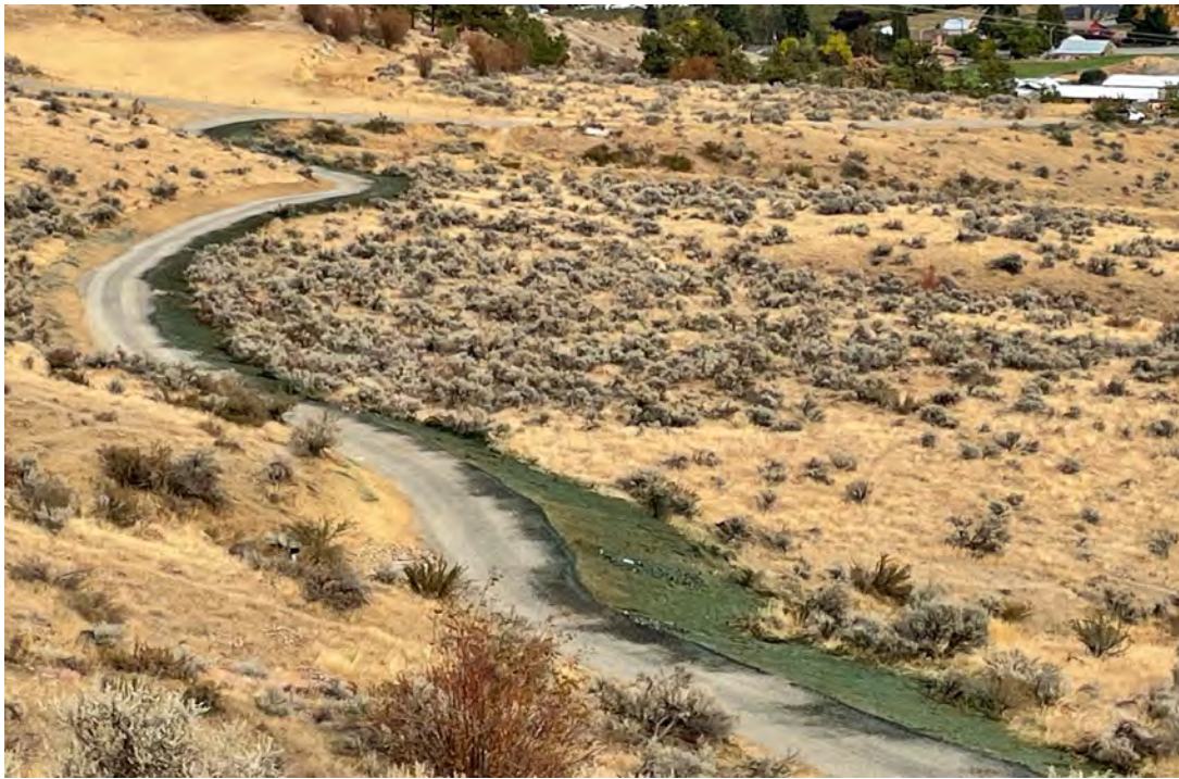
Photograph 14. Example hydroseeding activities along lower Phase 2 haul road and the former SR02 staging area.
