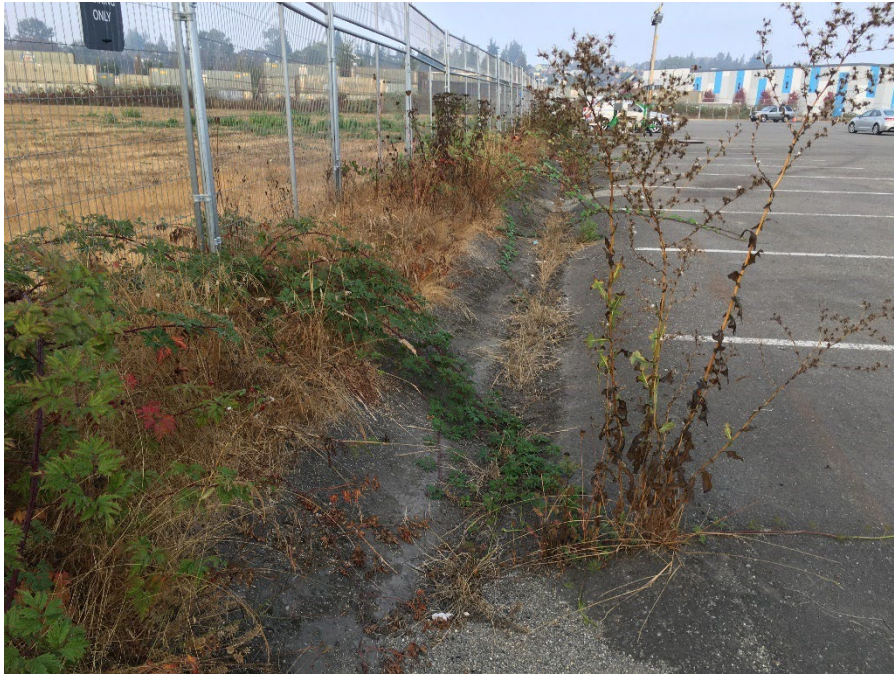
Photo 3. Looking west at the south drainage ditch. Less than 1 inch of accumulated sediment was observed. Vegetation was observed to be growing through minor cracks.
