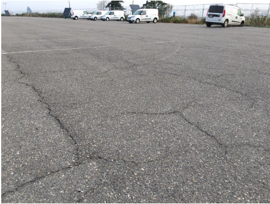
Photo 2. Looking north-northeast at the southern portion of the asphalt cap, observing minor cracking.
