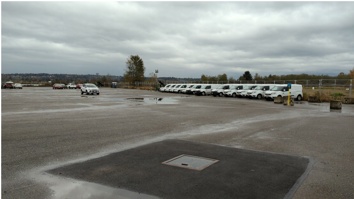
Photo 5. Facing southeast at the western and southern portions of the asphalt cap. Minor ponding is observed after a rainfall event.
