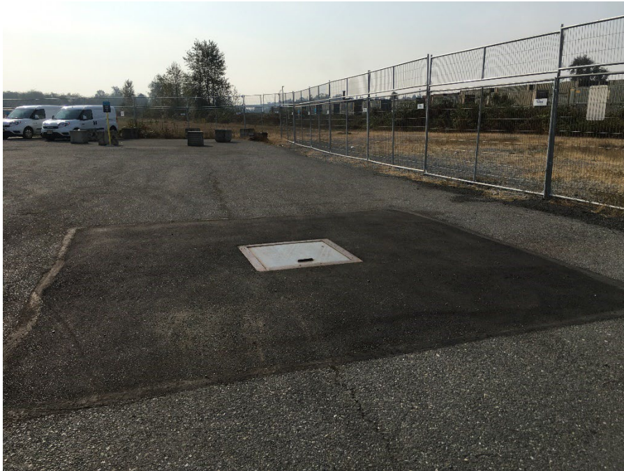
Photo 4. Observing minor cracking on the surface of the asphalt cap in the south portion of the asphalt cap.
