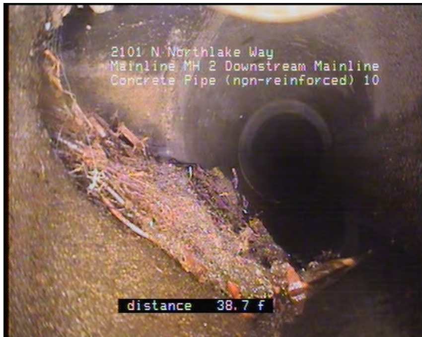
Photo: Mainline MH 2_Mainline MH104331_25062010_A.JPG, VCR No.: Floyd/Gas Works 06.25.2010 38.7FT, Roots Fine Lateral, from 03 to 09 o'clock
