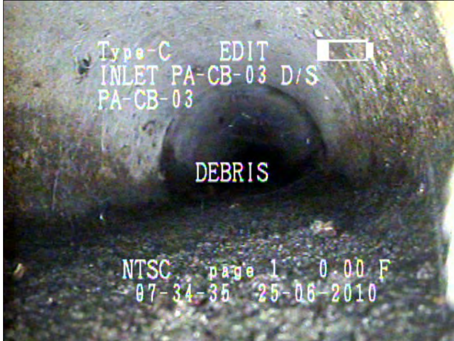
Photo: Inlet PA-CB-03_PA-CB-03041601_28062010_A.jpg, VCR No.: Floyd/Gas Works 06.25.2010 0FT, Deposits Settled Fine, 5 %of cross sectional area, from 05 to 07 o'clock, , within 8 inches of joint: YES, Start
