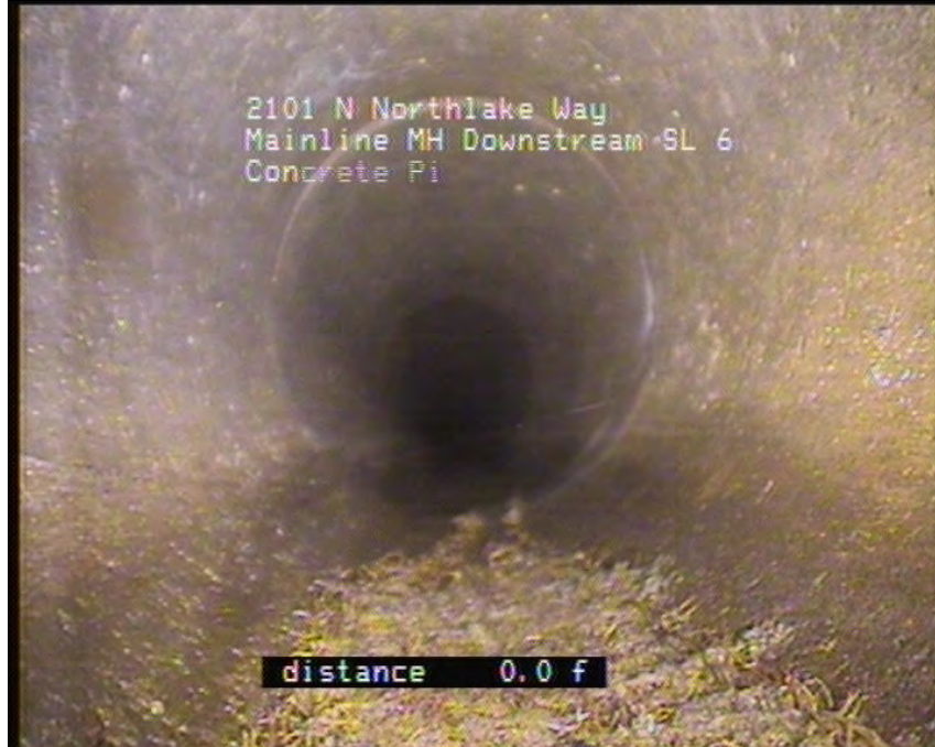
Photo: Mainline MH_SL 6101118_25062010_A.JPG, VCR No.: Floyd/Gas Works 06.25.2010 OFT, Roots Fine Joint, from 05 to 07 o'clock, within 8 inches of joint: YES / In MH
