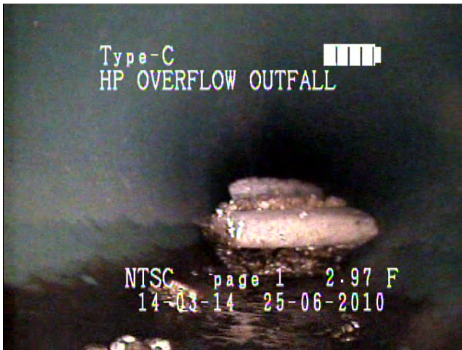
Photo: HP-CB-01_HP Over flow081251_30062010_A.jpg, VCR No.: Floyd/Gas Works 06.25.2010 5.6FT, Obstacles Rocks, 20 %of cross sectional area, from 04 to 08 o'clock
