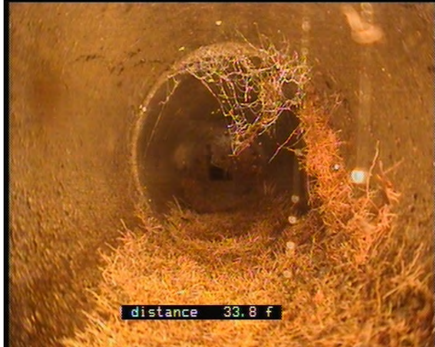
Photo: PA-CB-01_Mainline MH2111028_25062010_A.JPG, VCR No.: Floyd/Gas Works 06.25.2010 33.8FT, Roots Fine Barrell, from 04 to 07 o'clock, Start
