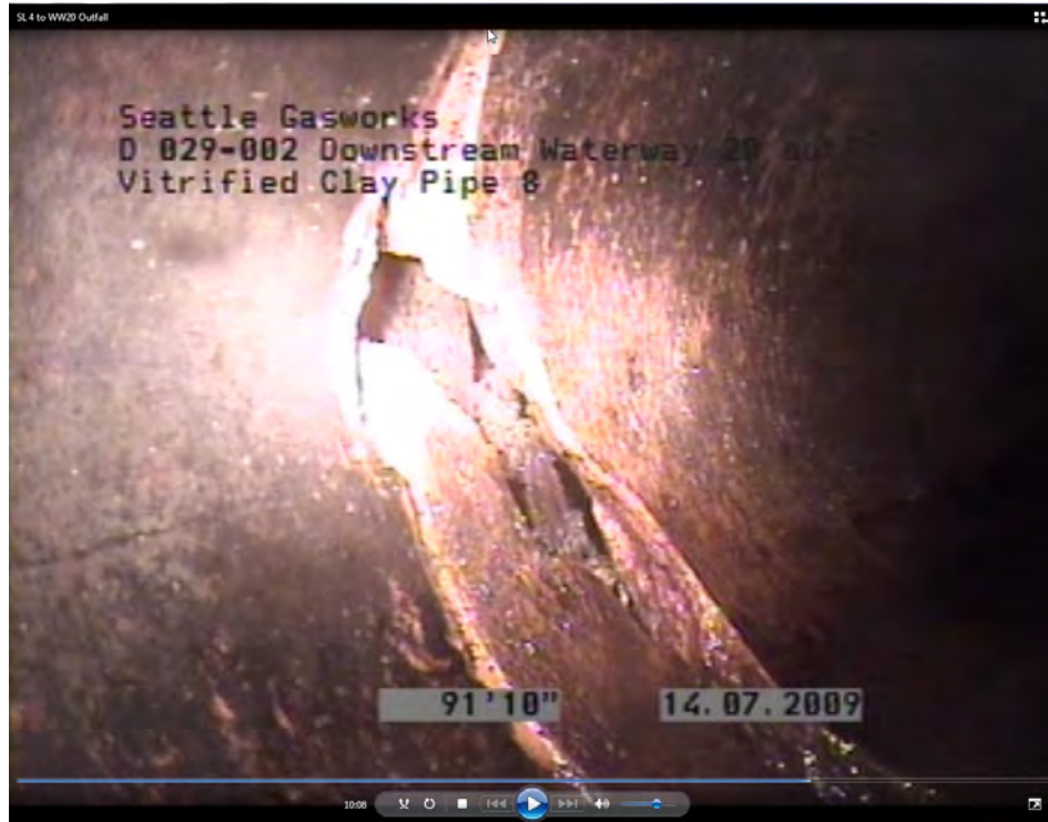
Photograph 5. SL 4 to WW20 Outfall, hole at 91 feet from SL 4.
