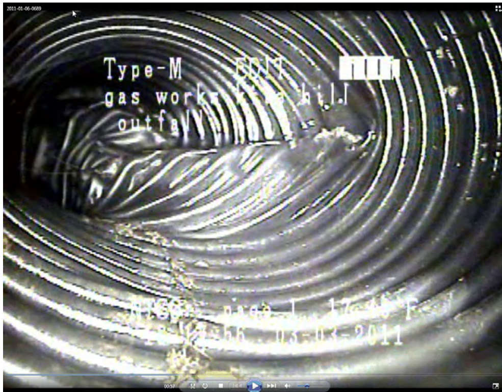
Photograph 2. Video capture of crushed pipe 20 feet from Kite Hill Outfall. January 5, 2011.
