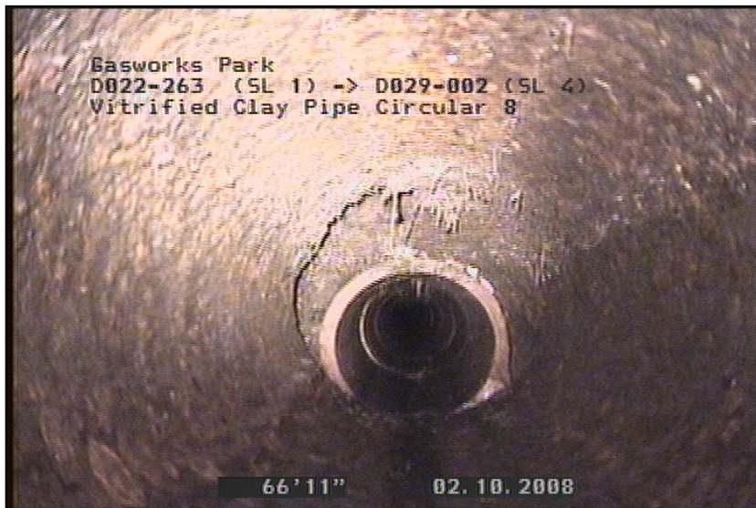
Photo: D022-263 (SL 1)_D029-002 (SL 4)_100208_093301_A.JPG, VCR #: GS-10.1.08 66.88FT, Material Change, Steel pipe, REMARK:
