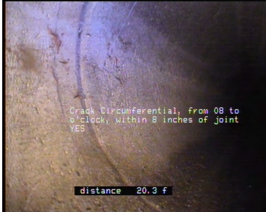
Photo: Mainline MH 2_Mainline MH104104_25062010_A.JPG, VCR No.: Floyd/Gas Works 06.25.2010 20.3FT, Crack Circumferential, from 08 to 12 o'clock, within 8 inches of joint: YES
