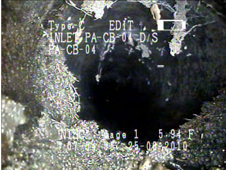
Photo: Inlet PA-CB-04_PA-CB-04043034_28062010_A.jpg, VCR No.: Floyd/Gas Works 06.25.2010 5.59FT, Roots Fine Joint, from 03 to 09 o'clock, within 8 inches of joint: YES
