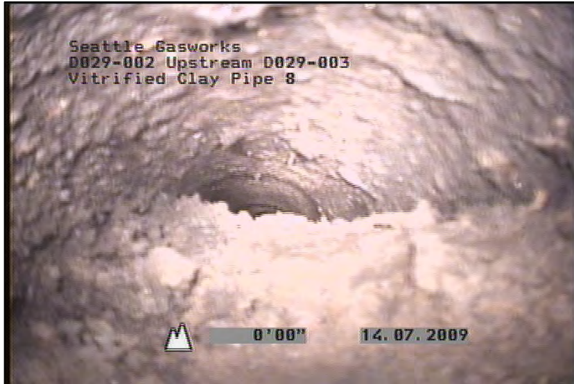
Photo: D029-003_D029-002_071409_112611_A.JPG, 00:00:23 0FT, Deposits Settled Fine, 80 %of cross sectional area, from 02 to 10 o'clock, within 8 inches of joint: YES
