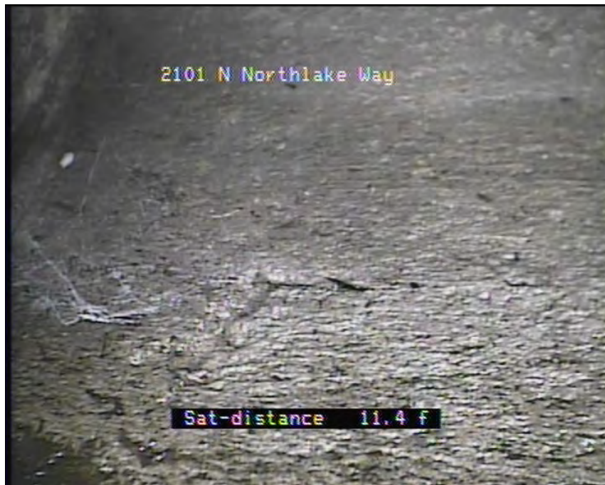
Photo: PA-CB-07_Discharge Point095656_25062010_A.JPG, VCR No.: Floyd/Gas Works 06.25.2010 11.4FT, Crack Longitudinal, at 05 o'clock, within 8 inches of joint: YES
