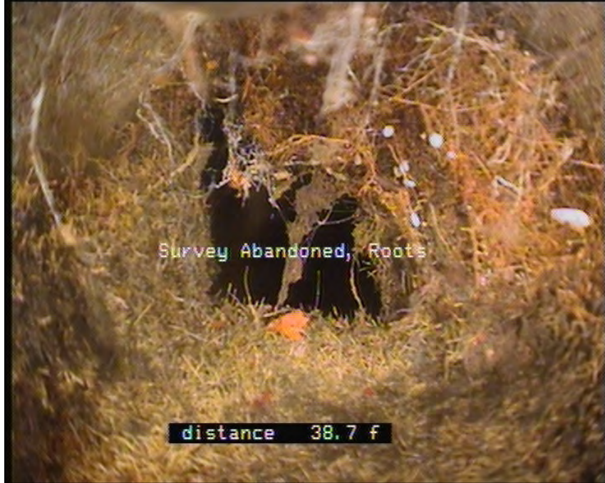
Photo: PA-CB-01_Mainline MH2111230_25062010_A.JPG, VCR No.: Floyd/Gas Works 06.25.2010 38.7FT, Survey Abandoned / Roots
