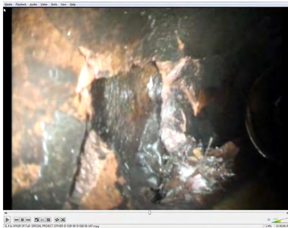
Photograph 6. SL 4 to WW20 Outfall, hole at ~94 feet from SL 4.
