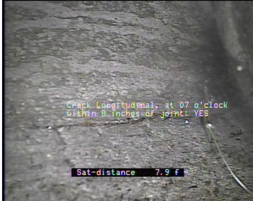
Photo: PA-CB-07_Discharge Point095517_25062010_A.JPG, VCR No.: Floyd/Gas Works 06.25.2010 7.9FT, Crack Longitudinal, at 07 o'clock, within 8 inches of joint: YES
