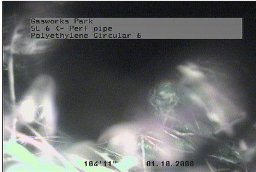
Photo: SL 6_Perf pipe_100108_141203_A.JPG, VCR #: GS-10.1.08 104.95FT, Roots Fine Barrell, from 12 to 12 o'clock, within 8 inches of joint: YES
