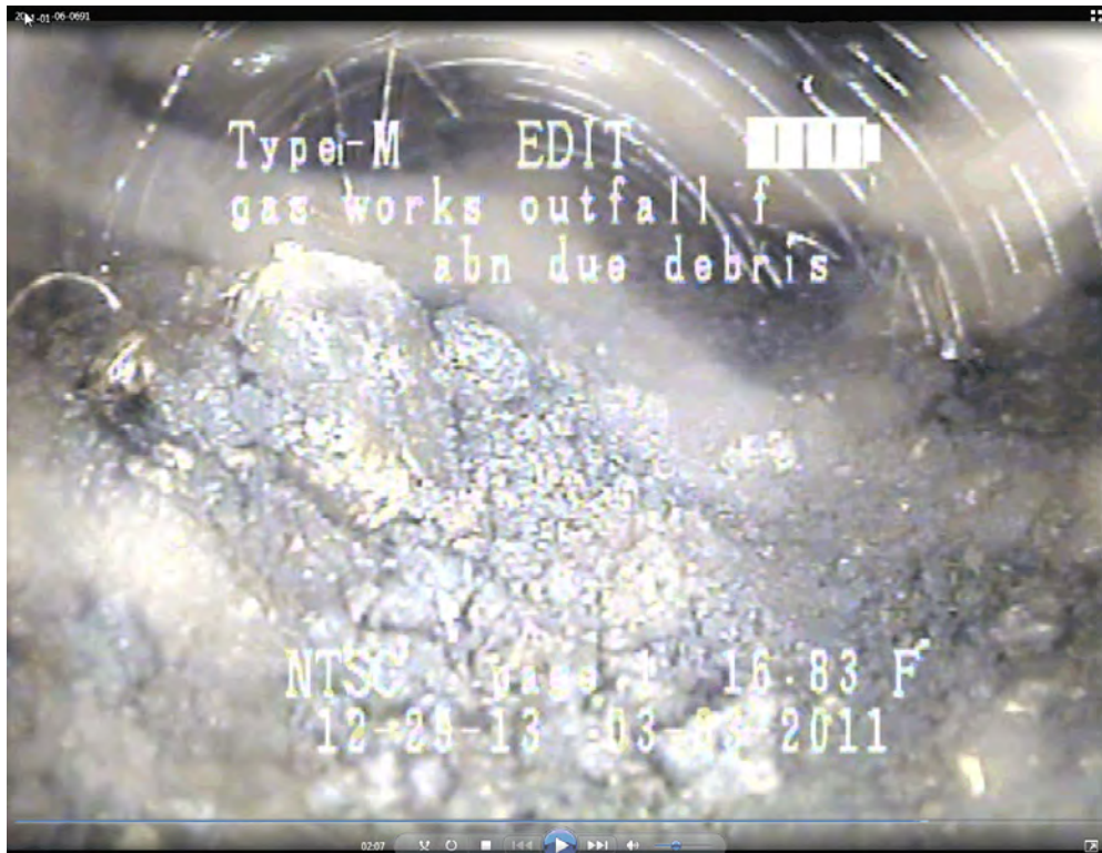
Photograph 8. Video capture of filled pipe 18 feet from Outfall F. January 5, 2011.
