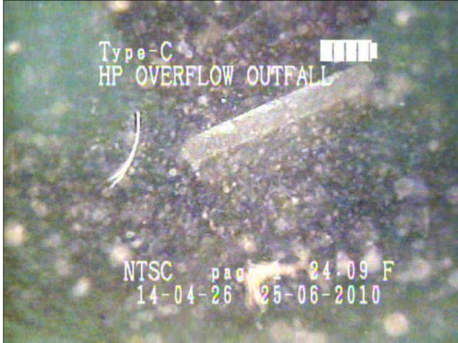
Photo: HP-CB-01_HP Over flow081441_30062010_A.jpg, VCR No.: Floyd/Gas Works 06.25.2010 24.1FT, Obstacles Other, 15 %of cross sectional area, from 10 to 02 o'clock / Wood
