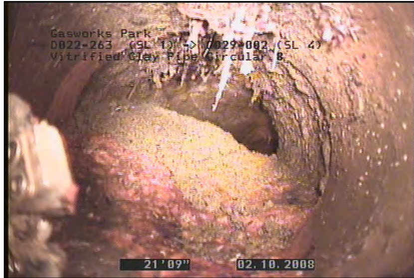
Photo: D022-263 (SL 1)_D029-002 (SL 4)_100208_092533_A.JPG, VCR #: GS-10.1.08 21.76FT, Tap Factory Made Defective, at 09 o'clock, 6", within 8 inches of joint: NO, REMARK: Debris
