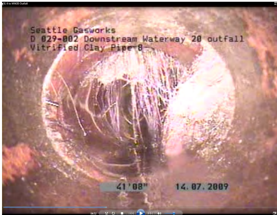
Photograph 4. SL 4 to WW20 Outfall, roots and soil intrusion at 41 feet from SL 4.
