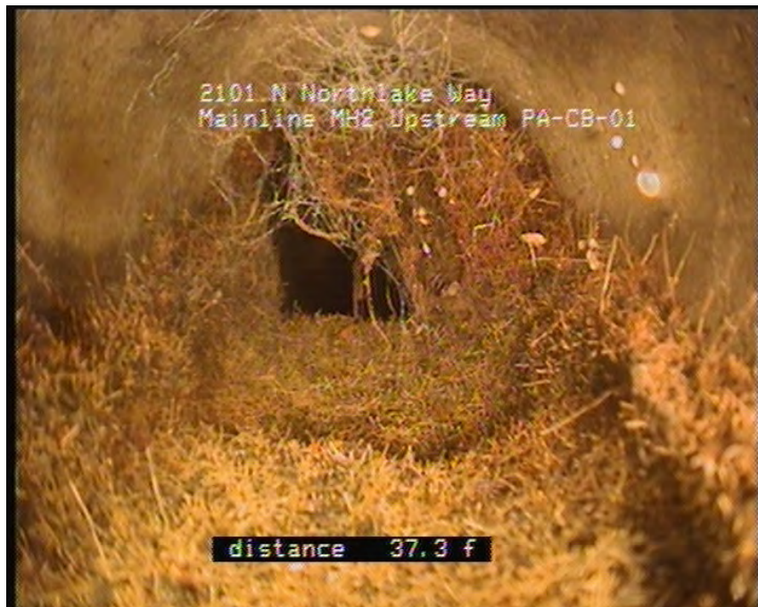
Photo: PA-CB-01_Mainline MH2111128_25062010_A.JPG, VCR No.: Floyd/Gas Works 06.25.2010 37.3FT, Roots Ball Barrell, from 02 to 09 o'clock, 50 %, within 8 inches of joint: YES, Start
