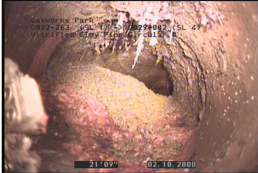
Photo: D022-263 (SL 1)_D029-002 (SL 4)_100208_092533_A.JPG, VCR #: GS-10.1.08 21.76FT, Tap Factory Made Defective, at 09 o'clock, 6", within 8 inches of joint: NO, REMARK: Debris
