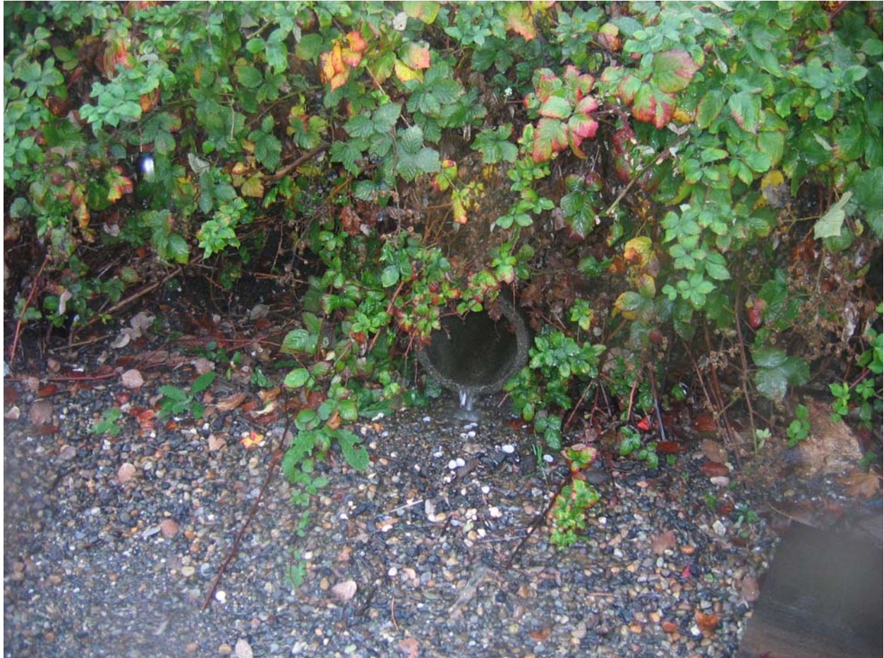
Photo 3: Outfall C during a storm, November 2006.
