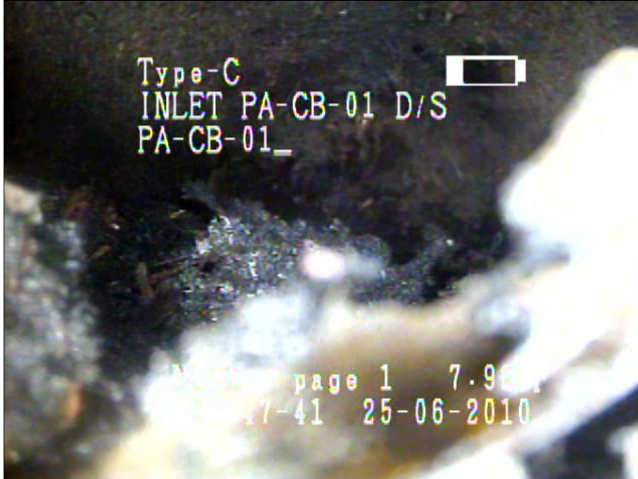
Photo: Inlet PA-CB-01_PA-CB-01042535_28062010_A.jpg, VCR No.: Floyd/Gas Works 06.25.2010 0FT, Deposits Settled Fine, 20 %of cross sectional area, from 03 to 09 o'clock, , within 8 inches of joint: YES
