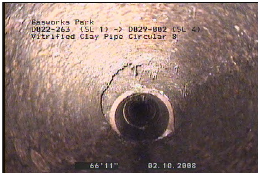
Photo: D022-263 (SL 1)_D029-002 (SL 4)_100208_093301_A.JPG, VCR #: GS-10.1.08 66.88FT, Material Change, Steel pipe, REMARK:
