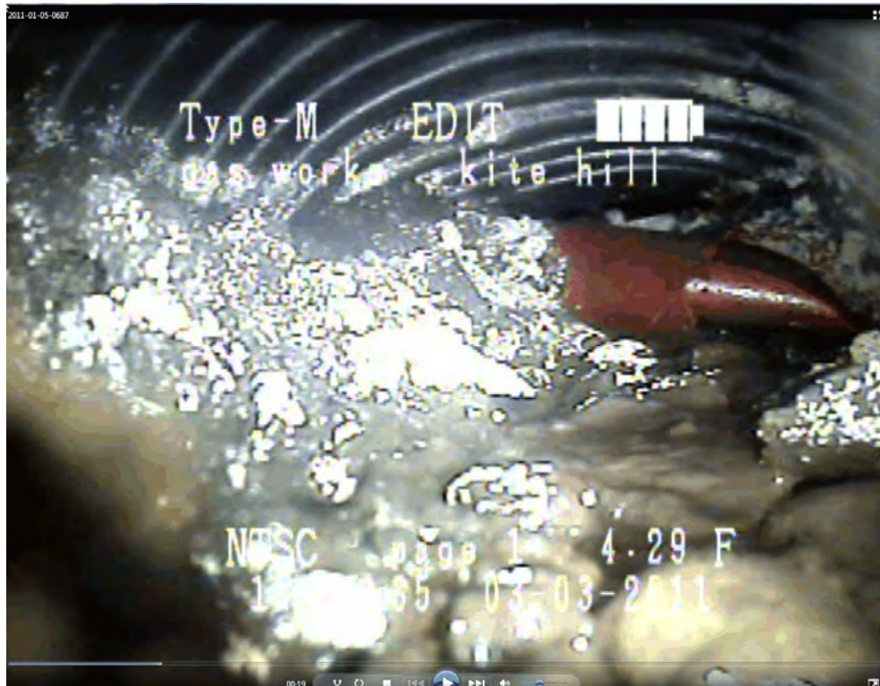
Photograph 6. Video capture of Kite Hill Manhole to completely filled Northern Inlet. January 5, 2011.
