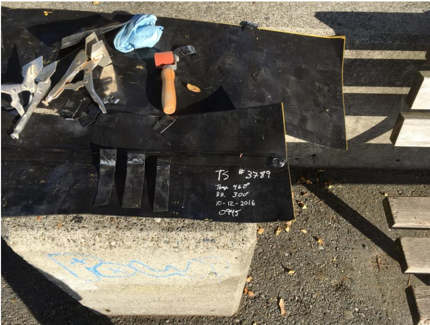
Testing out of DemTech extrusion welding machine prior to use to make patches
