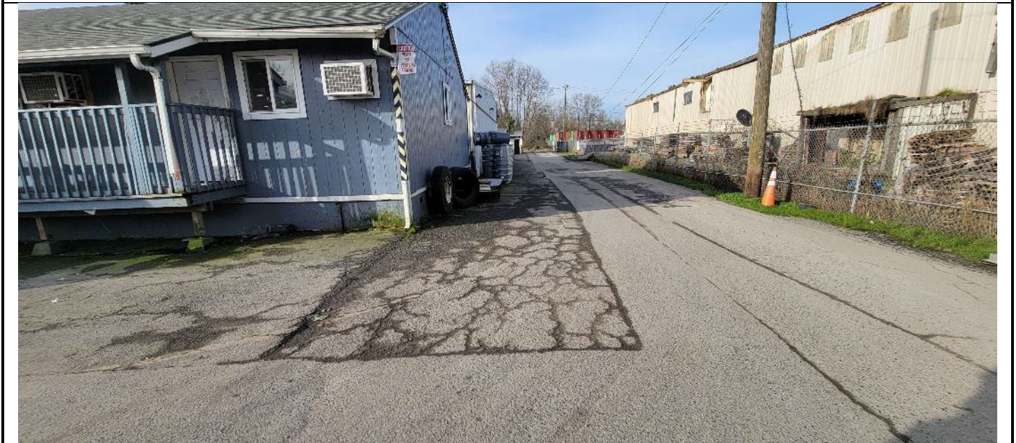
Alligator cracking northeast and north of lunchroom building. Multiple concrete patches in area.
