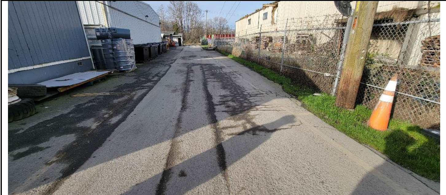
Alligator cracking on north side of shop along main truck route. Some cracking along north asphalt edge. Additional asphalt patch areas.
