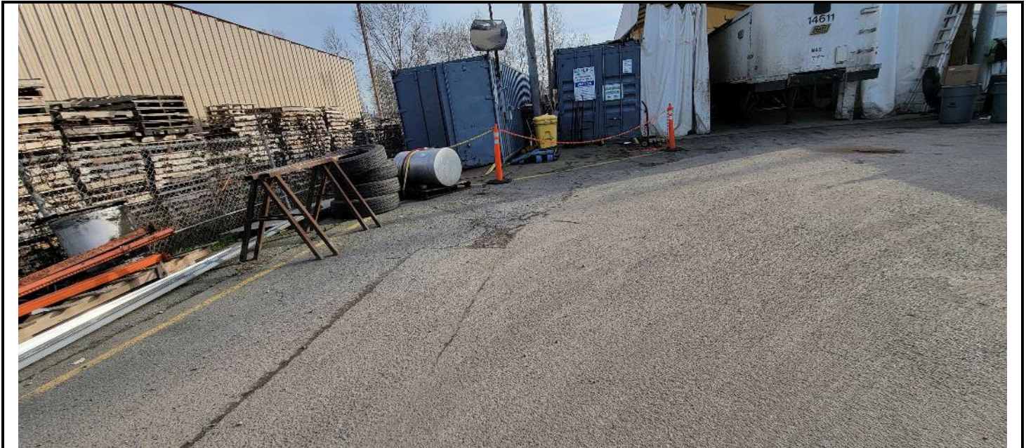
Small area of alligator cracking at end of concrete patch near truck shop.
