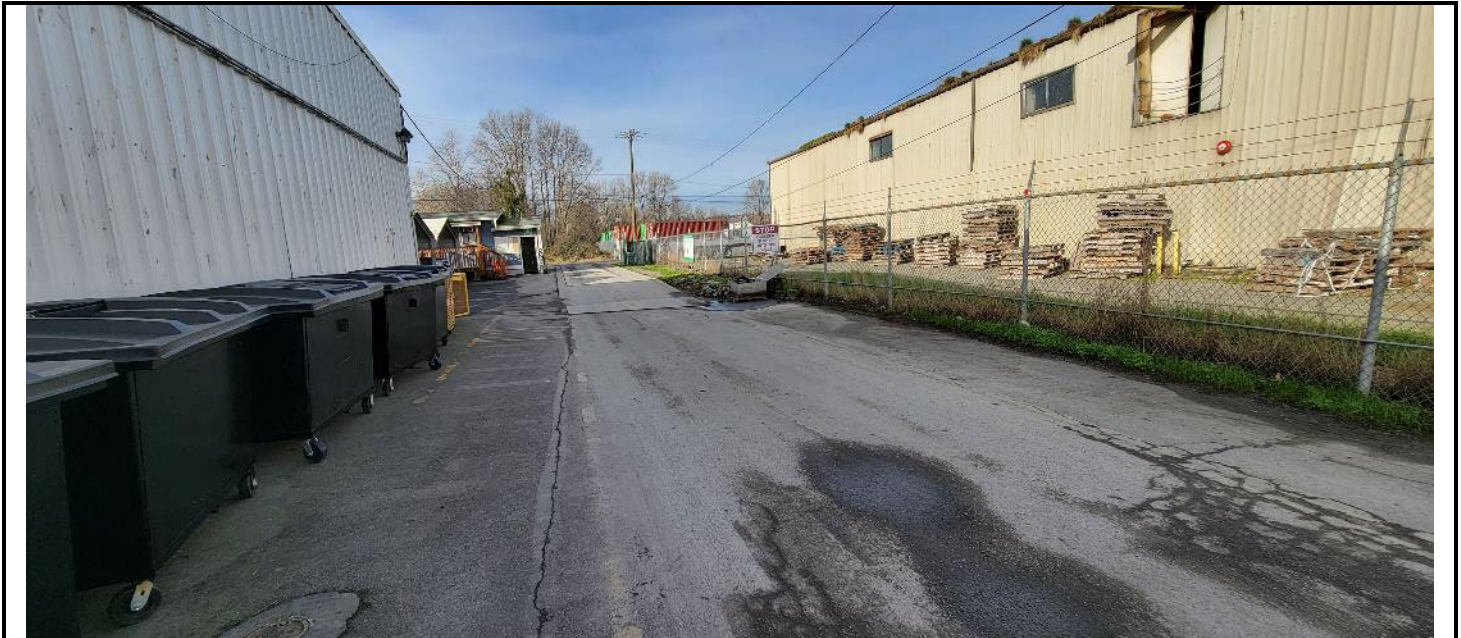
Linear crack that may have received patch material in the past; located n north side of shop near well MFG-1 (bottom left circular feature in photograph).
