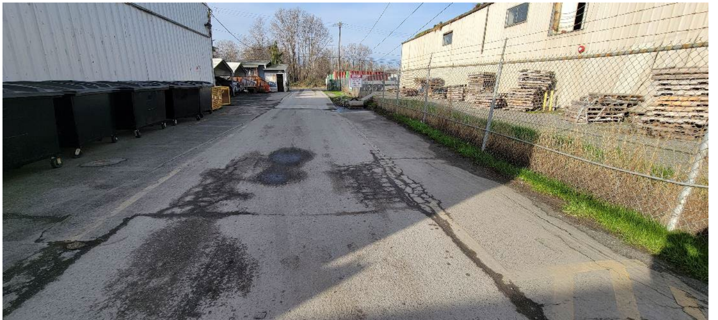
More alligator cracking along truck route north of shop.
