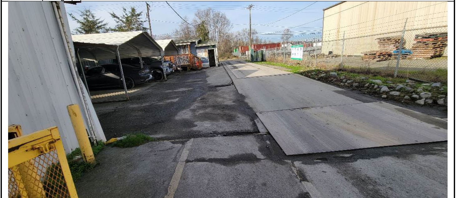
Miscellaneous small linear cracks near truck scale and car ports. Drain cut from building to weigh scale ramp in middle left of photograph.
