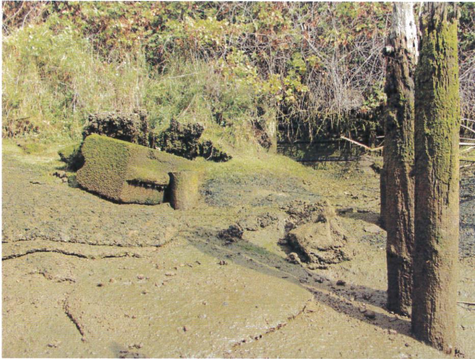
Conditions Near East End of Block Wall North Bank (view to northwest)
