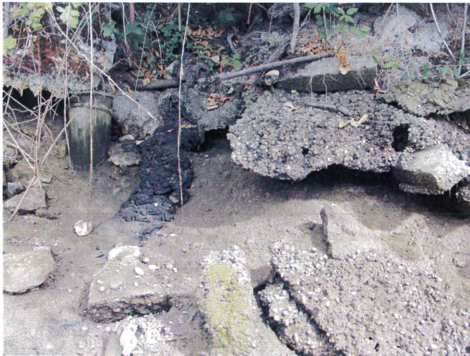
Asphalt-Like Material North Bank (view to north)
