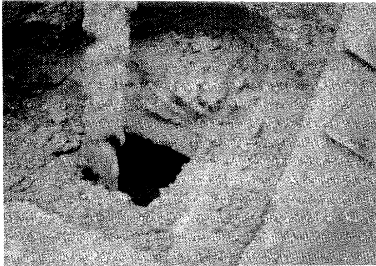
PHOTOGRAPH 4. Controlled density fill material was used to decommission the UST in place.
