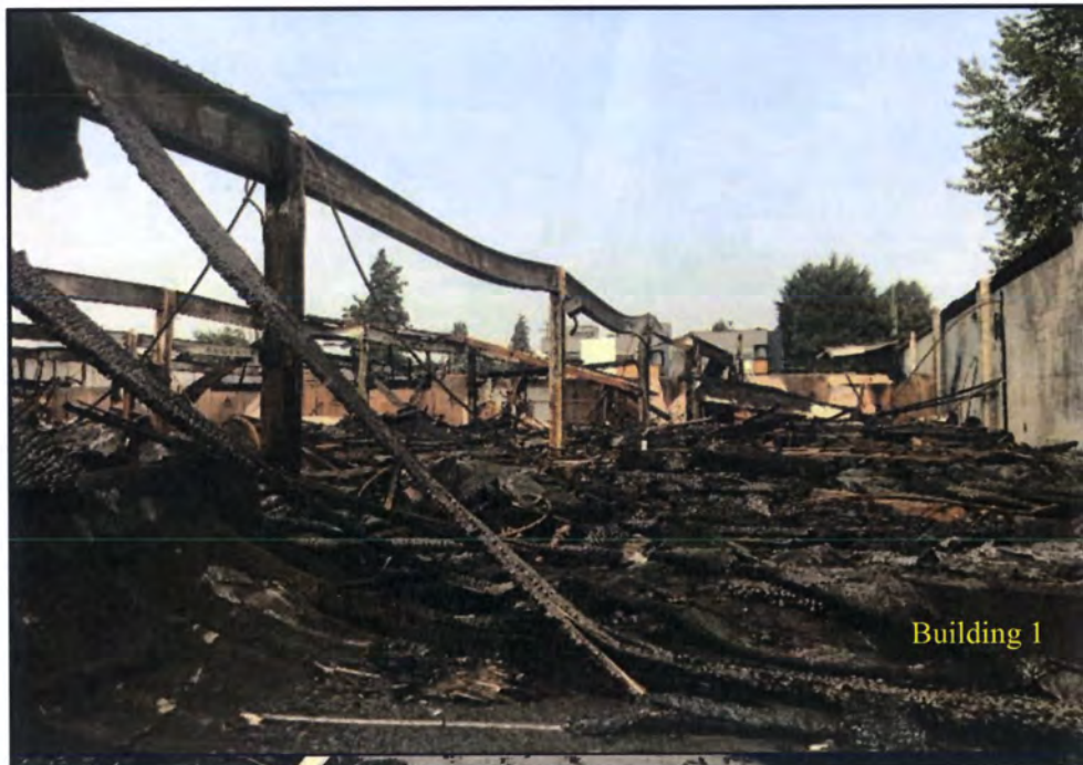
Photograph 6. Fire damaged Building 1 – Looking Southeast
