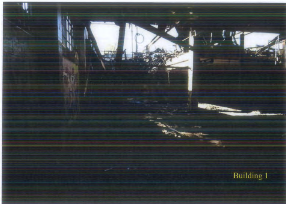
Photograph 7. Fire damaged Building 1 – Looking South
