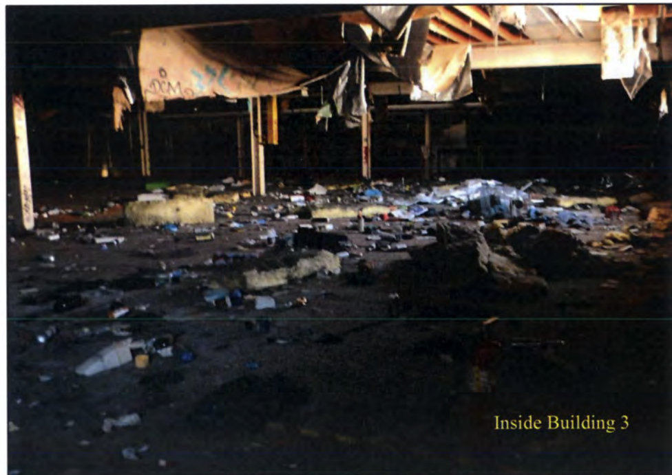
Photograph 10. Damaged roof and evidence of unsafe occupancy inside Building 3 – Looking North
