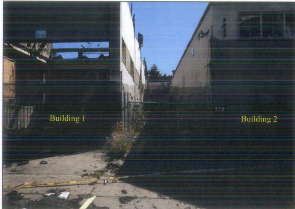
Photograph 8. Proximity of Building 1 (south wall) to the Building 2 (north wall) – Looking East
