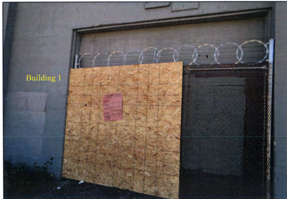
Photograph 2. View of SDCI Emergency Order on west wall of Building 1 – Looking Northeast
