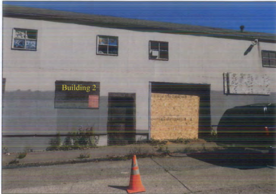
Photograph 3. View of SDCI Emergency Order on south wall of Building 2 – Looking North
