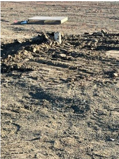
Photograph 8. Localized depression around test grouted helical pile backfilled by Budinger & Associates, Inc. and photographed by Garco on January 30, 2023.
