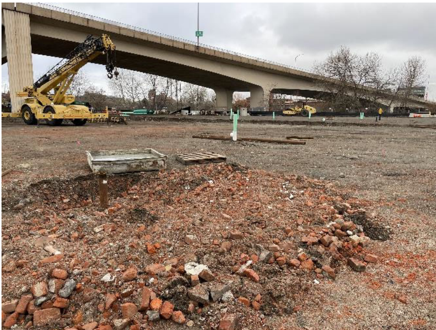
Photograph 6. Localized depression around test grouted helical piles within Building 2A footprint. Photo taken January 17, 2023.
