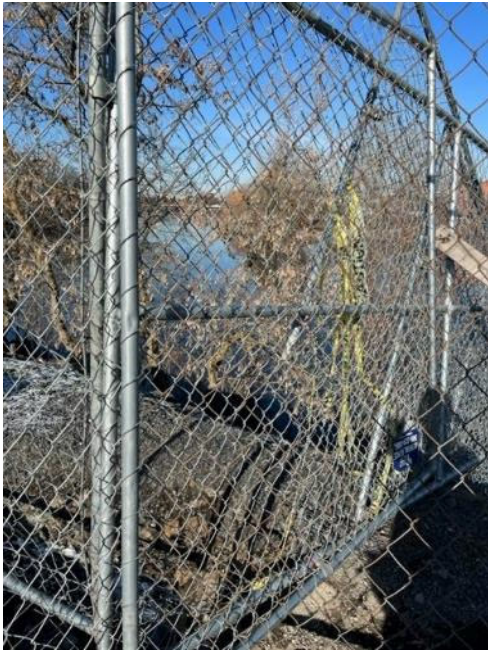
Photograph 5. Hole in temporary construction fence at the west end of the Site, repaired and photographed by Garco on January 30, 2023.
