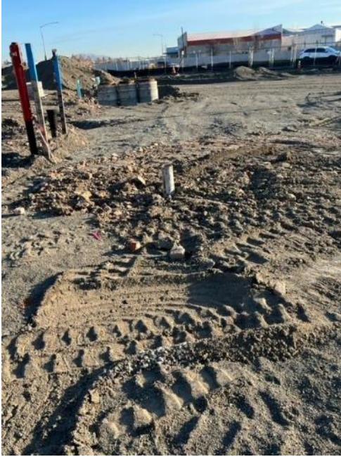
Photograph 7. Localized depression around test grouted helical pile backfilled by Budinger & Associates, Inc. and photographed by Garco on January 30, 2023.
