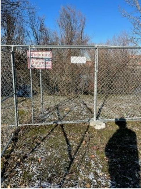
Photograph 3. Hole in temporary construction fence in the northeast portion of the Site, repaired and photographed by Garco on January 30, 2023.
