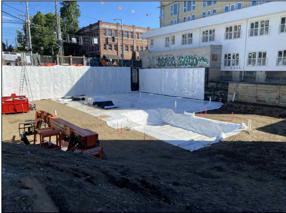
Photograph 3: View of Pretak sheet being installed along the south and east shoring walls in the location where the slab was to be poured.
