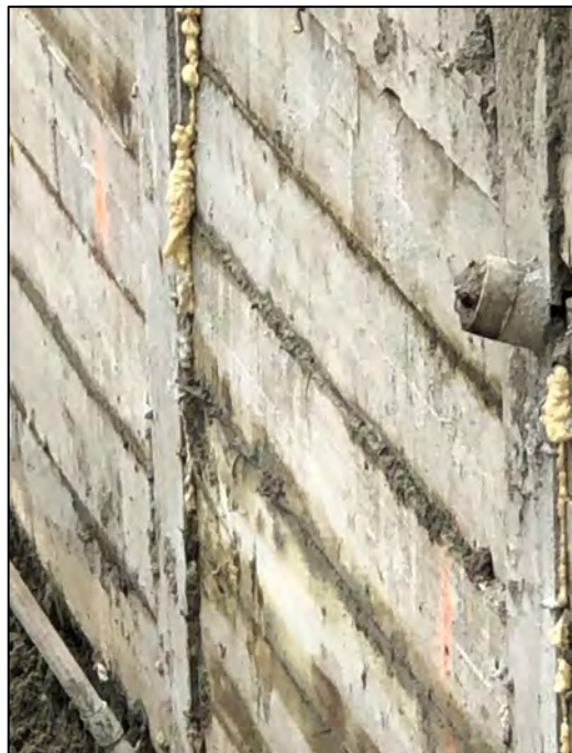
Photograph 4: View showing penetrations in the shoring wall that were sealed using Pretak tape, Benotak, and Estop GU as part of the chemical vapor barrier installation.
