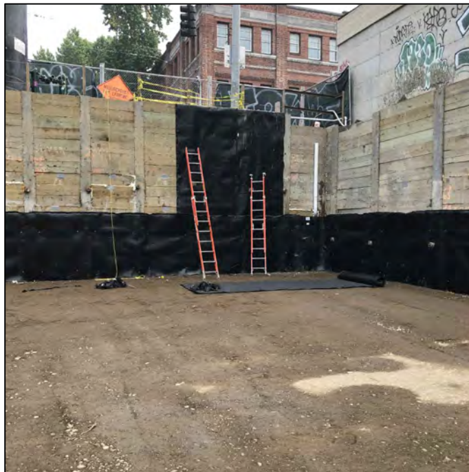
Photograph 2: View of E Drain 6000 being installed along the south and east shoring walls.
