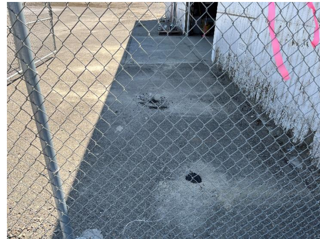
Photo 18. View of bore holes advanced near northeast corner of warehouse during Phase 3 soil sampling activities. Photo taken on 8/26/2022.
