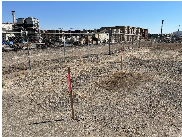
Photo 19. View of bore holes advanced near northern site boundary during Phase 3 soil sampling activities. Photo taken on 8/26/2022.
