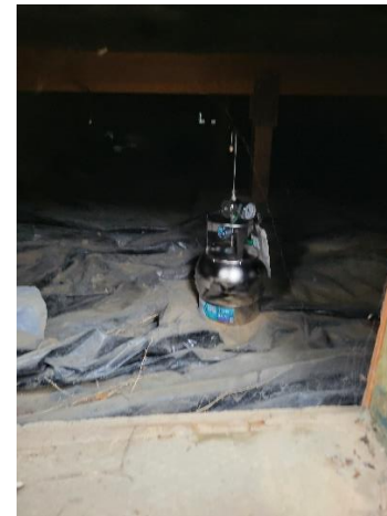
Photo 10. View of crawl space air sample collected from crawl space under the modular office building. Photo taken on 5/11/2022.
