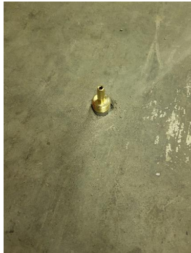
Photo 3. View of vapor pin installed in warehouse floor slab. Photo taken on 5/11/2022.
