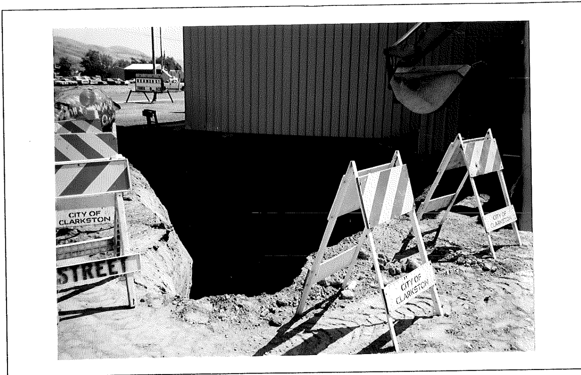
VIEW OF THE EXCAVATION LOOKING NORTHEAST WITH THE SHOP BUILDING AND BRIDGE STREET IN THE BACKGROUND.
