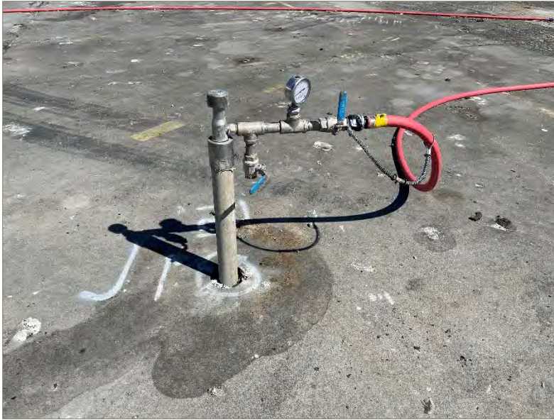
Exhibit 6-4: Photo of an Injection Point with 5-Foot Injection Tool Inserted (Watermarks are From Concrete Cutting)
