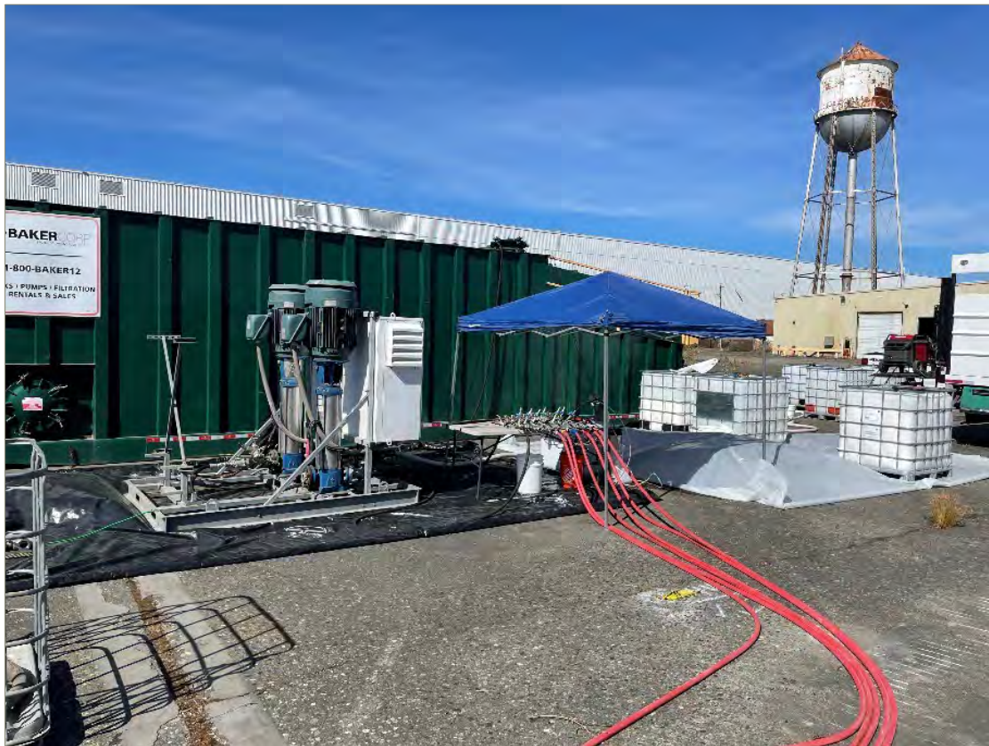
Exhibit 6-1: Photo of Pumping Assembly with Mixing Tank Used for Mixing of Remediation Compounds
