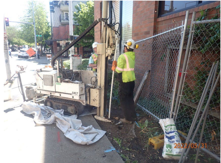
View south of drill rig set up on EB04 in landscaping next to Greenwood Avenue right-of-way.
