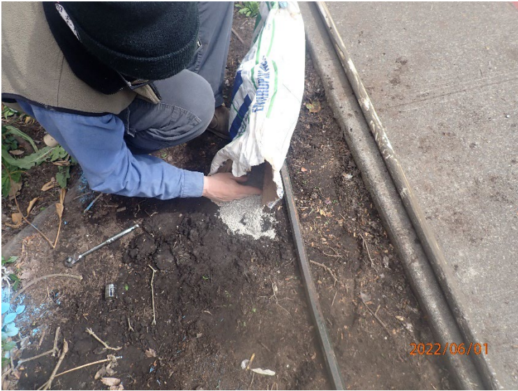
Following sampling activities, temporary reconnaissance borings were backfilled and sealed at the surface.
