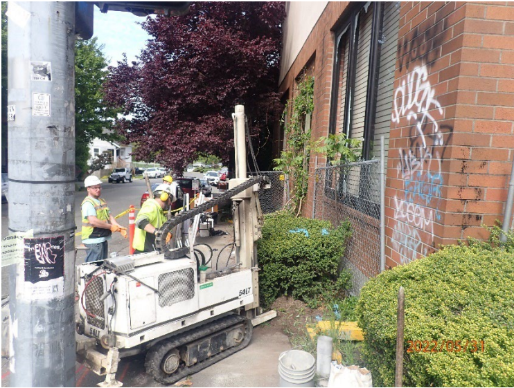
View west of drill rig set up on first attempt at EMW01.
