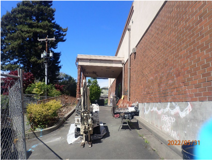
View north of drill rig set up on EB05 on west side of building.
