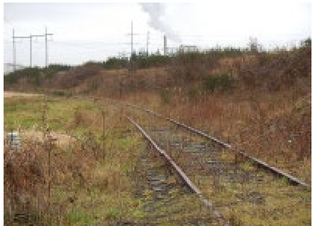
Abandoned rails on ground surface
