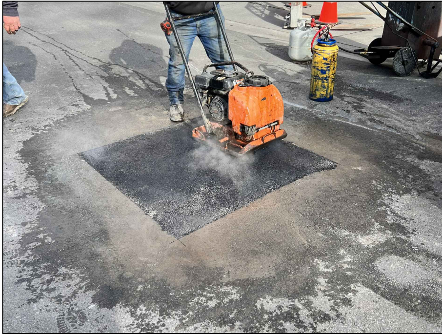
Photograph 5: View of well MW-5 location after backfilling with 6 inches of hot mix asphalt and finishing asphalt with an asphalt plate compactor.
