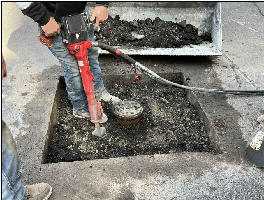
Photograph 2: View of 4' x 4' area where asphalt was saw cut around well MW-5 after decommissioning was completed.
