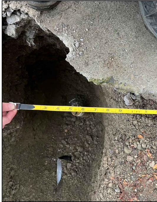
Photograph 3: View of well MW-10 after the well casing was cut to a depth approximately 18 inches below surface grade and prior to covering the well casing with gravel.
