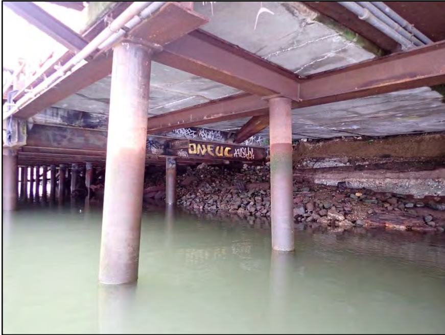
Photo 17 : Typical condition of steel piles and underdeck superstructure under northerly wheelhouse extension, looking south.
