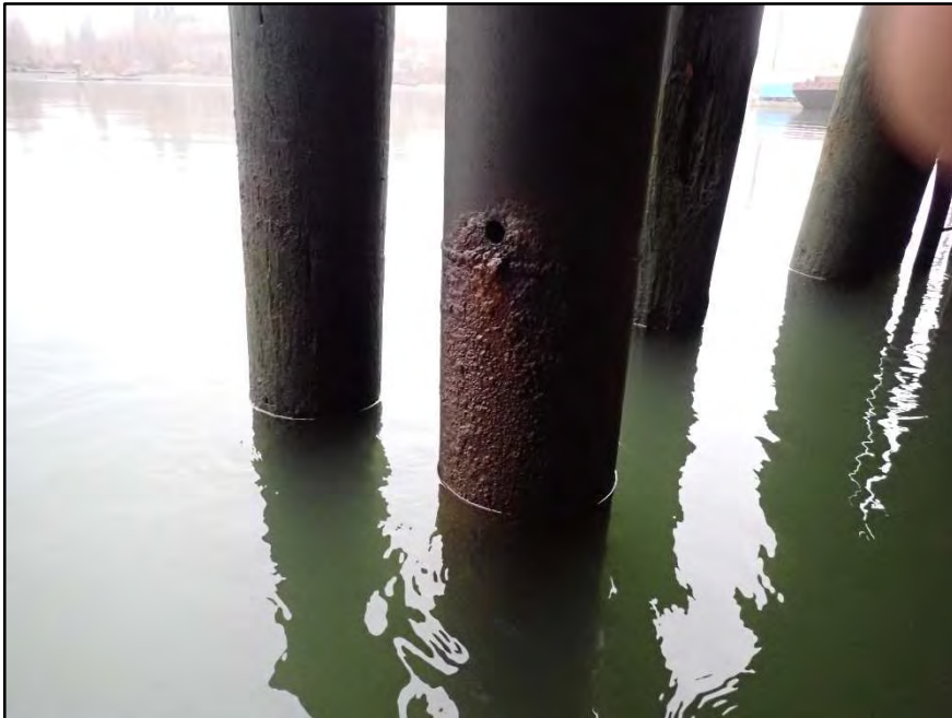
Photo 12 : Nodular corrosion below welded splice, Bent 11 Pile A, looking southeast.
