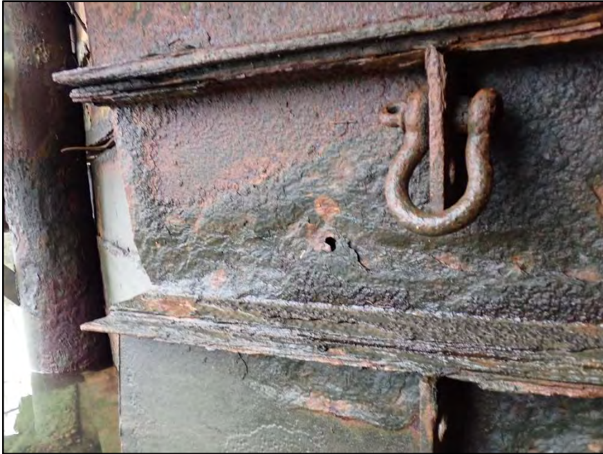
Photo 15 : Typical corrosion on steel bulkhead, looking southwest.
