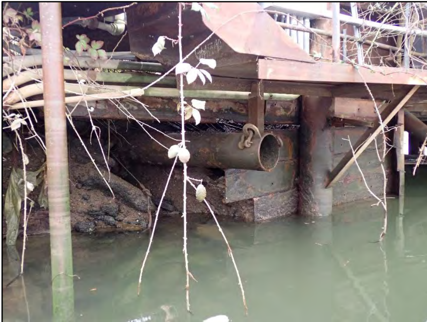
Photo 6 : Erosion behind south wingwall, looking north.
