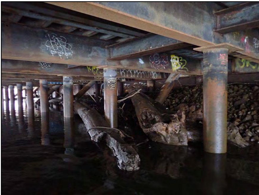
Photo 8 : Typical timber debris accumulation, looking south.
