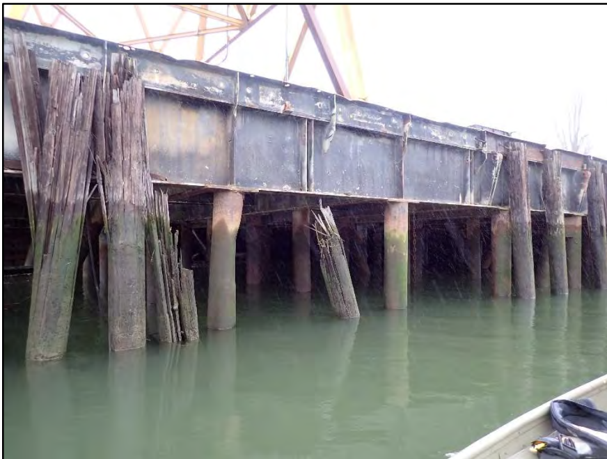
Photo 16 : Fractured fender piles, Bents 2-3, looking west.
