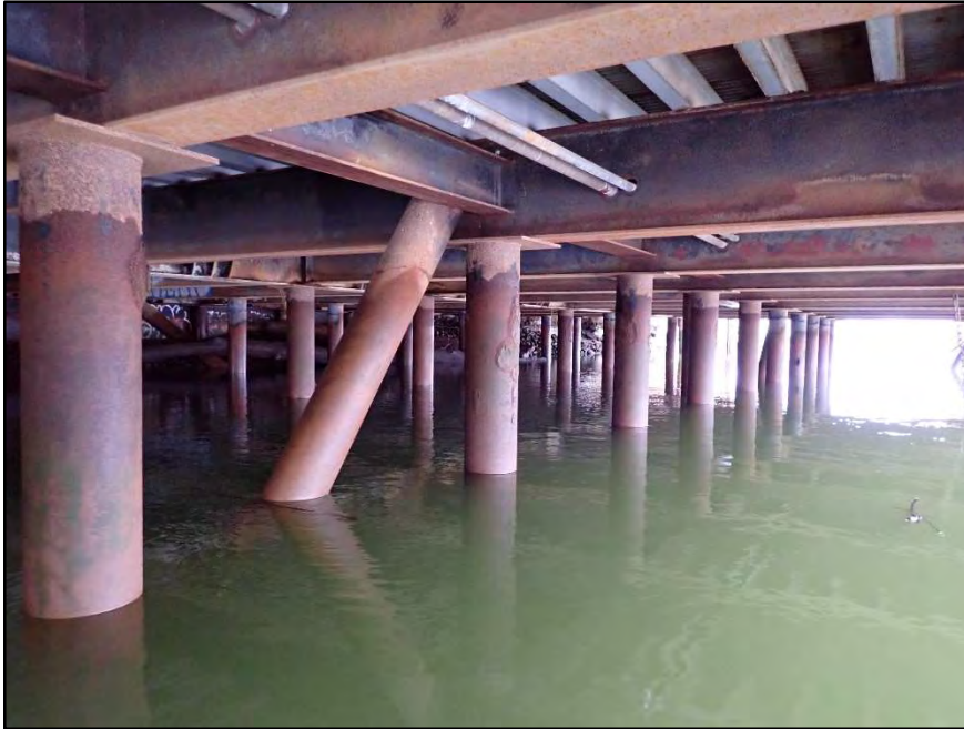
Photo 9 : Typical condition of steel piles and underdeck superstructure, C piles from Bent 6, looking northwest.
