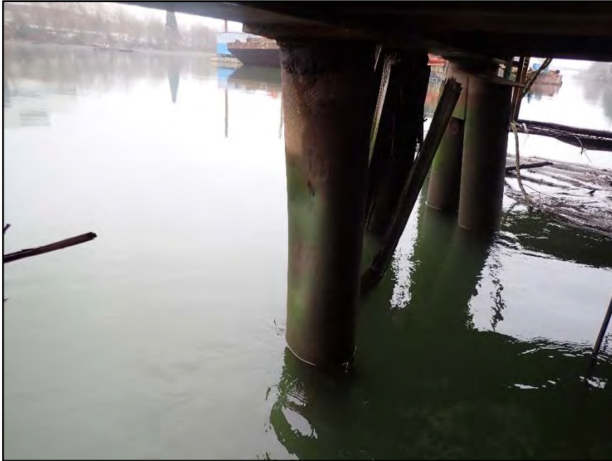
Photo 13 : Pile deformation, Bent 2 Pile A, looking southeast.
