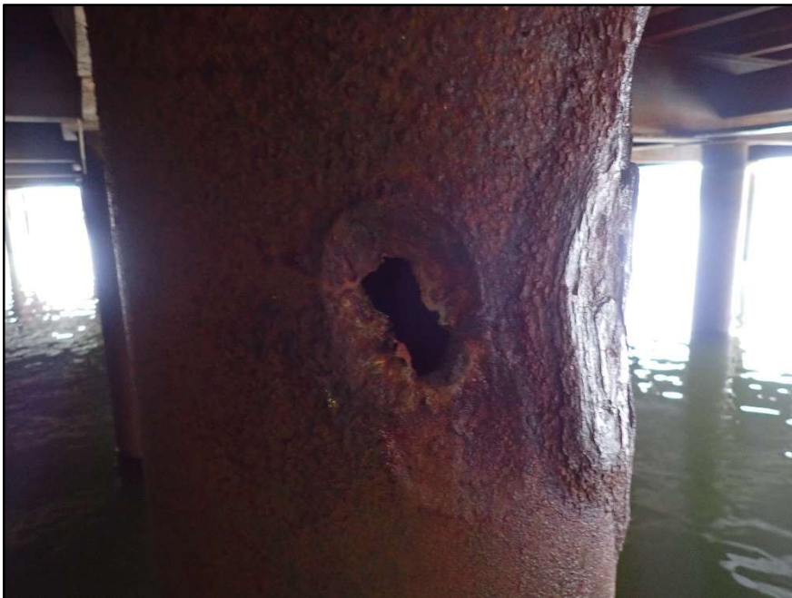
Photo 14 : Hole in steel, Bent 10 Pile E, looking north.
