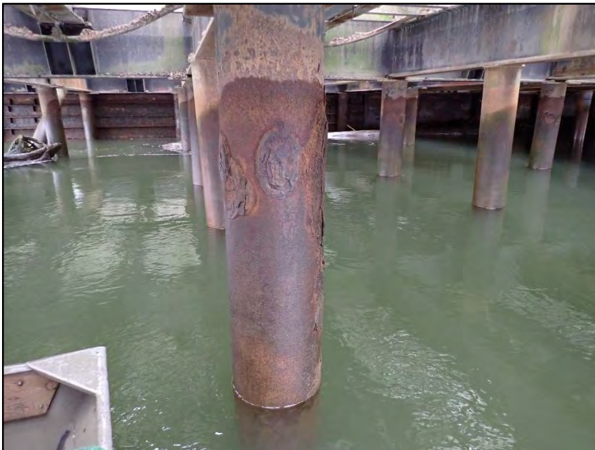
Photo 10 : Typical rust delamination, Bent 3 Pile C, looking west.
