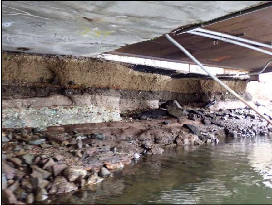
Photo 7 : Erosion under northerly wheelhouse extension, looking west.
