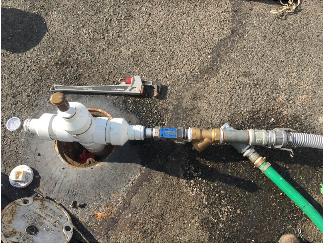
Photograph 3. Injection wellhead with pressure gauge and air release valve, with 2-inch flow totalizer to the right.
