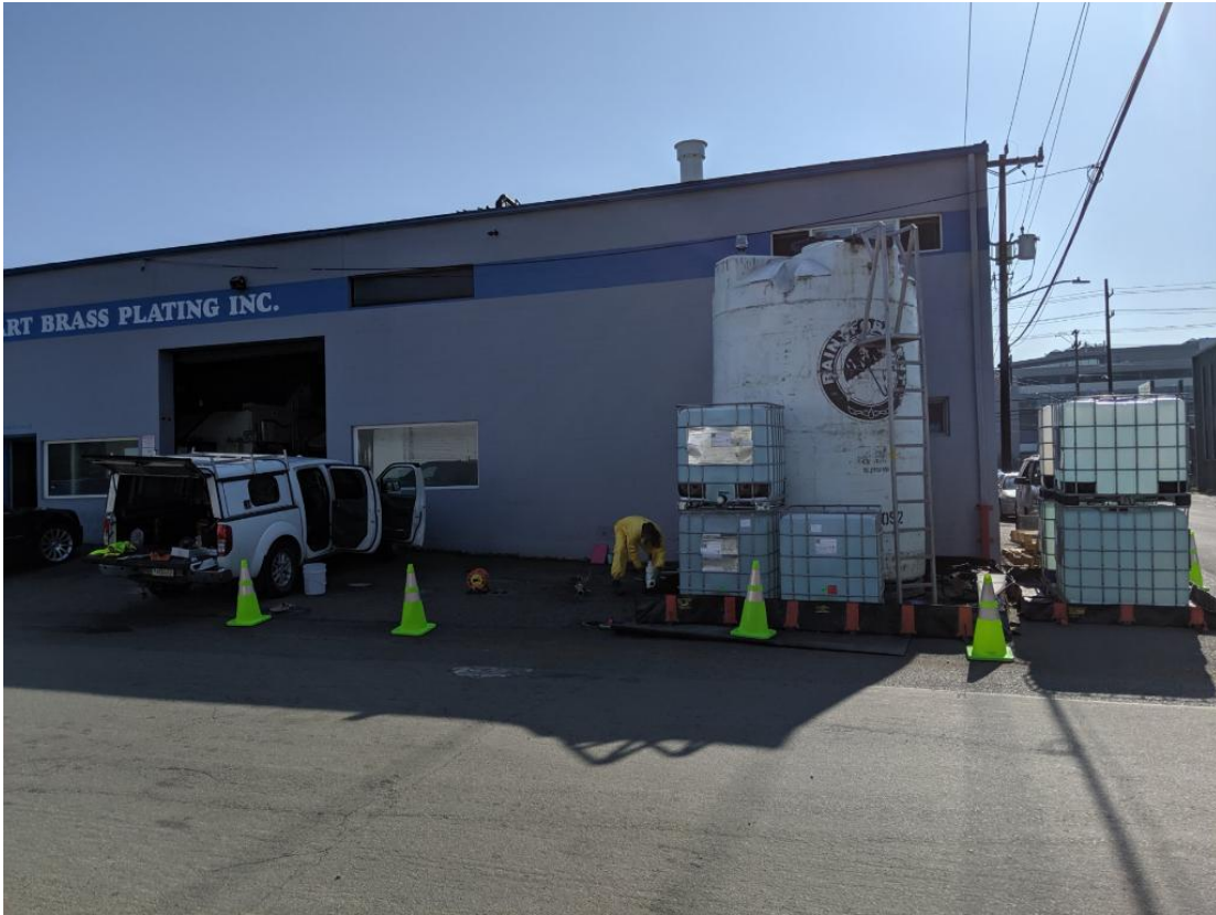
Photograph 1. Injection tank and reagent totes in front of Art Brass Plating.
