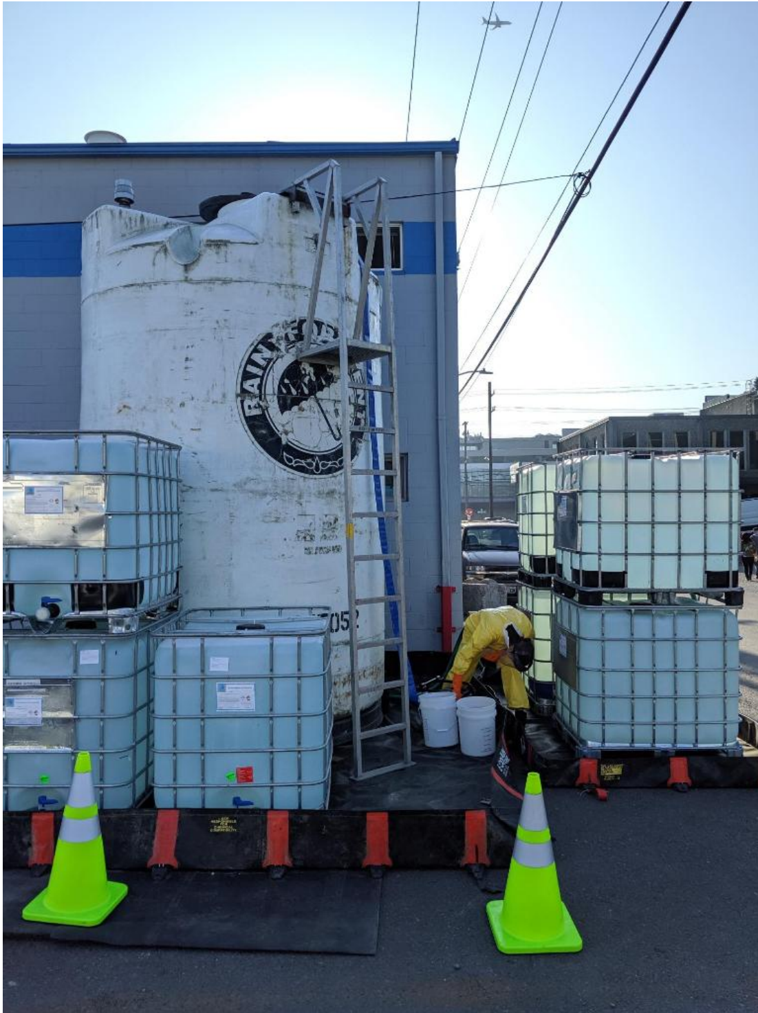
Photograph 2. Mixing a batch of injection-strength reagent from the concentrated reagent in the totes.
