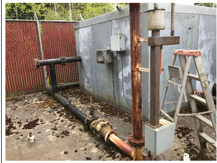
Flare facility overview
