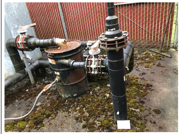
Flare Facility sampling port (lower right)
