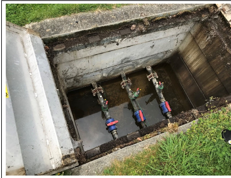
Typical subsurface manifold sampling ports on LFG control system
