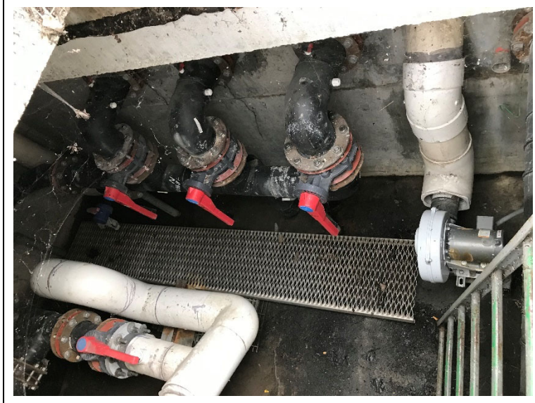
Vacuum system main underground manifold near bus station
