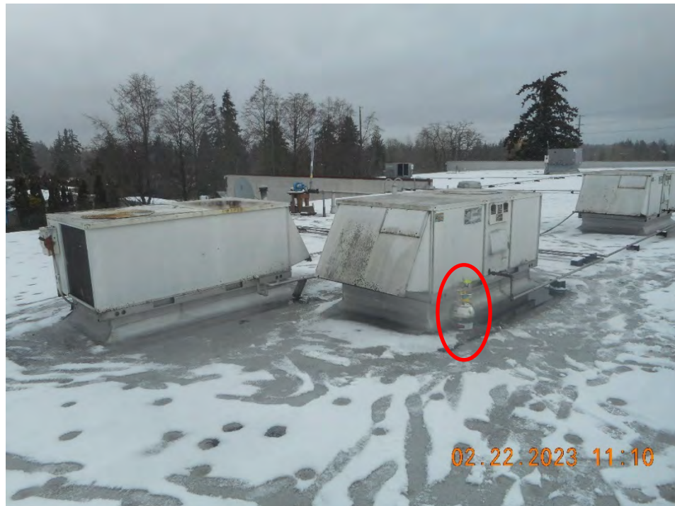
Photograph 2. Outdoor Air Sample OA-02 Placed on Building Roof, near Suite B-6 HVAC (February 22, 2023)
