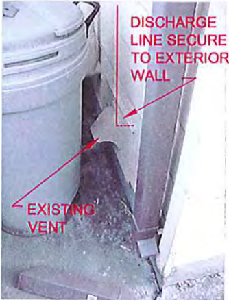
VIEW OF OUTSIDE VENT
