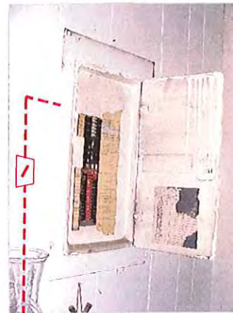
VIEW OF BREAKER PANEL
