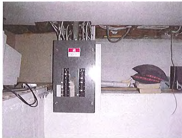
VIEW OF BREAKER PANEL
