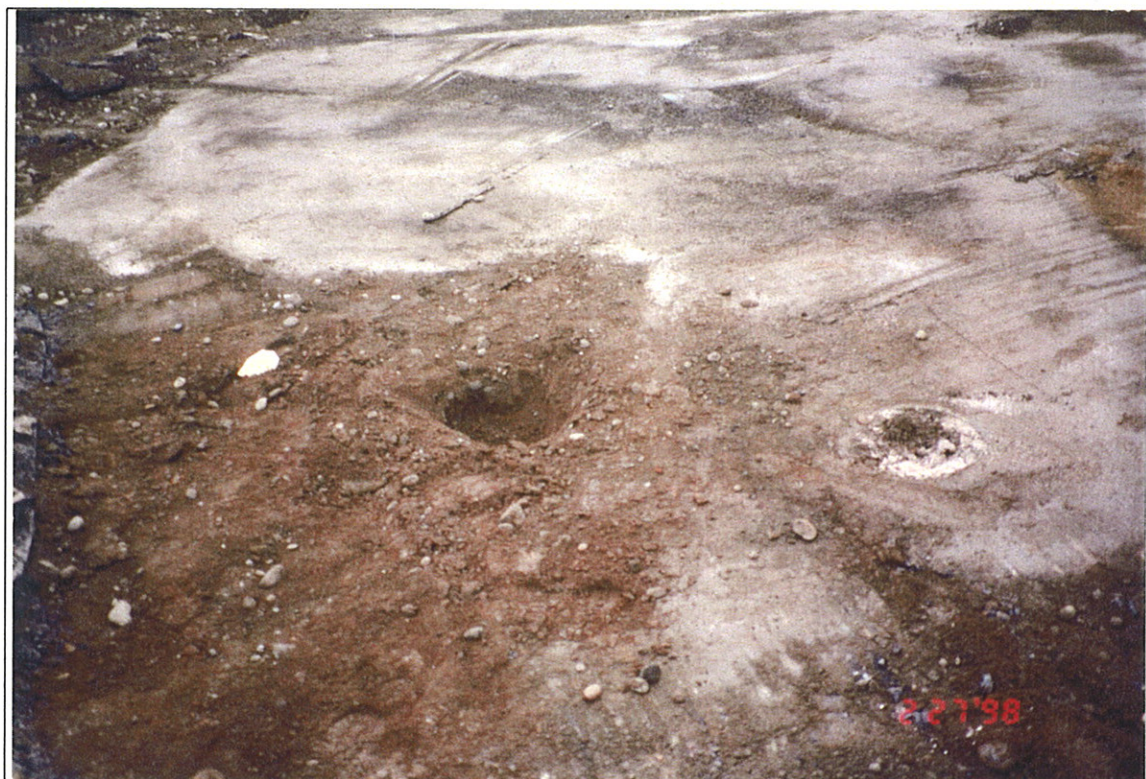
Photograph 2: Southwest corner of southern extension of SMC concrete floor slab, looking north.
