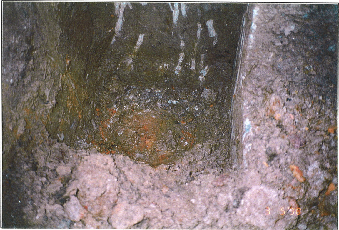
Photograph 23: Bottom of short leg of "L" shaped concrete vault showing circular depression in concrete.
