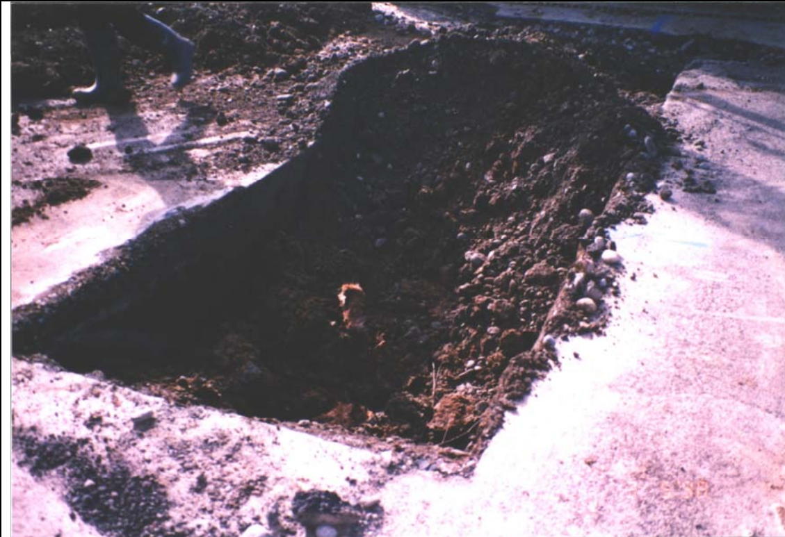
Photograph 15: Concrete pit in eastern part of the SMC concrete slab, looking south.
