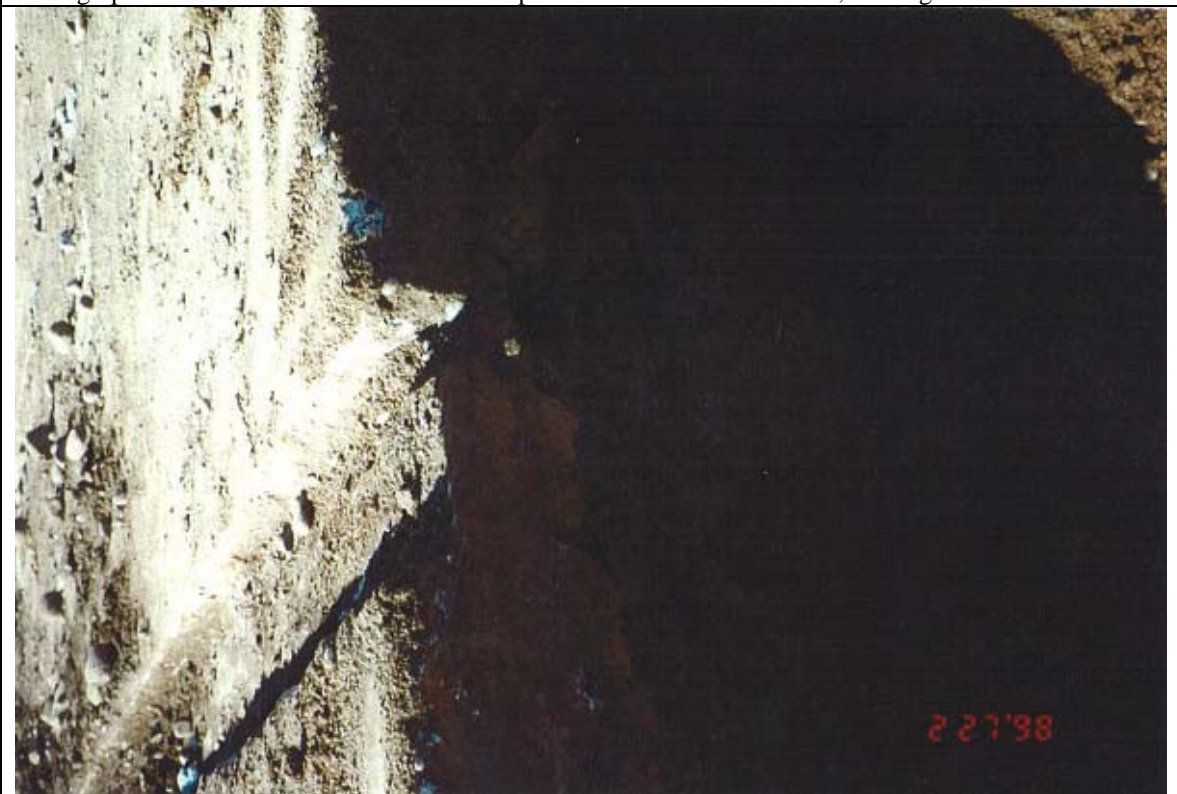
Photograph 6: Shallow groove or channel in southern extension of SMC concrete slab, looking west.
