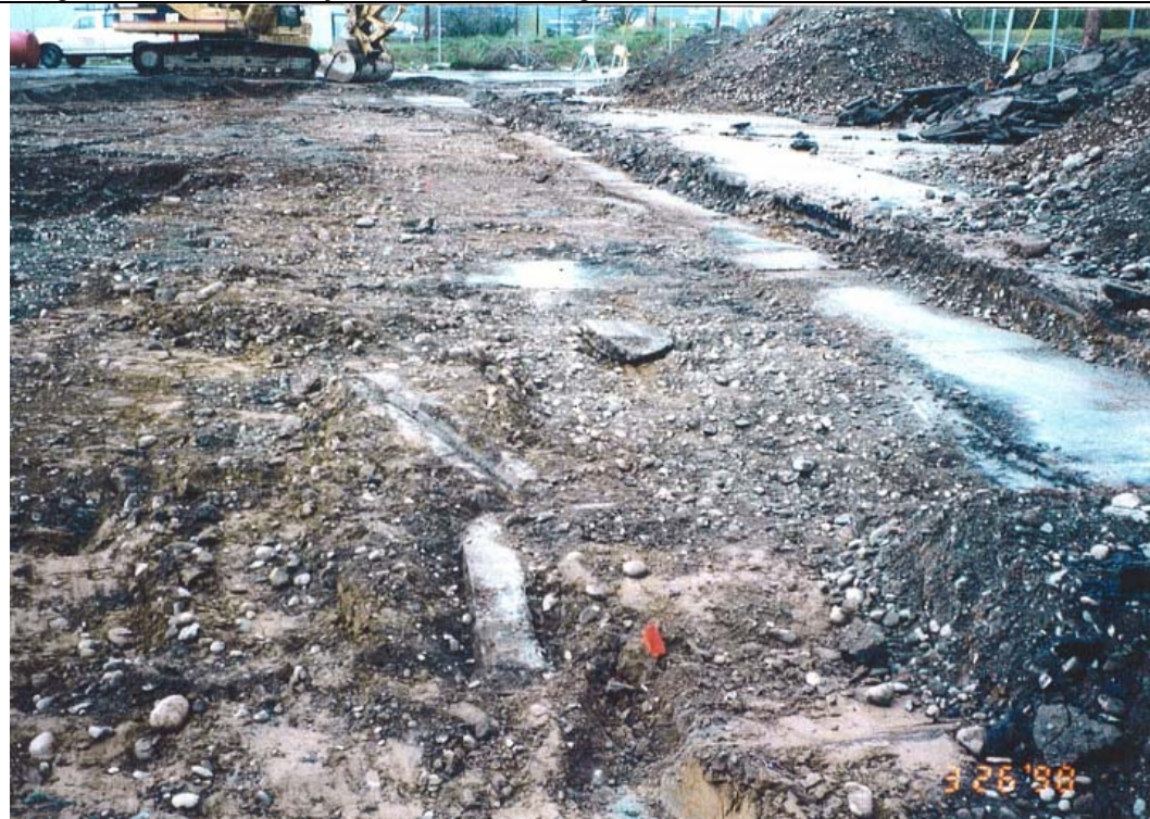
Photograph 28: View of the western portion of the SMC building where a concrete slab was not observed, looking west.
