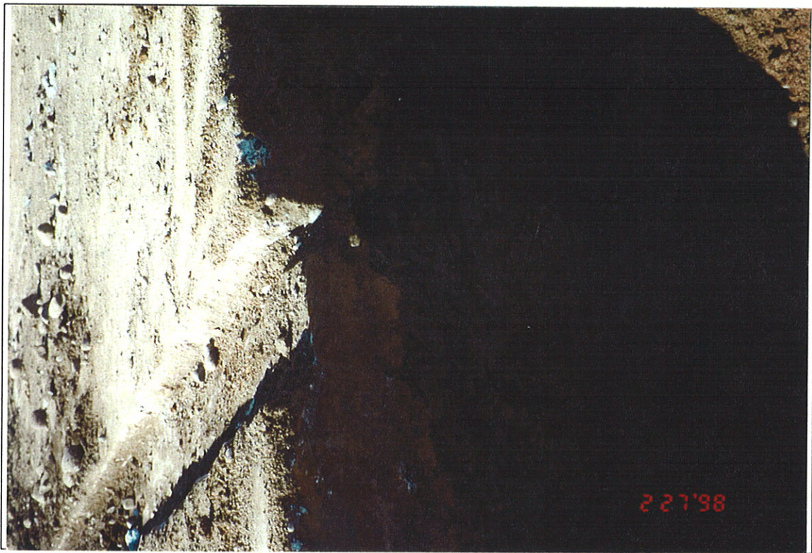
Photograph 6: Shallow groove or channel in southern extension of SMC concrete slab, looking west.
