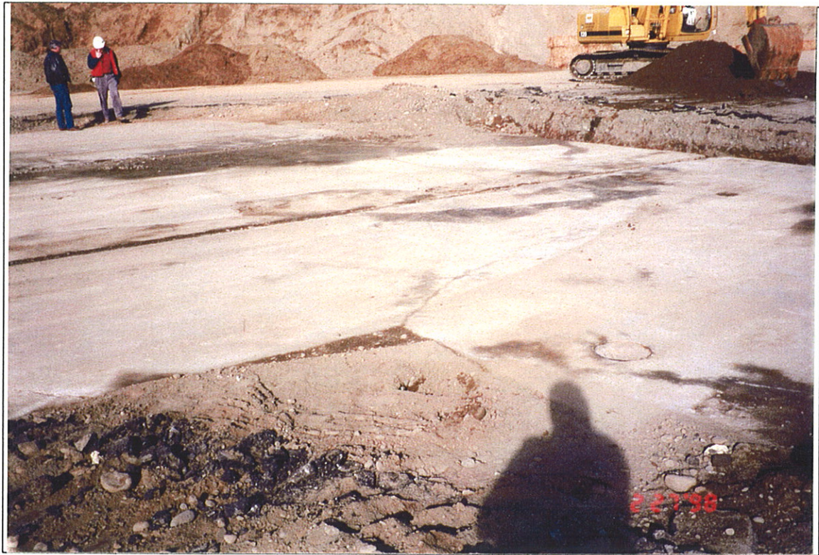
Photograph 3: Southern extension and central part of SMC concrete floor slab, looking northeast.
