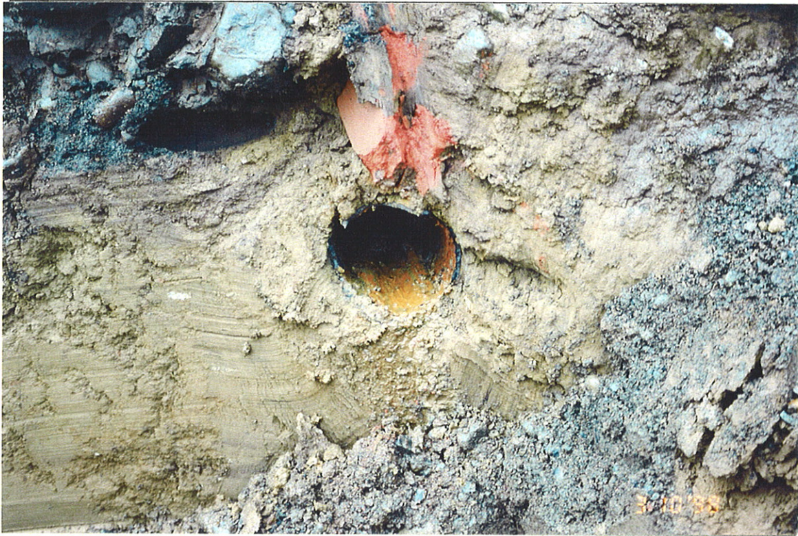
Photograph 30: Close-up of pipe in Photograph 29.
