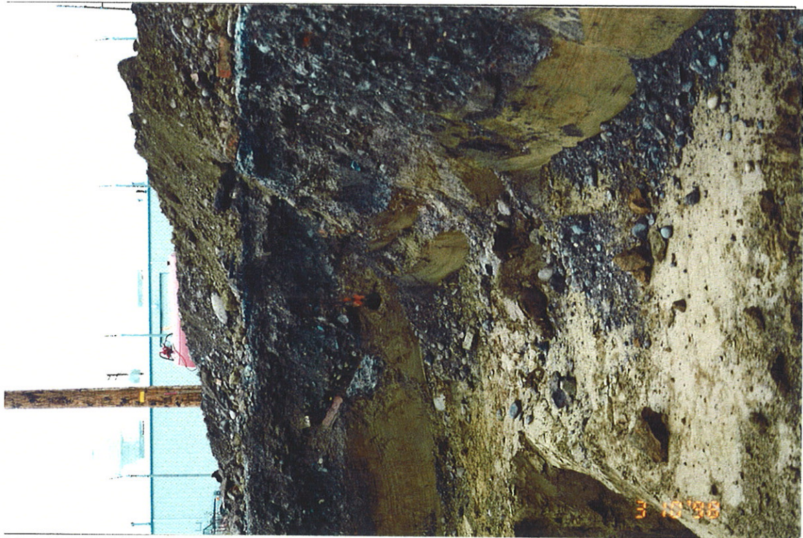
Photograph 29: Northwest corner of excavation which includes the southwest portion of the SMC building area. Notes pipe in corner of excavation.
