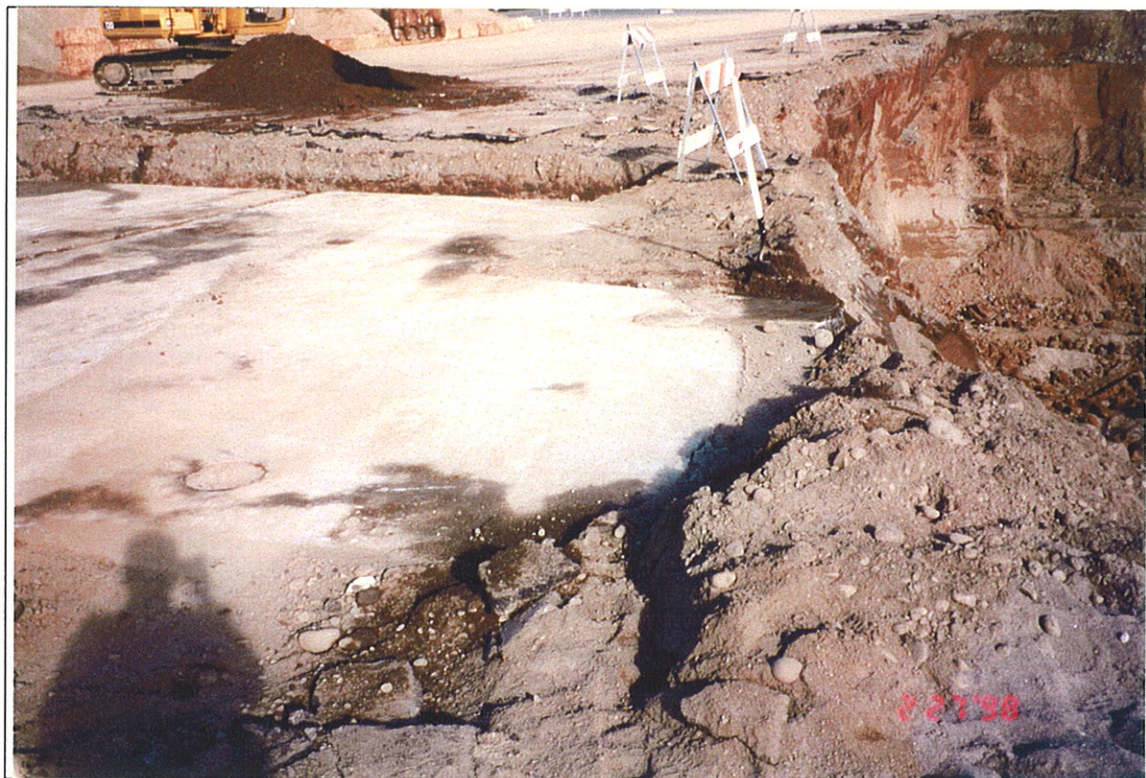
Photograph 1: Southern extension of Swan Manufacturing Co. (SMC) concrete floor slab, looking northeast.
