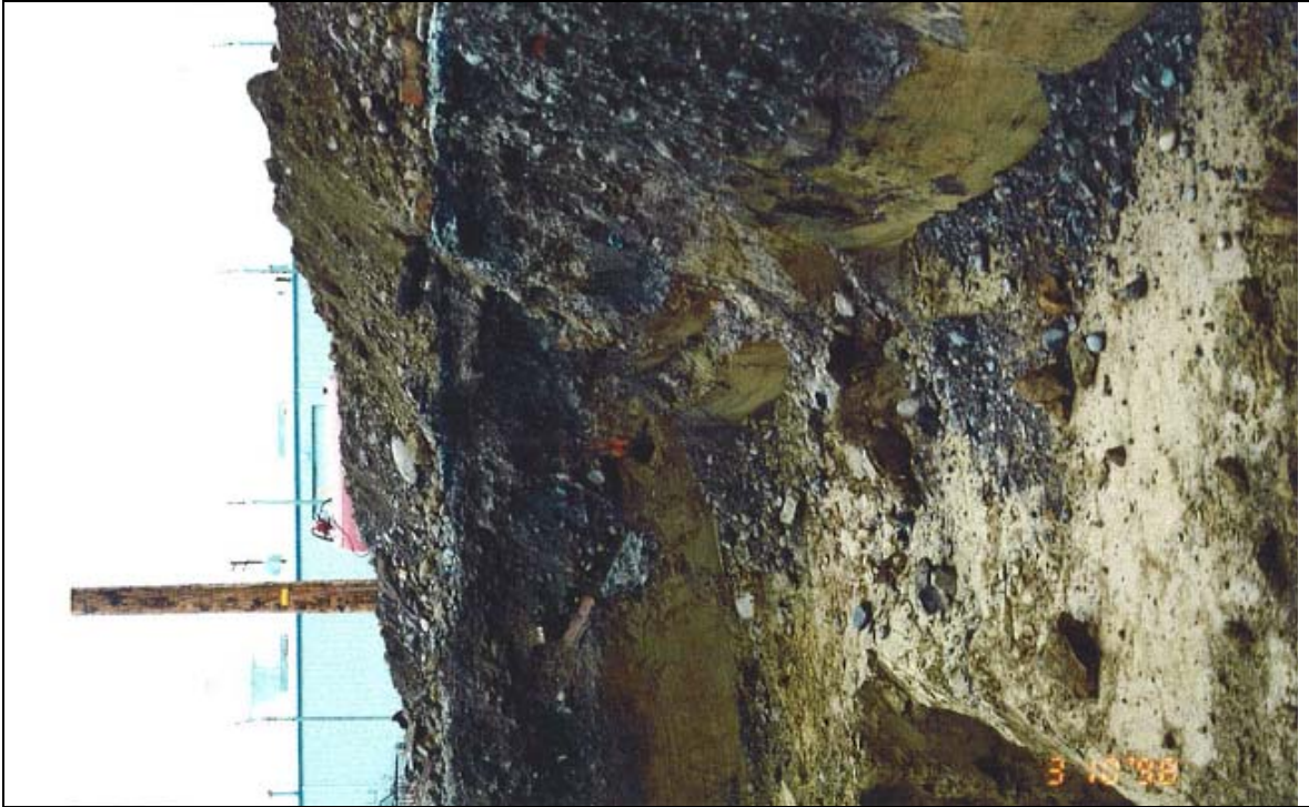
Photograph 29: Northwest corner of excavation which includes the southwest portion of the SMC building area. Note pipe in corner of excavation, looking west.
