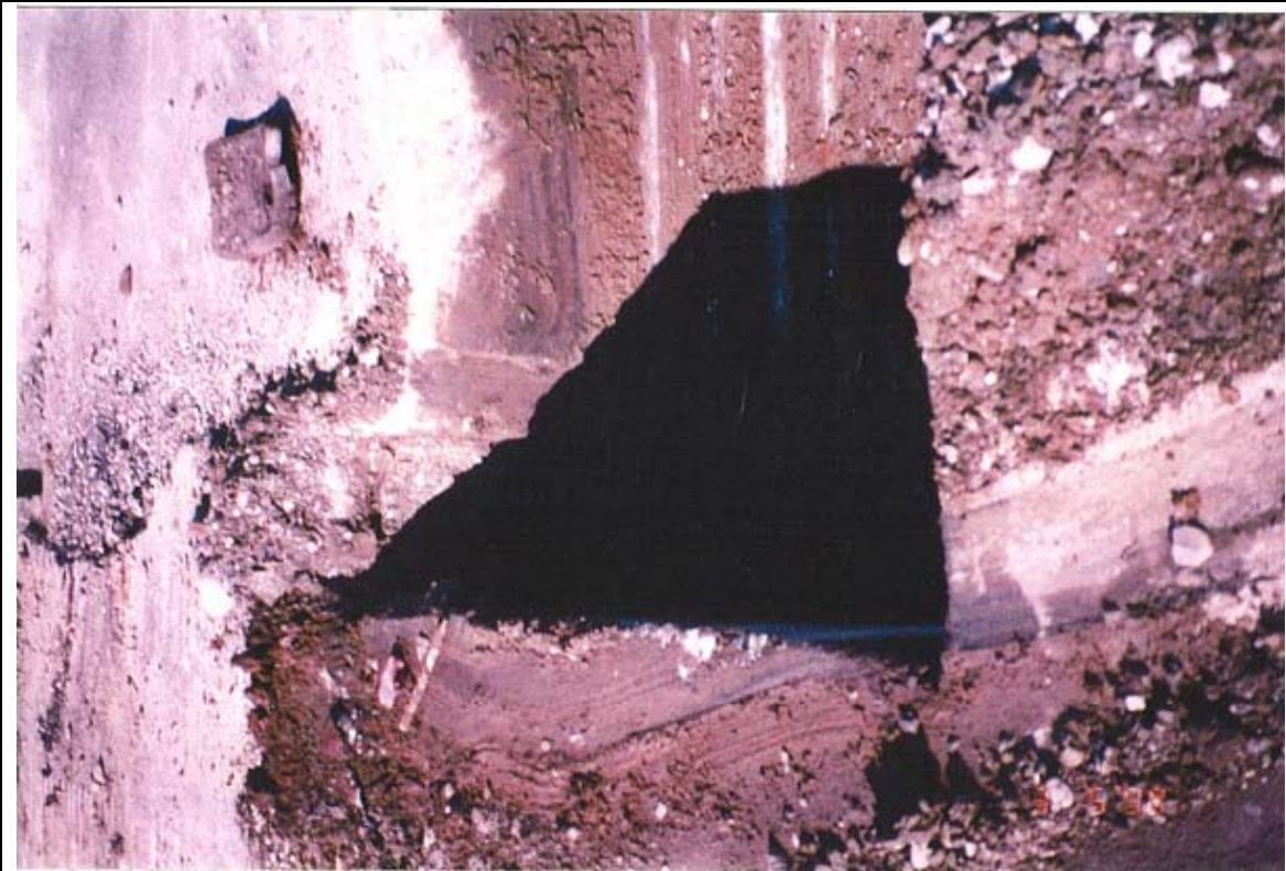
Photograph 18: Southern end of concrete pit. Photograph shows short "leg" of pit to the west of the large section of concrete pit.
