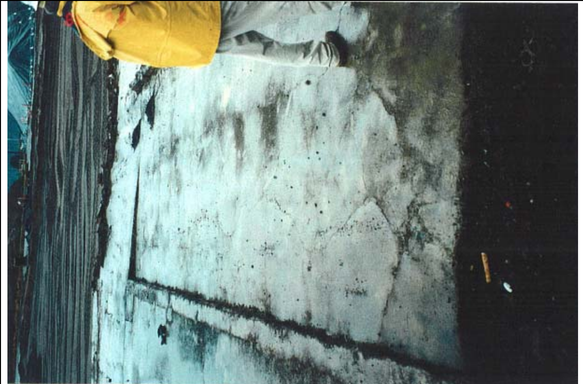
Photograph 27: Northern portion of SMC concrete slab showing concrete curb. Note ceramic cylinder in foreground found in soil adjacent to slab. Looking south.
