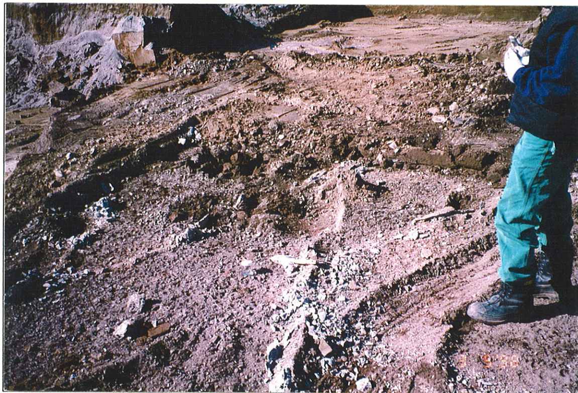
Photograph 8: Exposed soil under groove or channel after removal of concrete. Glass sample container shows location of sample MT.
