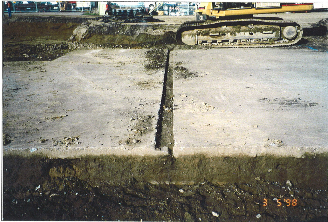
Photograph 7: Shallow groove or channel in southern extension of SMC concrete slab, looking west.
