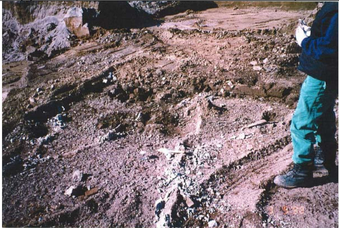
Photograph 8: Exposed soil under groove or channel after removal of concrete slab. Glass sample container shows location of sample Mid-trench.
