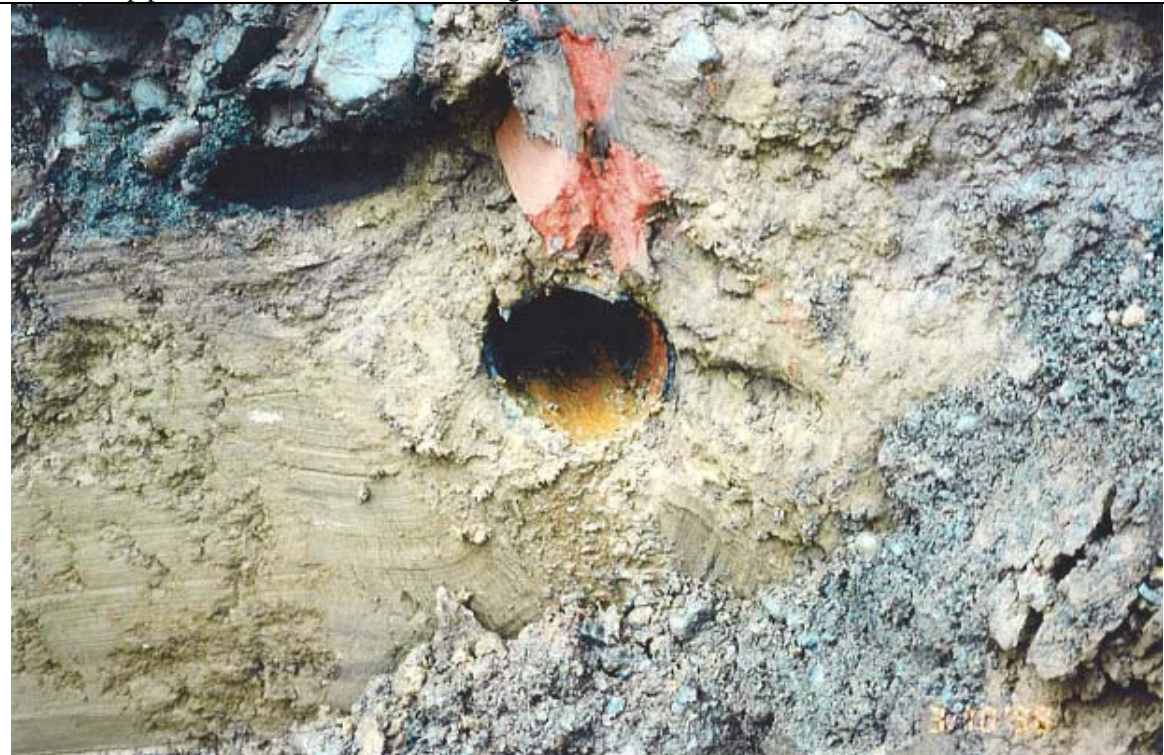
Photograph 30: Close-up of pipe in northwest corner of excavation observed in Photograph 29, looking west.
