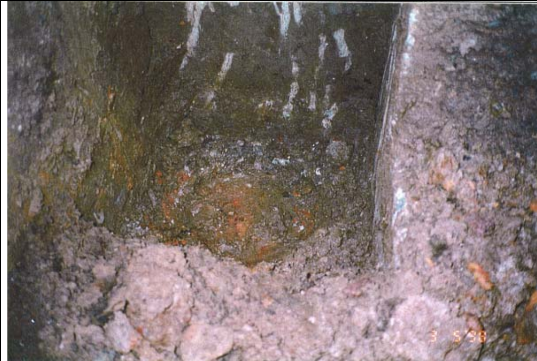
Photograph 23: Bottom of short leg of "L" shaped concrete pit showing circular depression in concrete.
