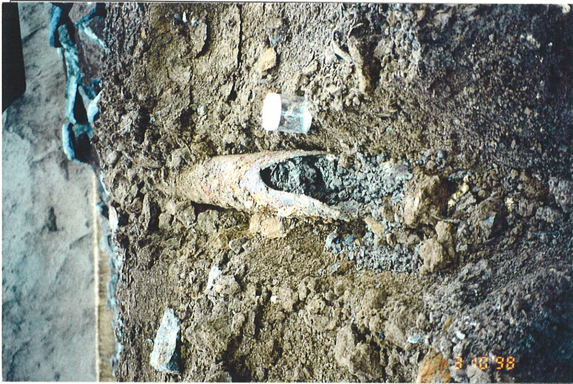
Photograph 31: Pipe under SMC concrete floor slab found approximately 10 feet east of the concrete vault. Note green gray material in pipe which was collected and labeled as CS-15.
