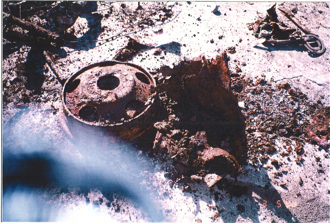
Photograph 19: Debris inside the concrete vault/pit.
