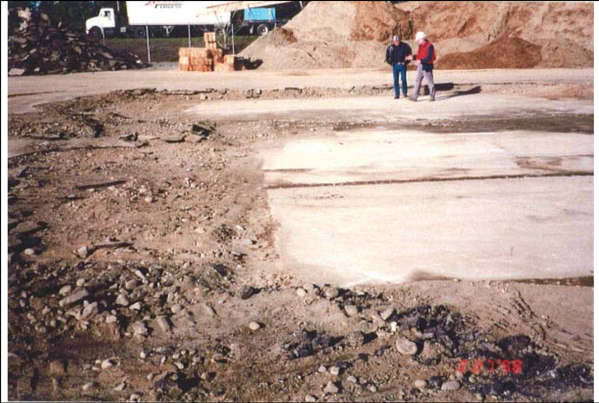
Photograph 5: Southern extension and western part of the SMC concrete slab, looking north.
