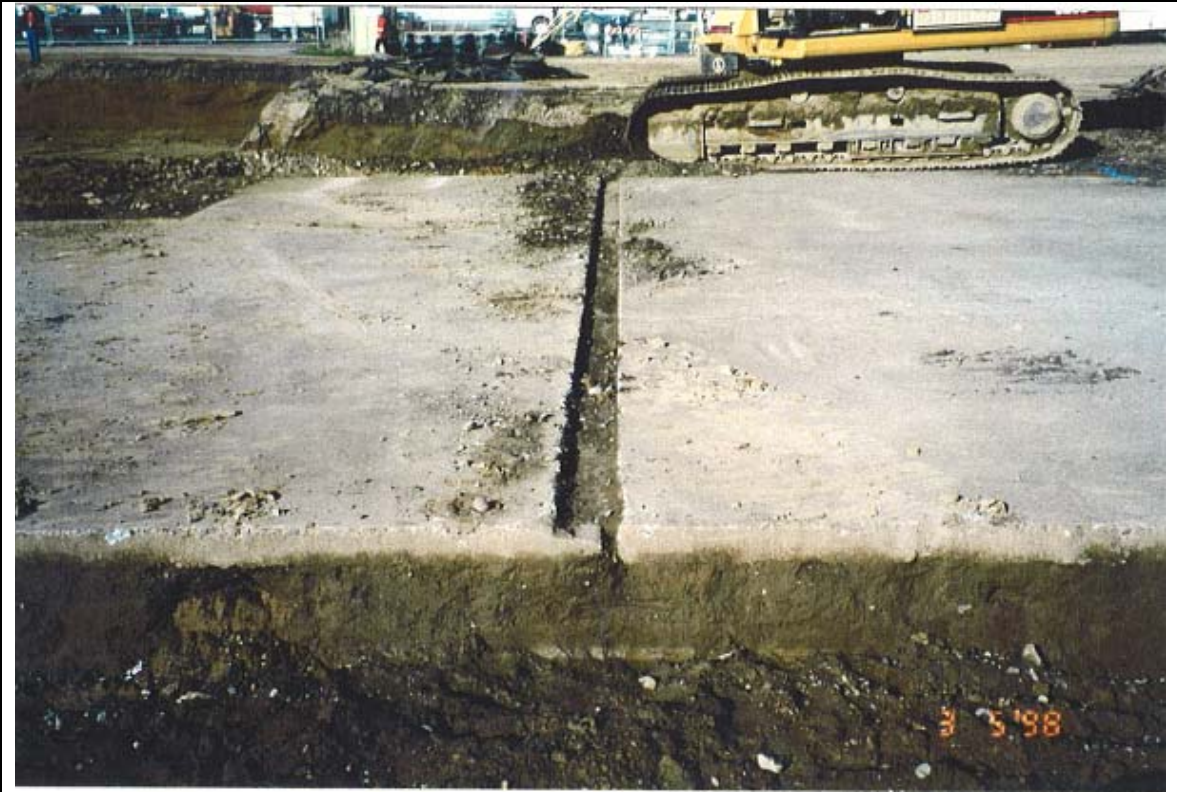
Photograph 7: Shallow groove or channel in southern extension of SMC concrete slab, looking west.
