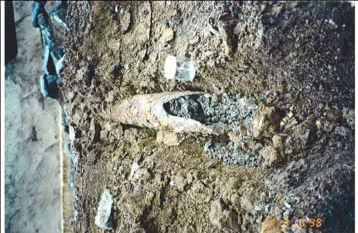
Photograph 31: Pipe under SMC concrete slab found approximately 10 feet east of the concrete pit. Note green gray material in pipe which was collected and designated CS-15.
