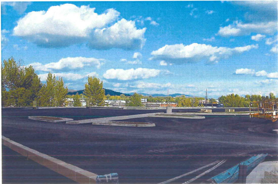
Photograph 22 – View to east of eastern property imported fill, storm water management, asphalt parking, and landscape improvements.
