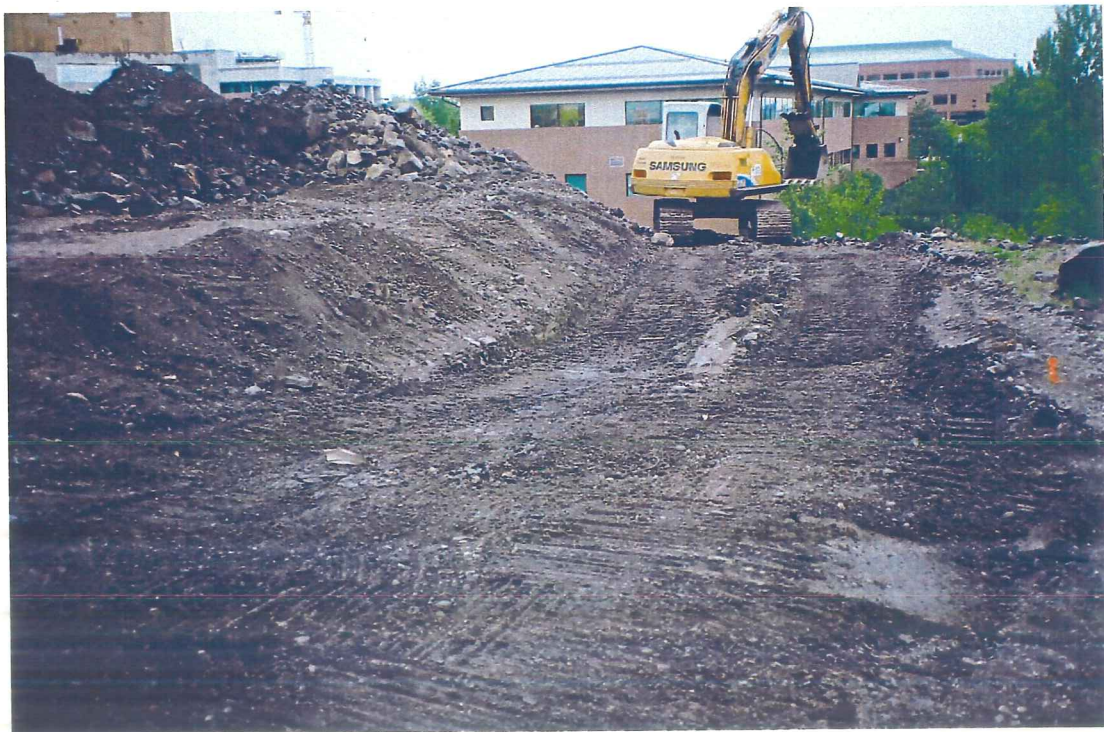
Photograph 16 – View to west of the riverside pedestrian walkway and waste storage, prior to screening operations.
