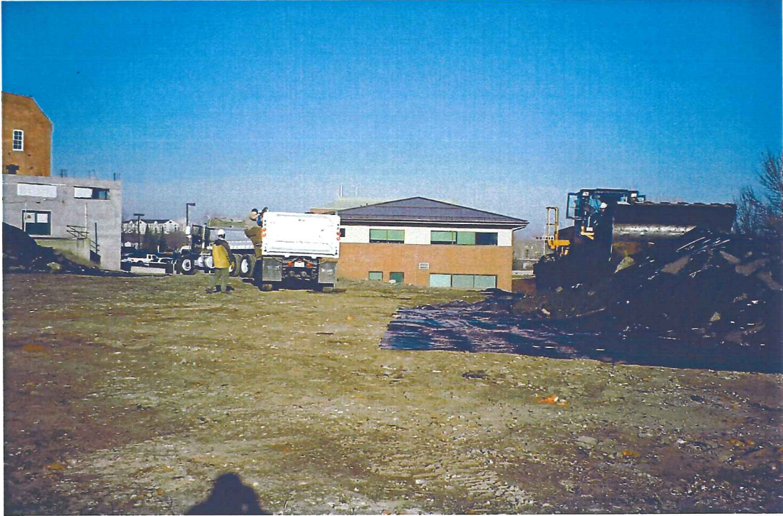
Photograph 13 – View of truck loading operations for waste soil material for transport to Greater Wenatchee Landfill.
