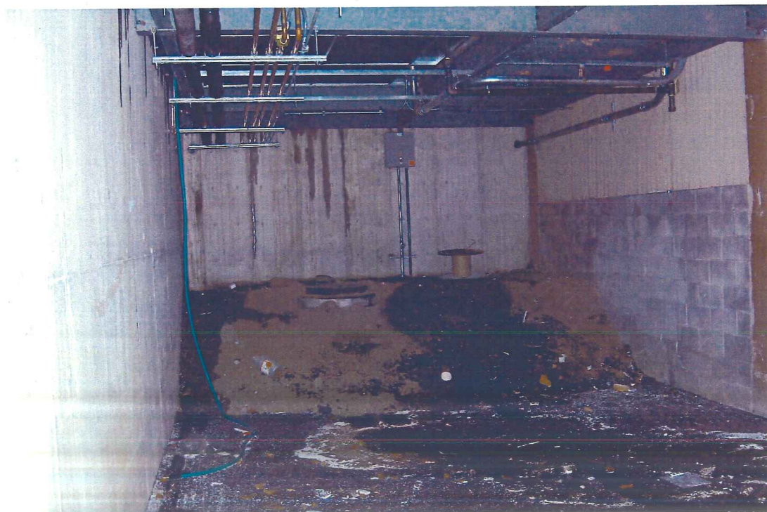
Photograph 30 – View of storm water collection sump and pump at east side of north alley.
