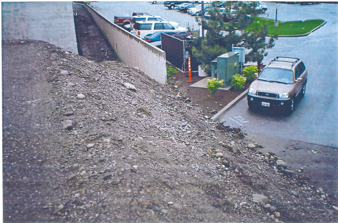
Photograph 18 – View of fill material along north central property line at north alley, prior to construction of storm water bio-filtration terrace.
