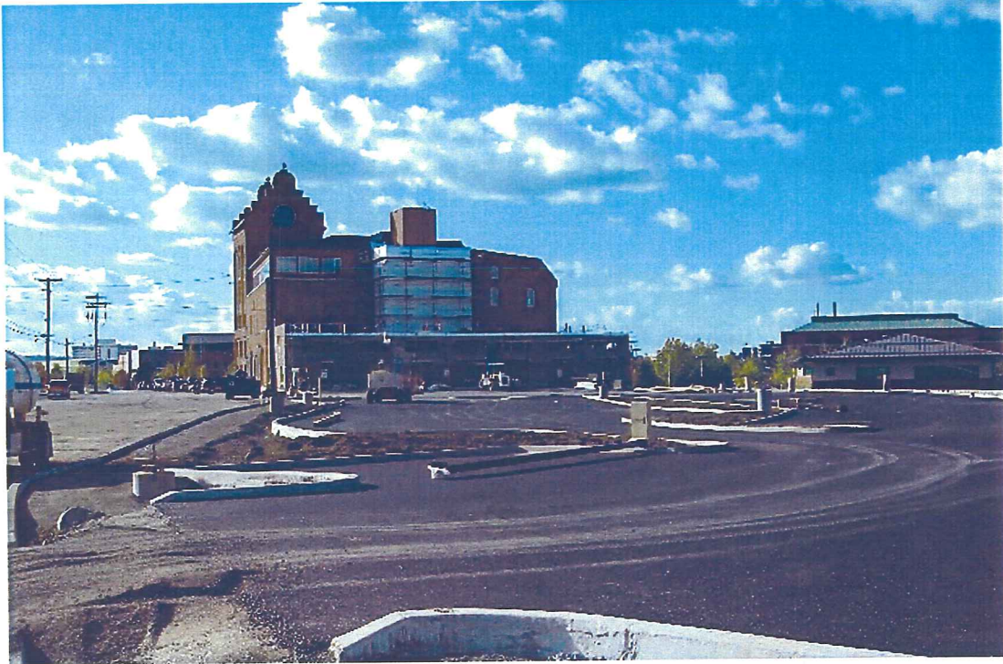
Photograph 21 - View to west of eastern property imported fill, storm water management, asphalt parking, and landscape improvements.
