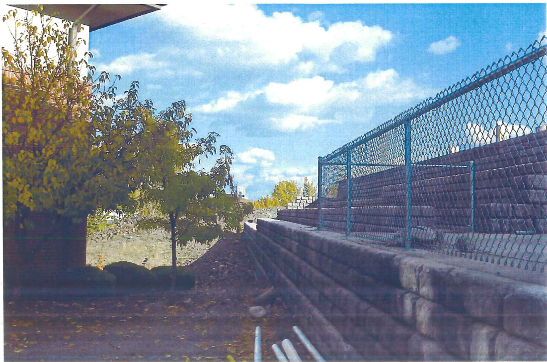
Photograph 20 – View to east of storm water bio-filtration terrace along north central property line.
