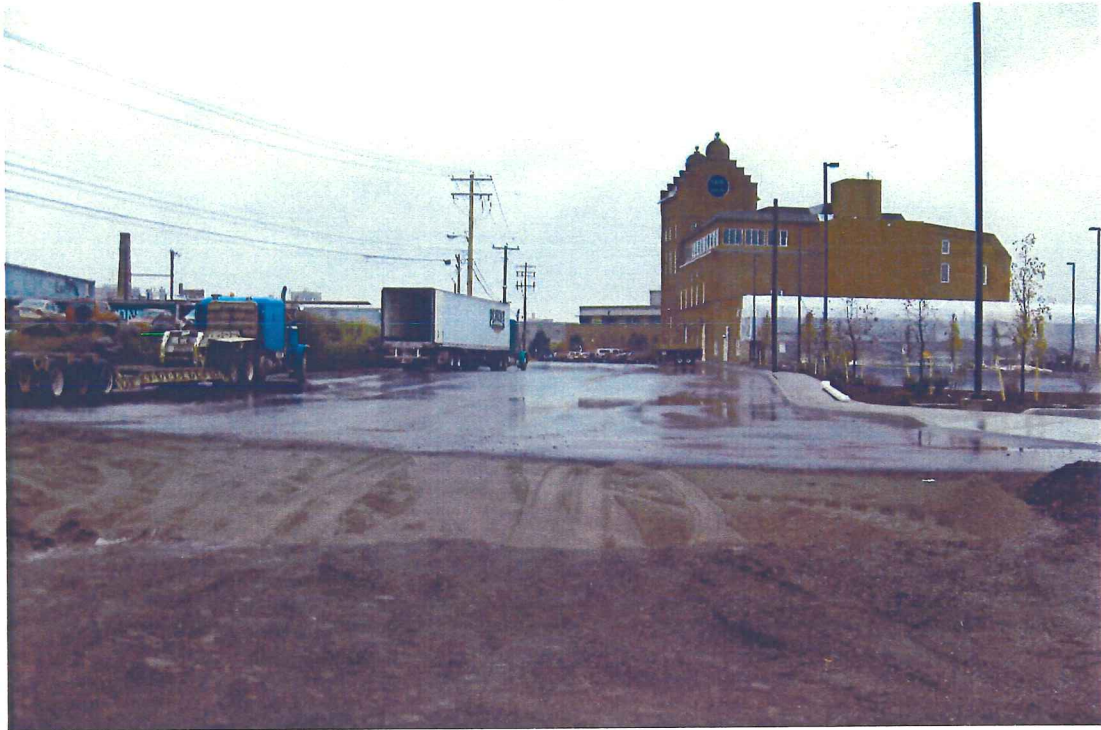
Photograph 27 – View to west of Front Street imported fill and asphalt improvements along the south side of the Schade Brewery.
