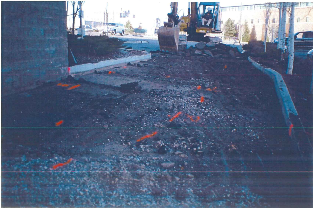
Photograph 2 – View to west of WNA remedial excavation area with utility markings (pre-remedial).
