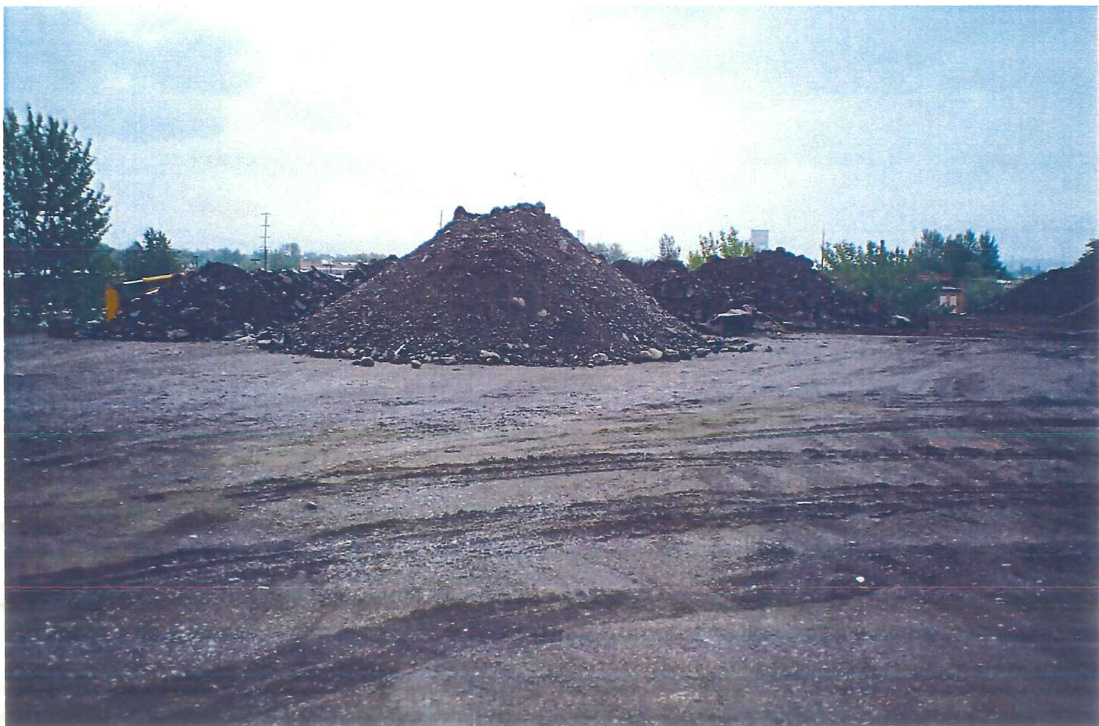
Photograph 14 – View of temporary waste storage during excavation of pedestrian walkway along Spokane River on north side of Site, prior to screening operations.
