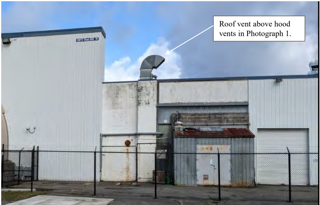
Photograph 2. C-1 Building roof vents above the equipment workshop area. Small metal shed attached to building also pictured.
