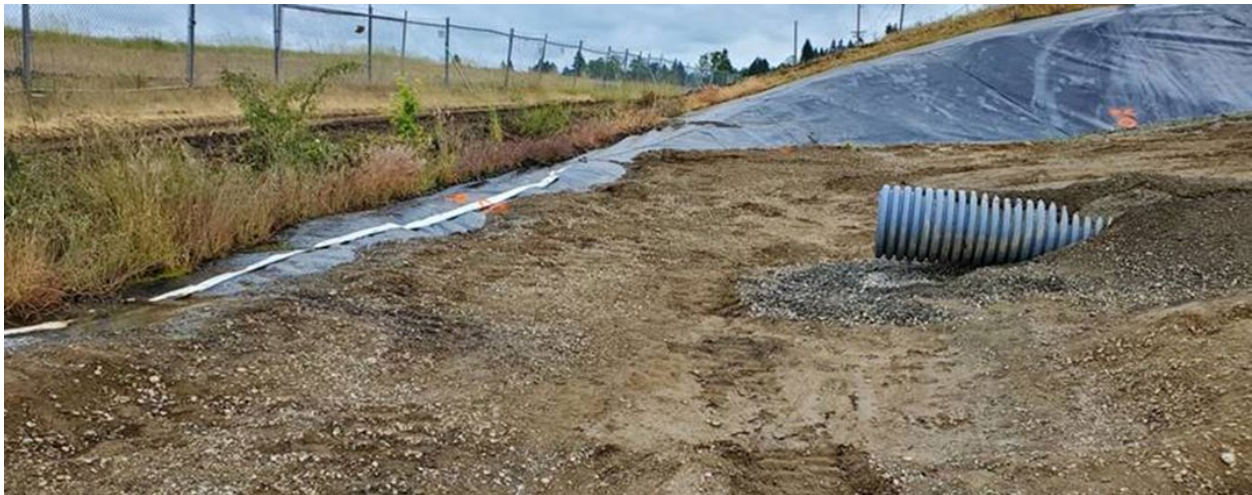
Photo 5 – Inlet to stormwater collection pipe will be about 12 inches above the surface that will receive the new geomembrane liner.
