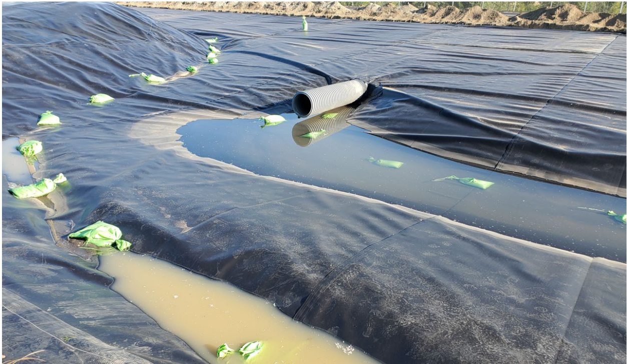
June 22 nd , 2023: Stormwater ponding on liner after weekend rains.
