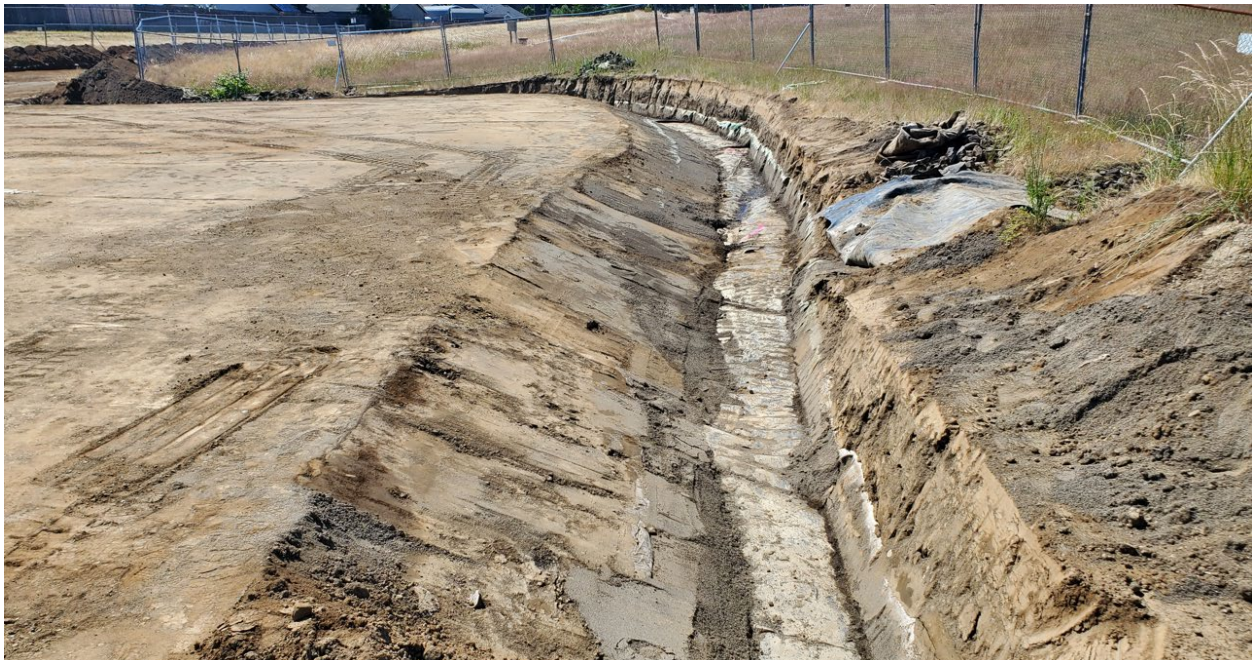
June 22 nd , 2023: Exposed existing Landfill cover liner in northeast corner of Landfill.
