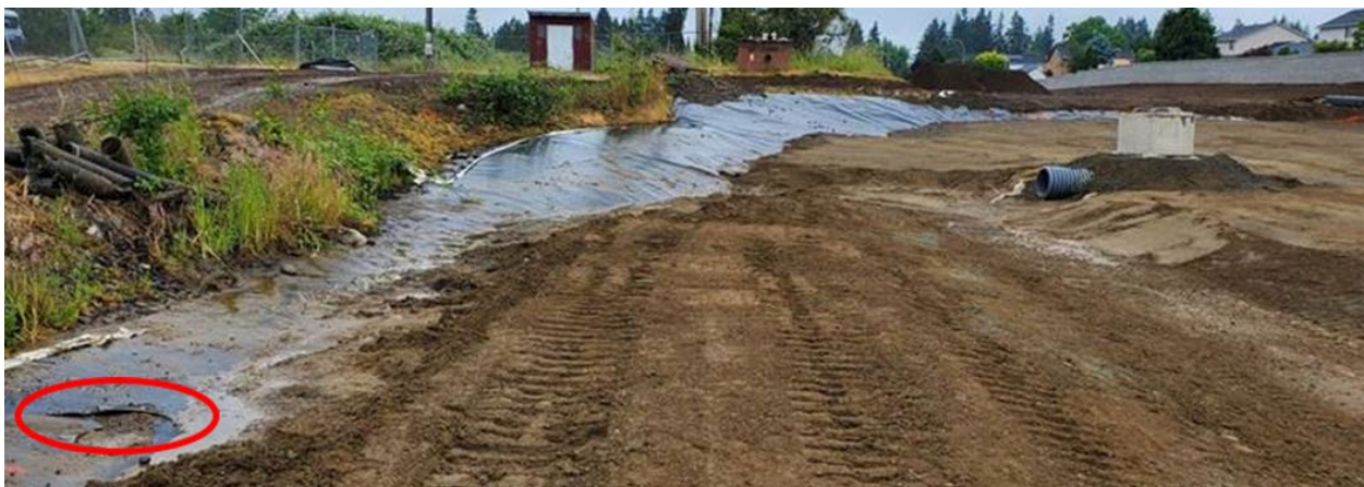
Photo 4 – Existing landfill liner with visible damage that needs to be repaired prior to installing new liner material.
