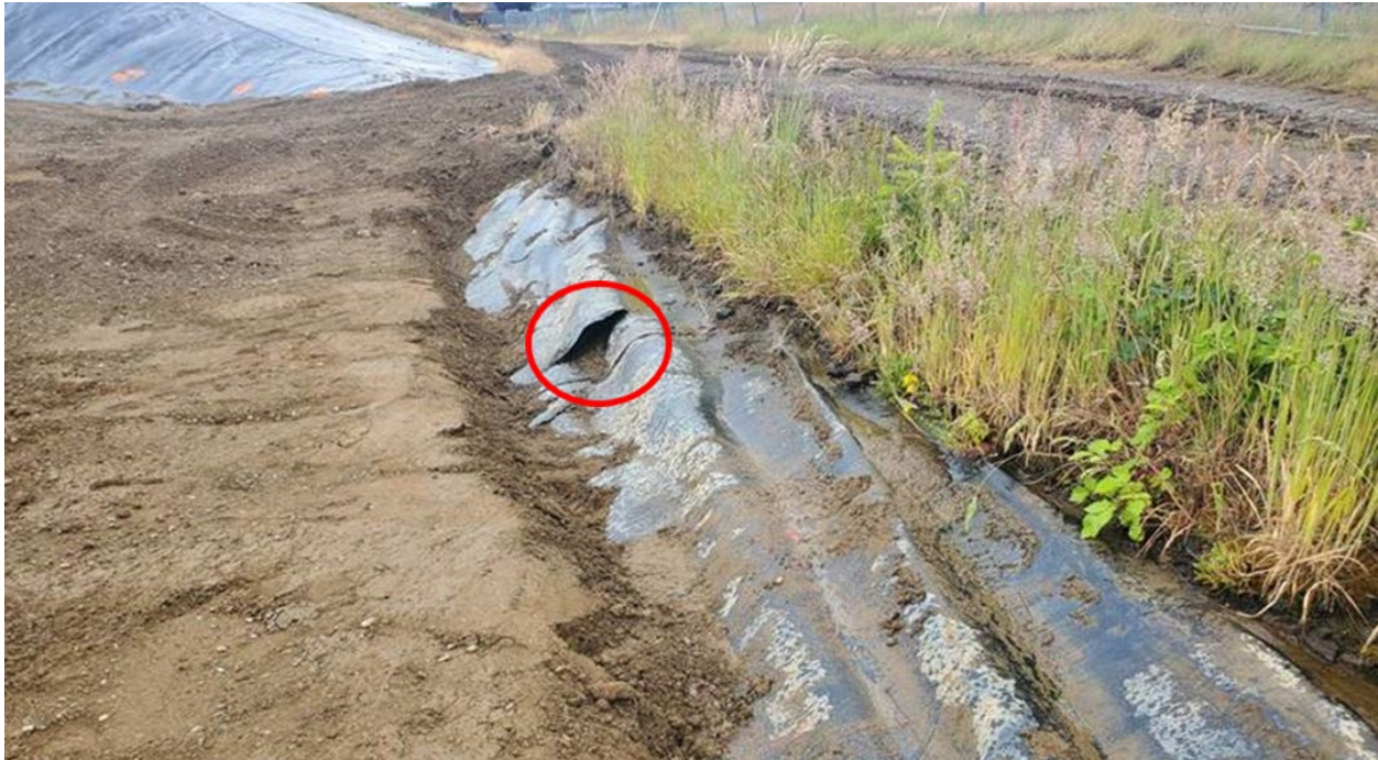
Photo 3 – Existing landfill liner with overlying soil that needs to be removed and visible damage that needs to be repaired prior to installing new liner material.
