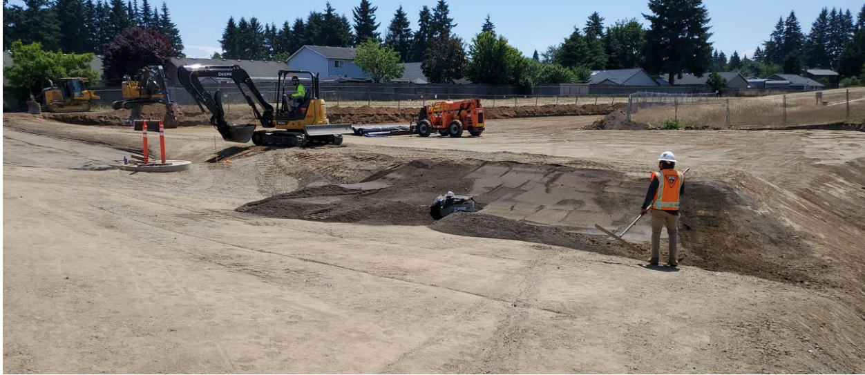
June 26 th , 2023: Preparation of subgrade for geomembrane deployment in northeast corner of Landfill.
