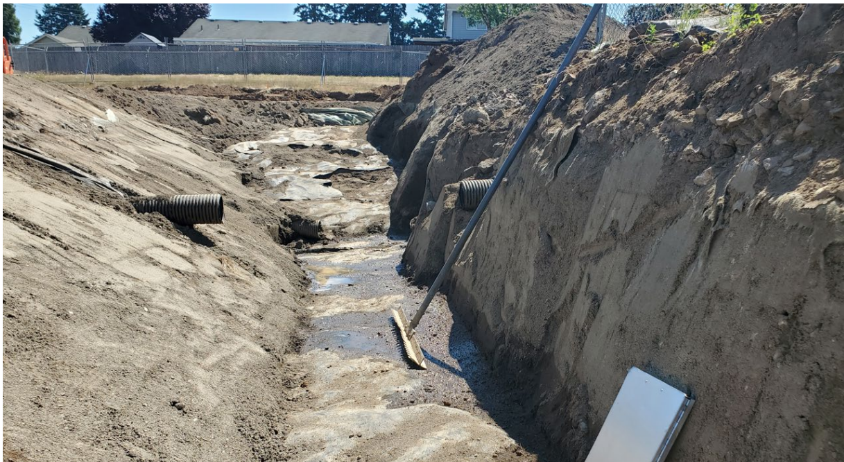
June 22 nd , 2023: Exposed corrugated plastic drain pipes above Landfill cover liner.
