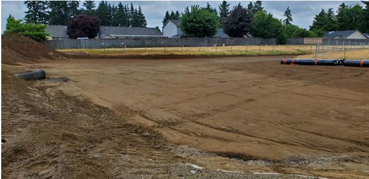
Photo 6 - Grading appears to be inadequate for surface water drainage into the stormwater collection pipes.
