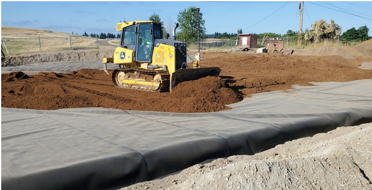
June 29 th , 2023: Spreading of cover layer soil, wrinkles in geomembrane being “walked” to anchor trench where extra material can be removed.
