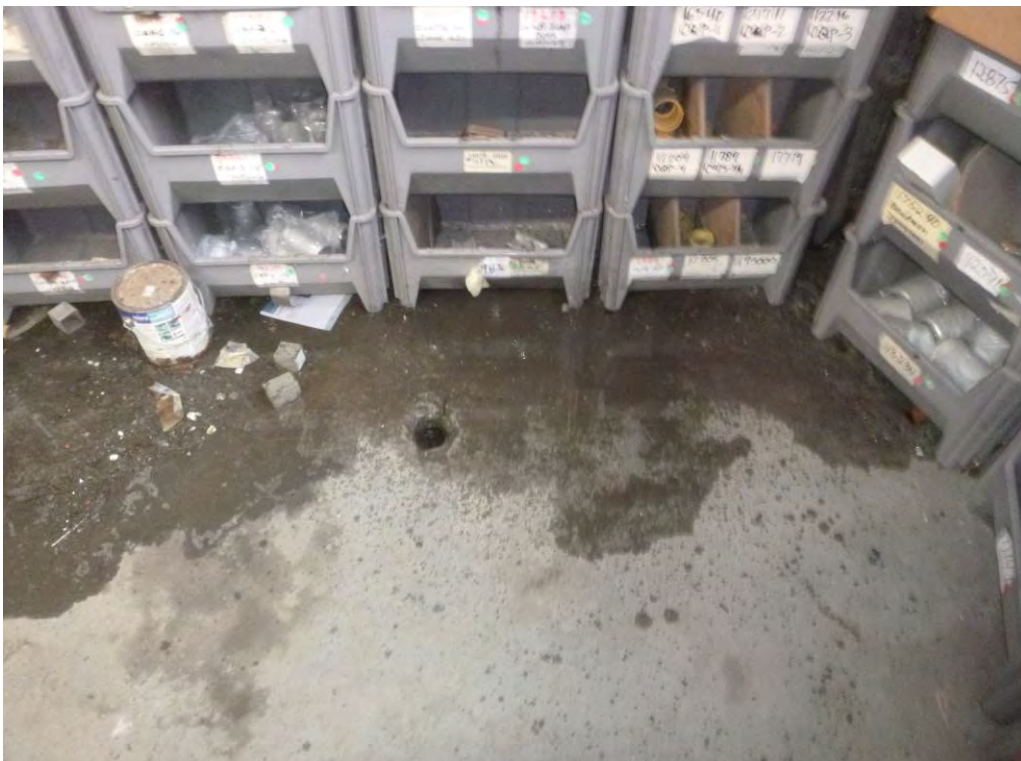
Photo 4: An approximately 6-inch uncovered hole located in the parts storage area in the northeast corner site building (rainwater from leaks in ceiling visible).
