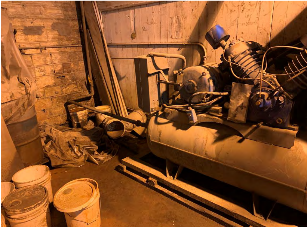
Photo 9: View of an air compressor in Bay 3 for warehouse operation. Signs of water intrusion (wet floor) and oil staining (approximately 20 square feet) around the air compressor.
