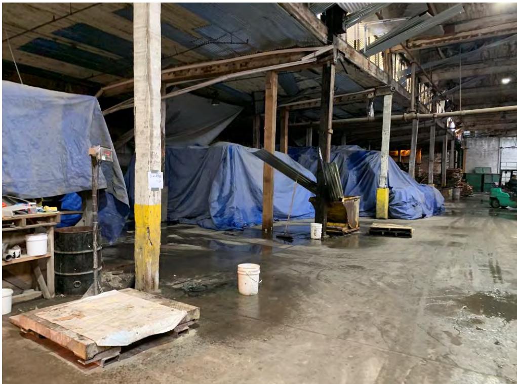
Photo 8: Storage of blast media (mostly repackaged slags) covered under blue tarps (rainwater from leaks in ceiling visible).
