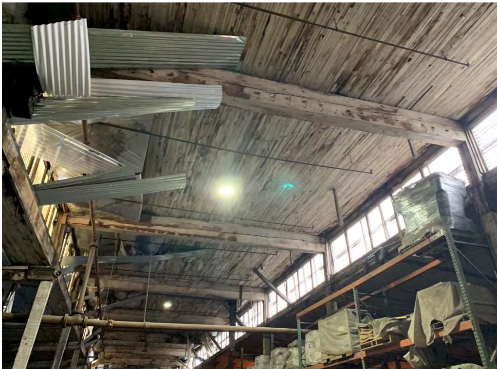
Photo 10: Ceiling of the site building (aluminum sheets used to divert water through upper windows).
